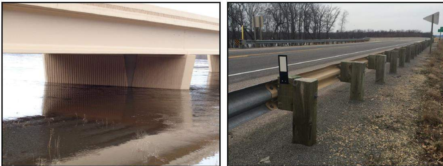
Figure 23. Examples of Treatments Used On B-56-181, US 14 over Wisconsin River, Spring Green
