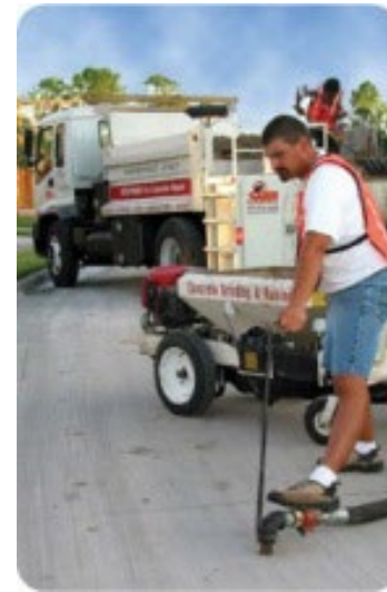
Class 912 Miscellaneous Equipment Mudjack
