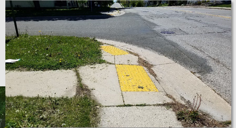
Example of non-compliant curb ramp on WIS 92
