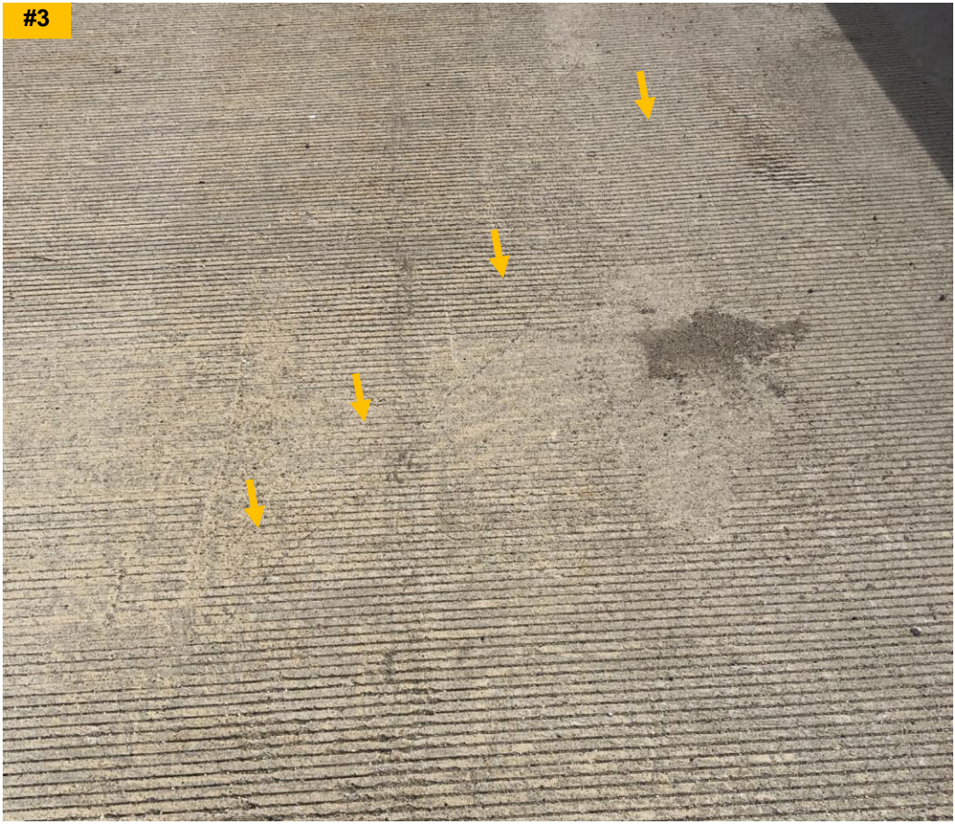
Figure A-17: IL 390 over Mittel Dr – Observed Cracking Photos
