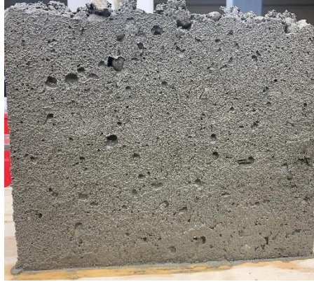
Figure 5-1: Mixture BD-C-036 overall surface voids visual rating; 2 which is equivalent a surface void value of 10-30%
