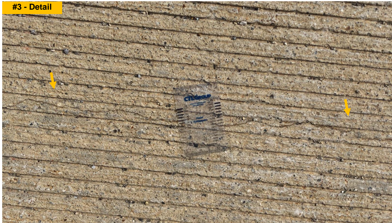
Figure A-19: IL 390 over Lively Blvd – Observed Cracking Photos
