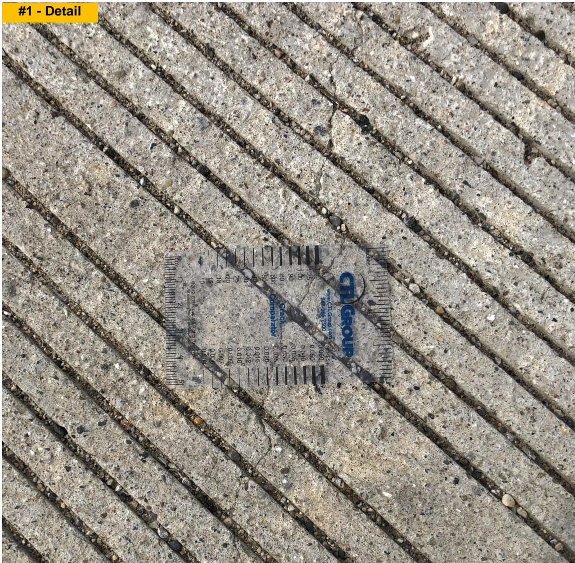
Figure A-13: IL 390 over N Prospect Ave – Observed Cracking Photos
