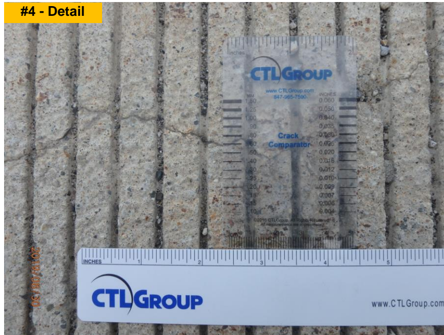
Figure A-11: IL 390 over N Arlington Heights Rd – Observed Cracking Photos
