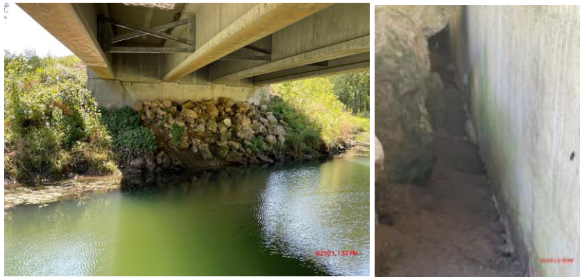
Photos of an abutment and a close-up of erosion along the abutment
