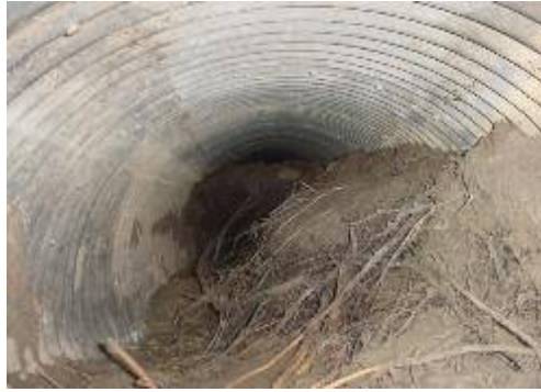
Figure 4-1 Example of Obstruction in Culvert (ASCE, 2008).
