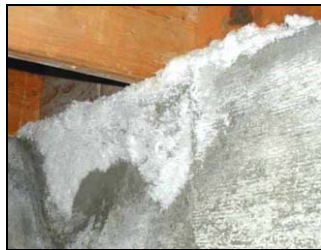
Figure 2-9 Formation of Efflorescence on a Concrete Surface.
