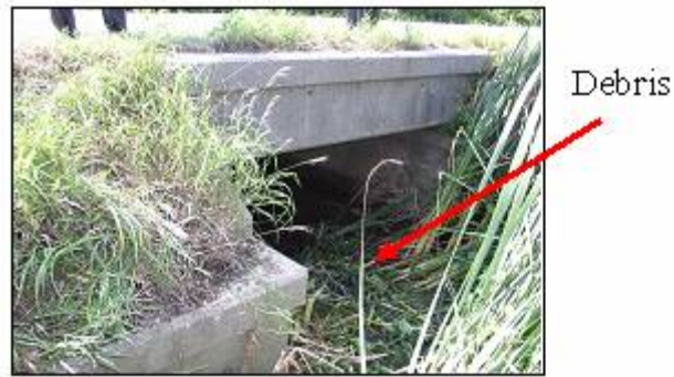
Figure 2-12 Debris at the Opening of the Culvert
