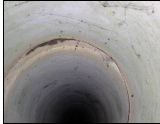
Figure 2-5 Transverse Cracks in a Culvert Pipe
