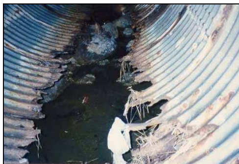
Figure 2-2 Deterioration due to Abrasion (Caltrans, 2003)
