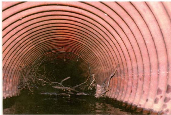
Figure 2-13 Beaver dam inside a culvert. (Paternaude, R., 2003).
