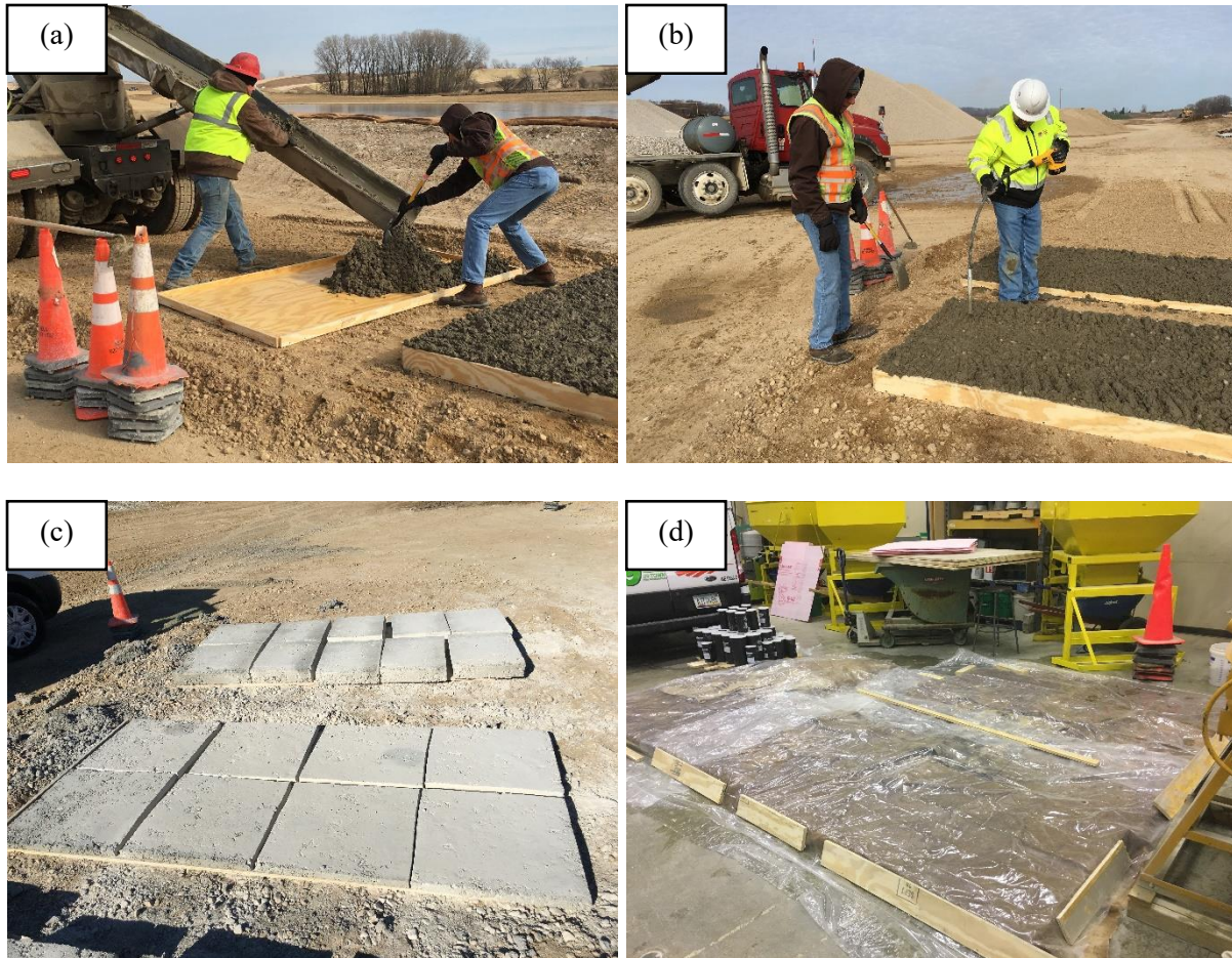
Figure 2.1 (a) Plant-mixed concrete was poured into 4’*8’ forms (b) consolidated and finished on site (c) sawcut into 2’*2’ panels after 48-hour on-site curing (d) panels were transported to the lab and burlap cured for 28 days.
