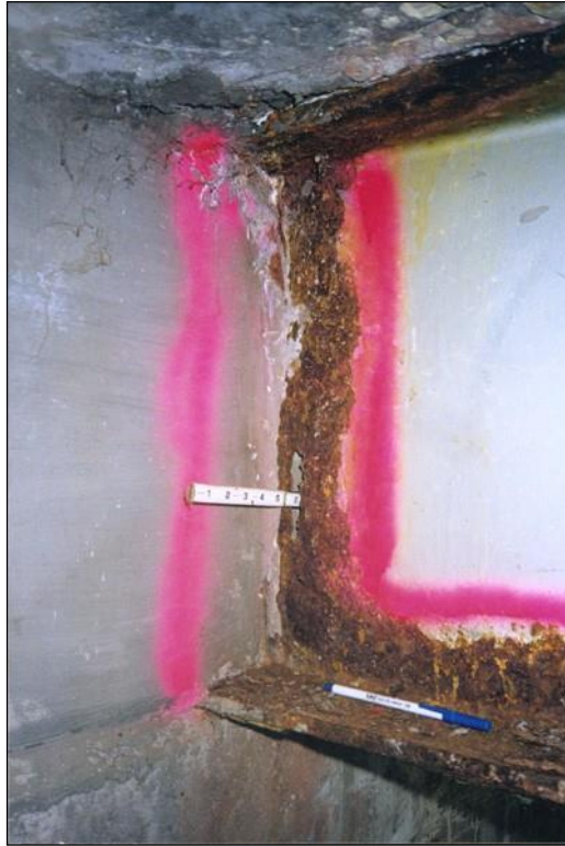
Figure 2.4.4.1-37: Through Thickness Section Loss of a Rolled Beam Web - Condition State 4.
