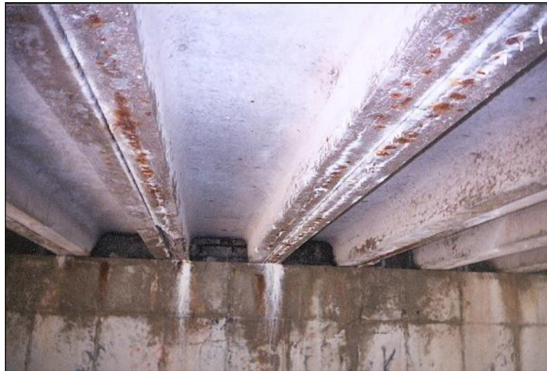
Figure 2.4.3-4: Deteriorated Prestressed Channel Beams.
