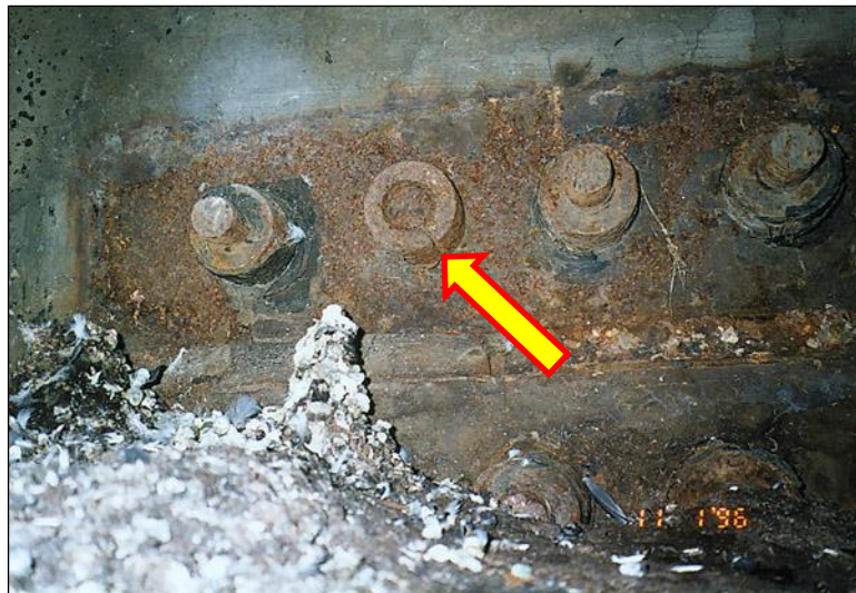
Figure 2.4.4.3-4: End of Post-Tensioning Rod with Cracked Nut – Connection Condition State 3.
