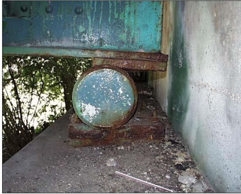
Figure 2.4.8.2-11: Critically Misaligned Roller Bearing – Alignment Condition State 3.
