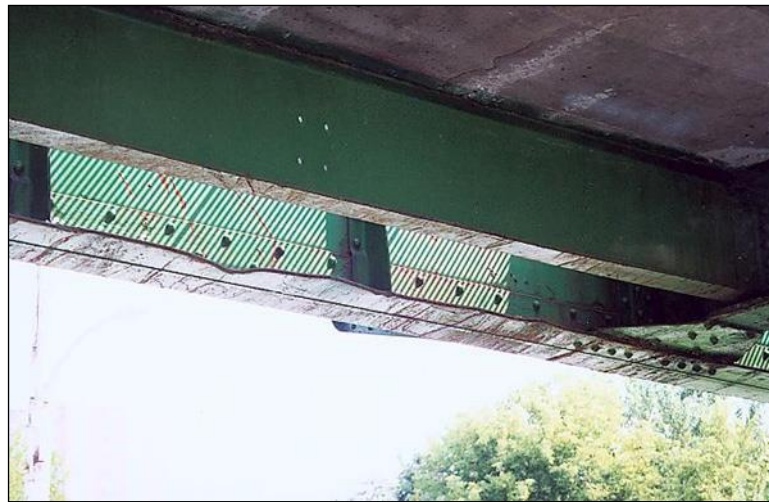
Figure 2.4.4.1-28: Impact Damage to Bottom Flange of a Two-Girder Bridge – Distortion Condition State 2.
