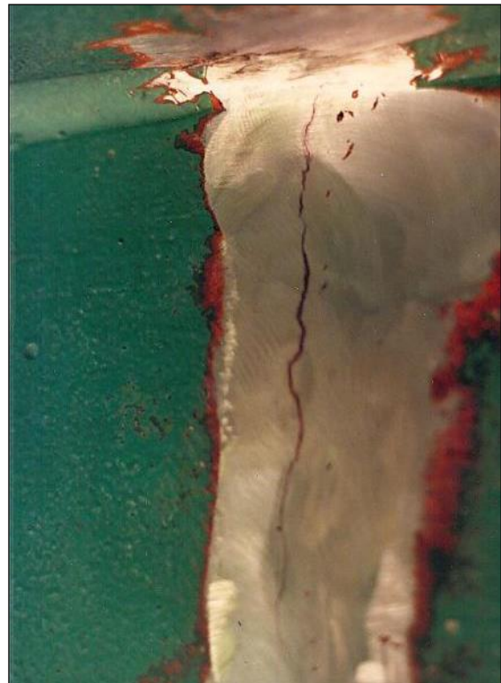
Figure 2.4.4.1-17: Unarrested Fatigue Crack - Condition State 3.
