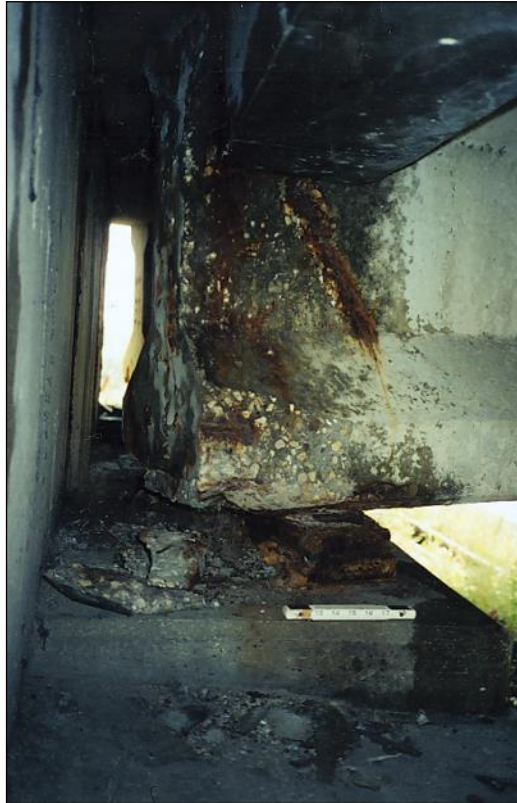
Figure 2.4.3.1-5: End of Prestressed I-Beam with Spalls and Exposed Strands and Rebar – Delamination/Spall/Patched Area Condition State 3.
