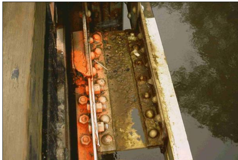
Figure 2.4.4.4-4: Batten Plate on Truss Bottom Chord – Connection Condition State 4.
