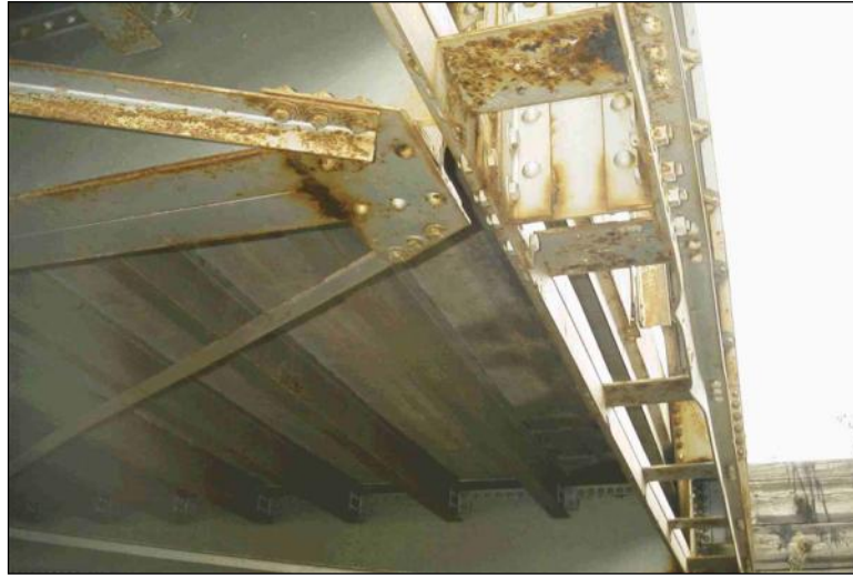
Figure 2.4.4.4-5: Truss Bottom Chord (Note Impact Damage) – Distortion Condition State 2.
