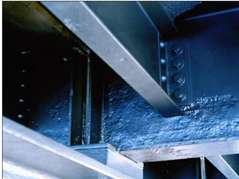
Figure 2.4.4.1-32: Section Loss on Girder Web Painted Over – Corrosion Condition State 3.
