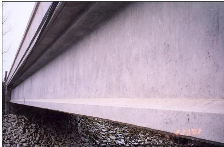
Figure 2.4.3.1-2: Prestressed I-Beam – Condition State 1.
