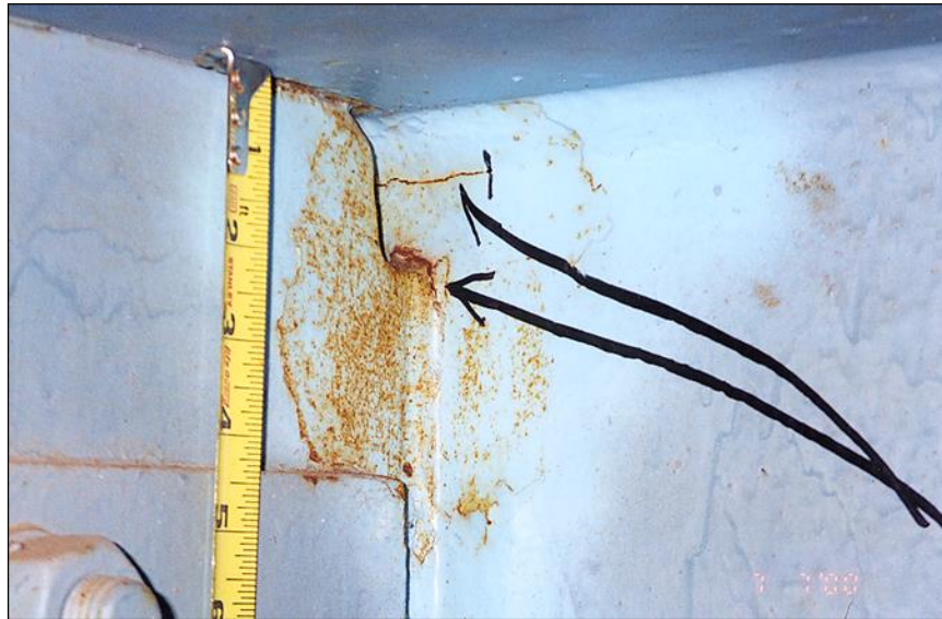
Figure 2.4.4.1-15: Double Fatigue Cracks in Girder Web, Top of Connection Plate – Condition State 3.
