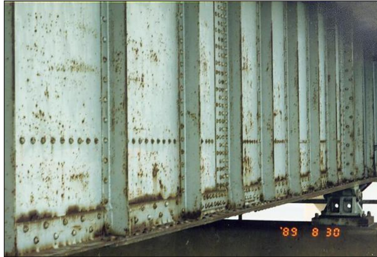
Figure 2.4.4.1-25: Steel Girder – Corrosion Condition State 2.
