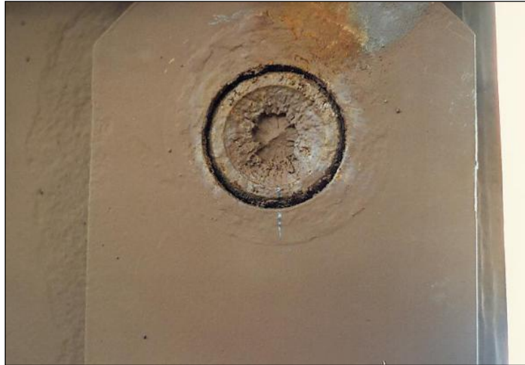
Figure 2.4.4.7-3: Pin Shear Failure.
