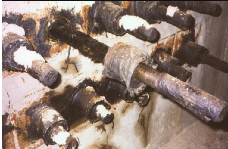
Figure 2.4.4.3-3: Protruding Post-Tensioning Rod – Connection Condition State 3.
