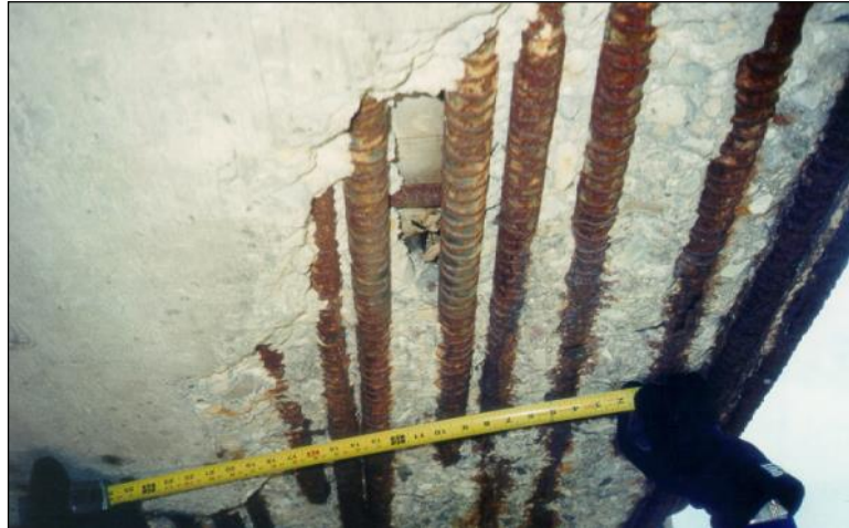
Figure 2.4.2.2-4: Corner of Reinforced Concrete Box Girder – Condition State 3.
