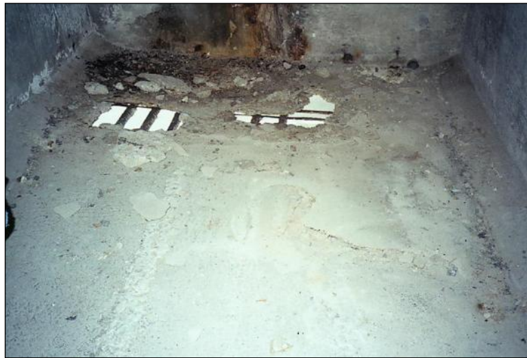
Figure 2.4.2.2-7: Reinforced Concrete Box Girder Bottom Flange Through Thickness Section Loss - Condition State 4.
