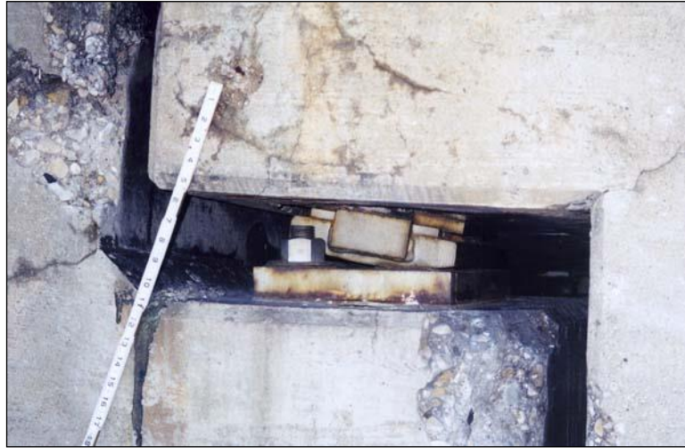
Figure 2.4.8.2-15: Severely Tipped Sliding Bearing – Movement Condition State 3.
