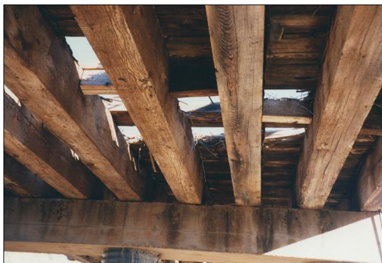
Figure 2.4.5.1-2: Timber Beams – Decay/Section Loss Condition State 1.
