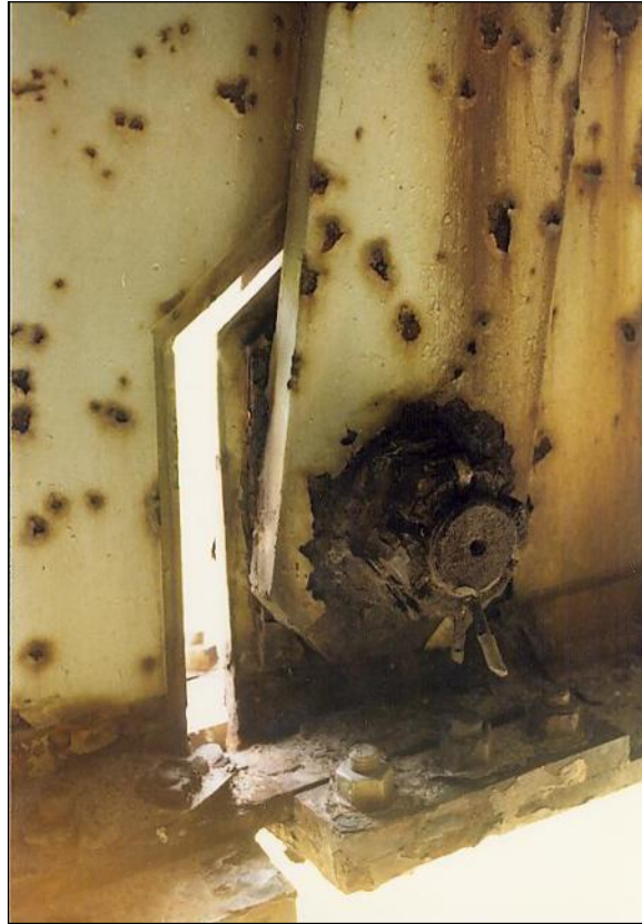
Figure 2.4.4.7-6: Pin and Hanger – Corrosion Condition State 4.
