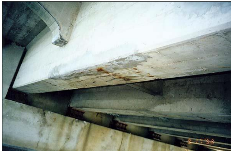
Figure 2.4.2.2-3: Reinforced Concrete Tee Beam – Condition State 2.
