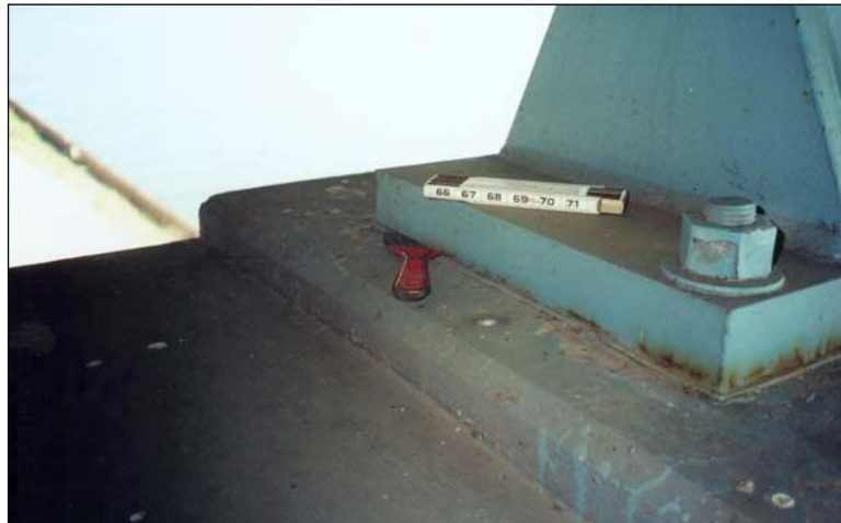
Figure 2.4.8.3-2: Slight Uplift on Masonry Plate – Movement Condition State 2.
