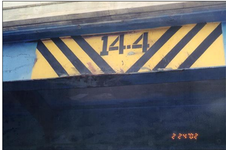
Figure 2.4.4.1-27: Impact Damage to a Girder Bottom Flange – Distortion Condition State 2.
