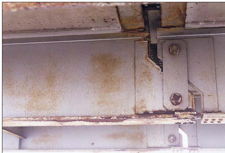
Figure 2.4.4.7-5: Girder, Pin, and Hanger – Corrosion Condition State 2.
