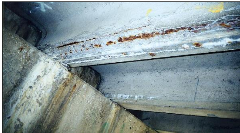
Figure 2.4.3.1-6: Prestressed Channel Beams with Exposed Strands, Longitudinal Cracks, Leaching, and Rust Staining – Cracking Condition State 4.
