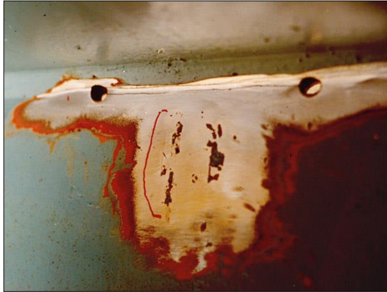
Figure 2.4.4.1-13: Fatigue Crack at Flange/Web Intersection After Cleaning – Condition State 2.
