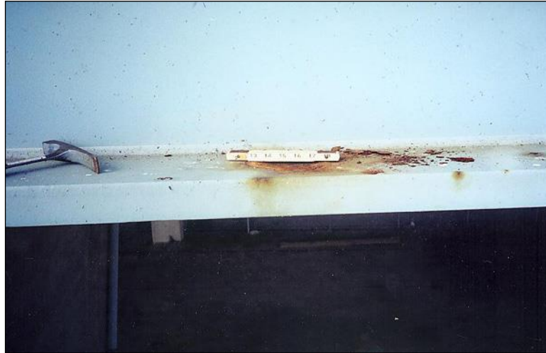
Figure 2.4.4.1-29: Pit Caused by Section Loss on Girder Bottom Flange – Corrosion Condition State 3.
