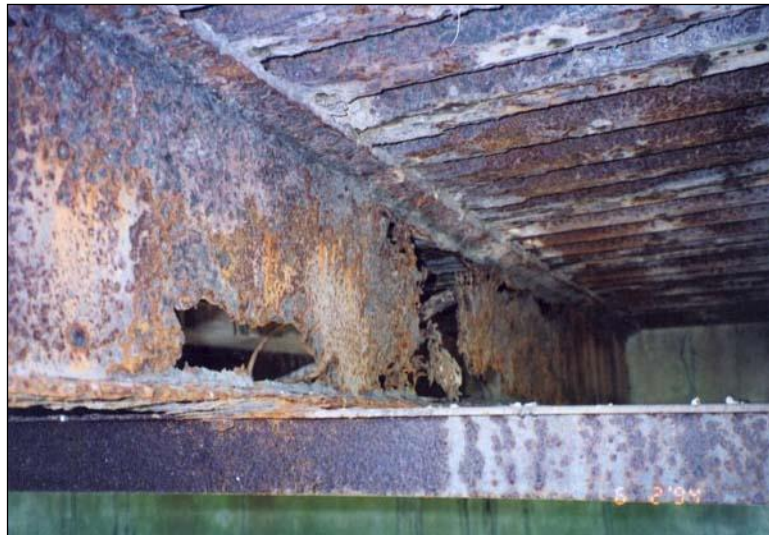
Figure 2.4.4.1-36: Steel Beam – Corrosion Condition State 4.
