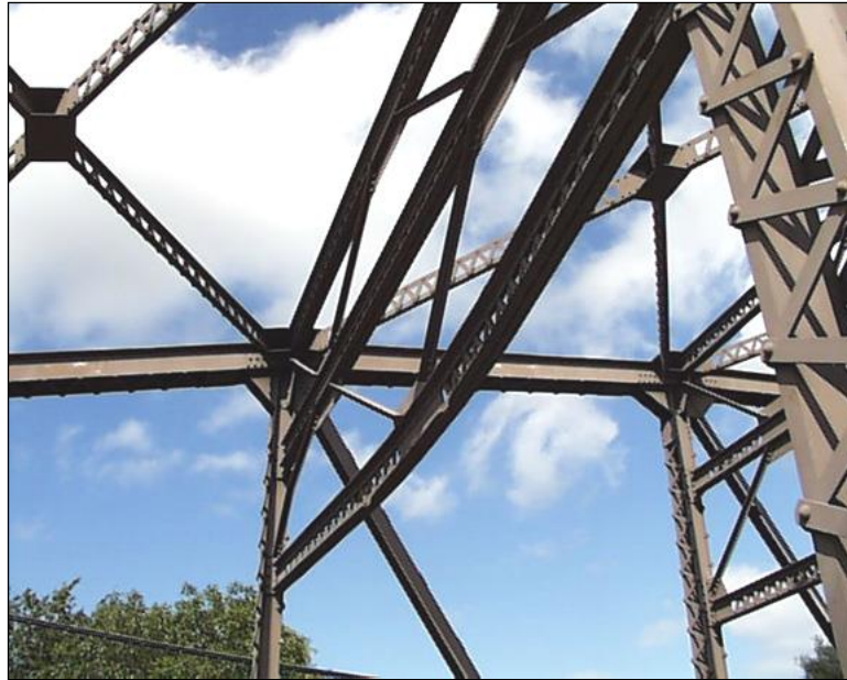
Figure 2.4.4.4-6: Impact Damage to a Truss Sway Strut – Distortion - Condition State 2.
