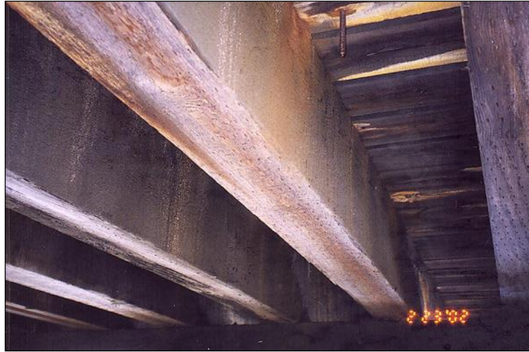
Figure 2.4.5.1-3: Timber Beams – Checks/Shakes/Cracks/Splits/Delaminations Condition State 1.
