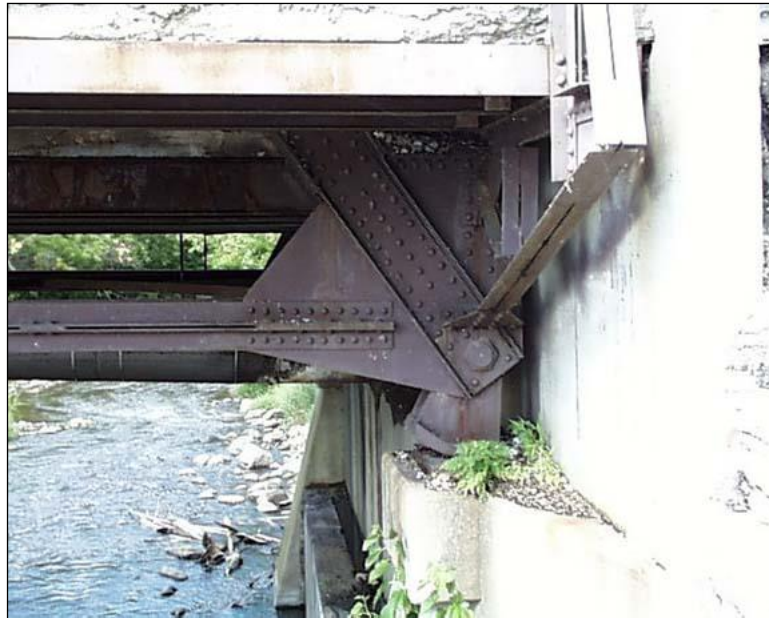
Figure 2.4.8.2-12: Rocker Bearing – Movement Condition State 3.
