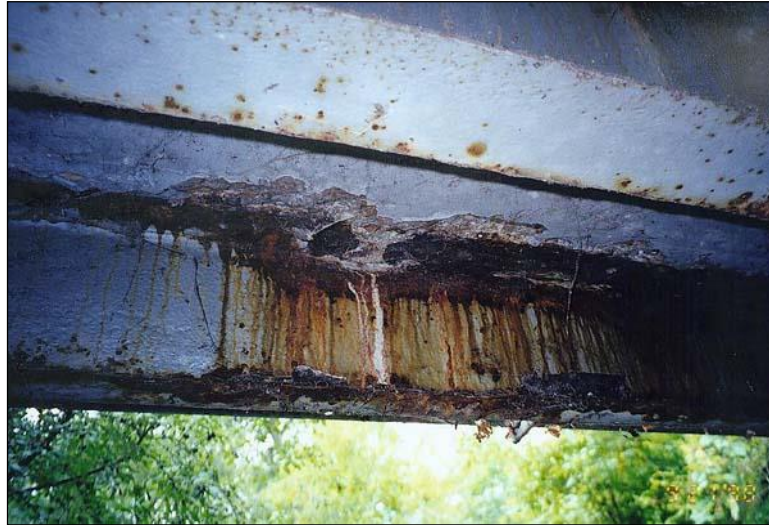
Figure 2.4.4.1-35: Steel Rolled Beams – Corrosion Condition State 4.
