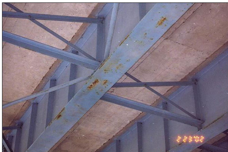
Figure 2.4.4.1-22: Steel Girders – Corrosion Condition State 2.
