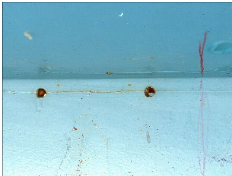
Figure 2.4.4.1-12: Fatigue Crack at Flange/Web Intersection Arrested with Drilled Holes - Condition State 2.
