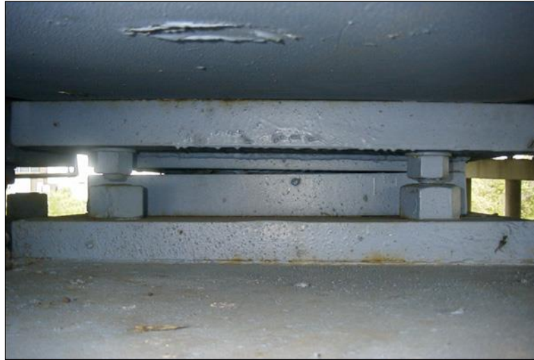
Figure 2.4.8.4-2: Tipped Pot Bearing – Movement Condition State 2.
