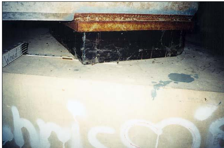
Figure 2.4.6.1-4: Uplift at Corner of Elastomeric Bearing – Movement Condition State 2.
