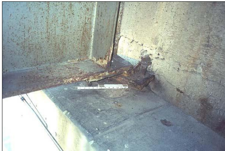
Figure 2.4.8.2-14: Masonry Plate Walkout Due to Failed Anchor Bolt – Connection Condition State 3.
