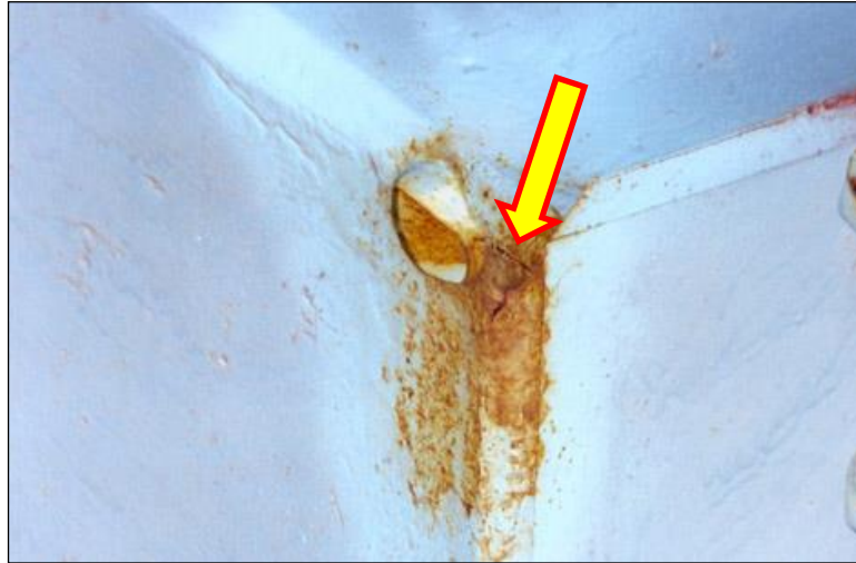
Figure 2.4.4.1-11: Fatigue Crack Through Girder Web Arrested with a Drilled Hole, Top of Connection Plate - Condition State 2.
