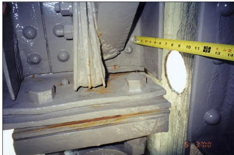
Figure 2.4.4.1-38: Heavy Pack Rust (Painted Over) at a Multiple Plate Bearing Stiffener – Connection Condition State 4.
