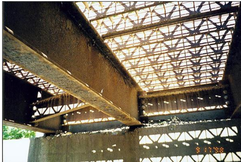
Figure 2.4.4.1-21: Weathering Steel Girders with Scaling on the Bottom Flanges – Condition State 3.
