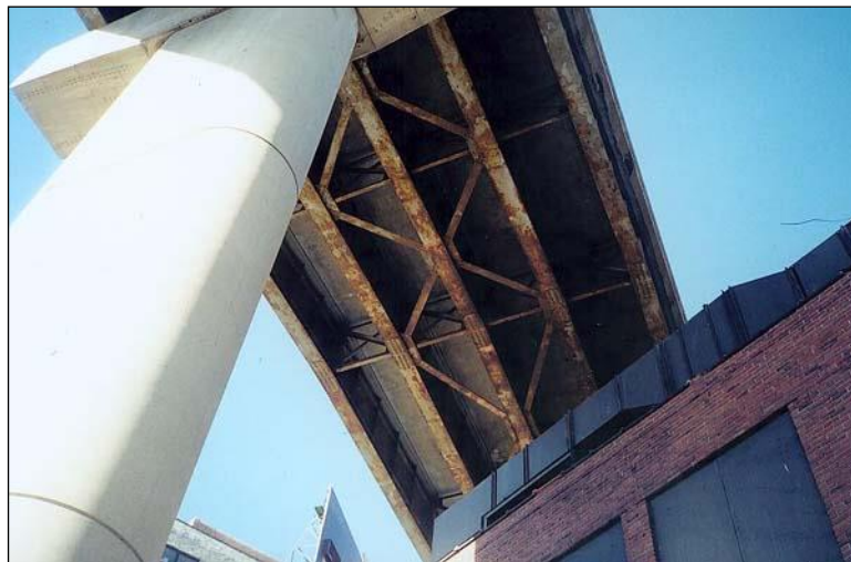
Figure 2.4.4.1-30: Steel Girders – Corrosion Condition State 3.
