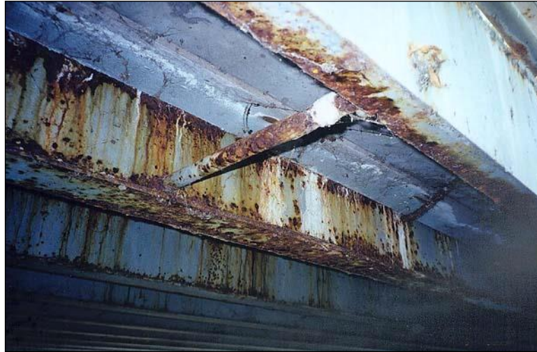
Figure 2.4.4.1-31: Steel Girders – Corrosion Condition State 3.
