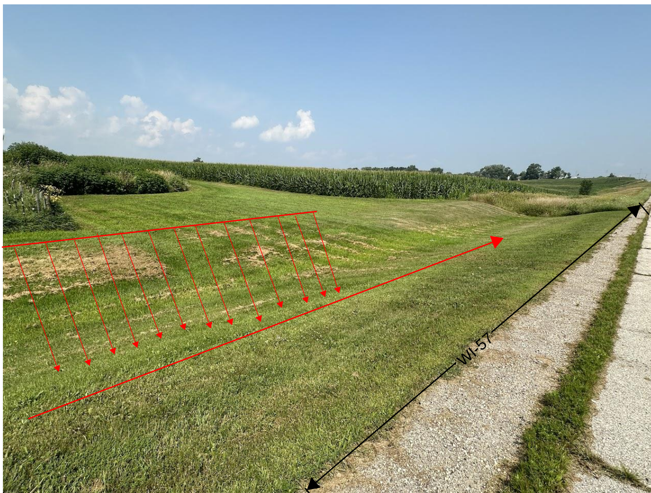
Photo taken north of the unnamed farm on the same side of WI-57. Runoff collects into the roadside ditch and flows downstream from south to north.
