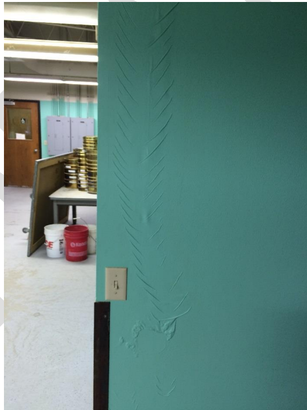
FIGURE 23 Water damage near electrical switch due to leaking roof.
