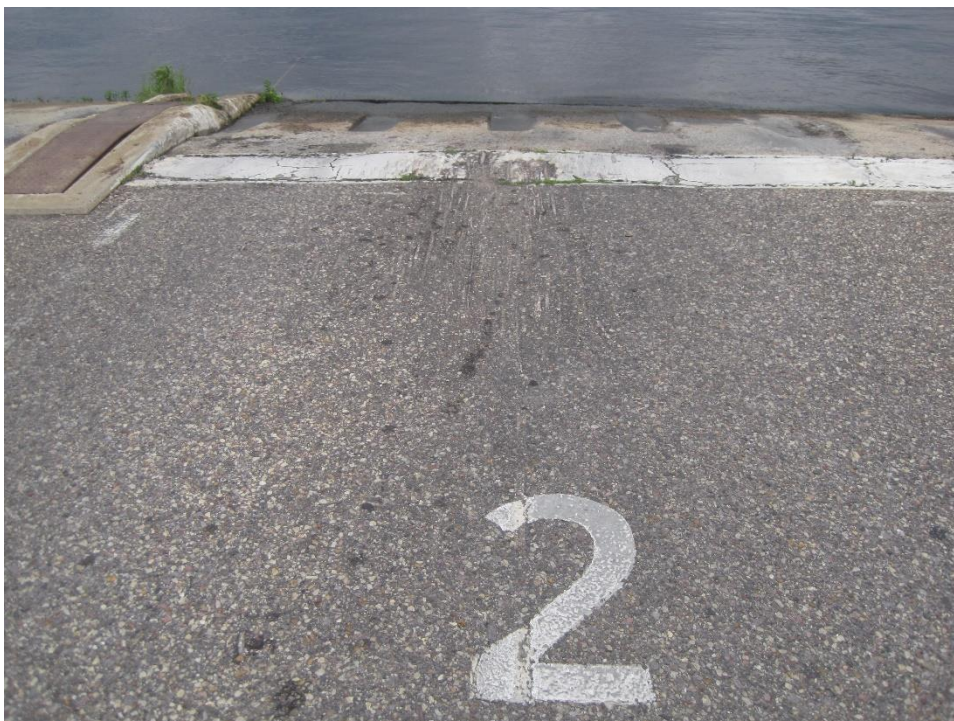
Figure 8: Asphalt abrasion at loading lane centerline, North Ramp
