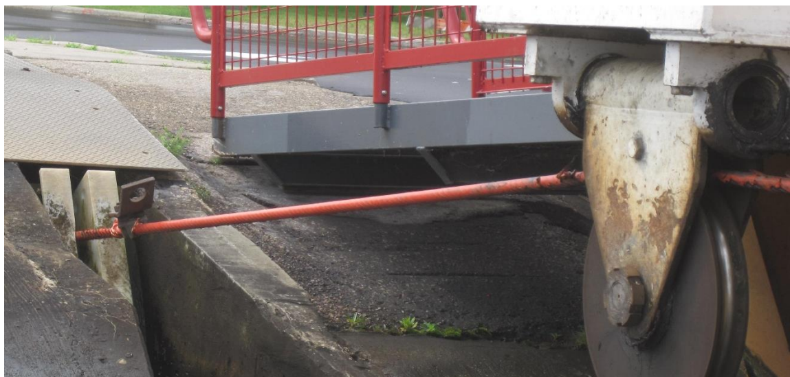
Figure 19: East Guide Cable at south Landing, worn coating
