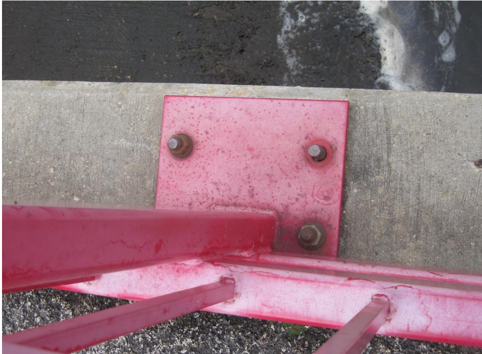
Figure 3: Typical Missing pedestrian railing Anchor bolt nut, SE landing shown.
