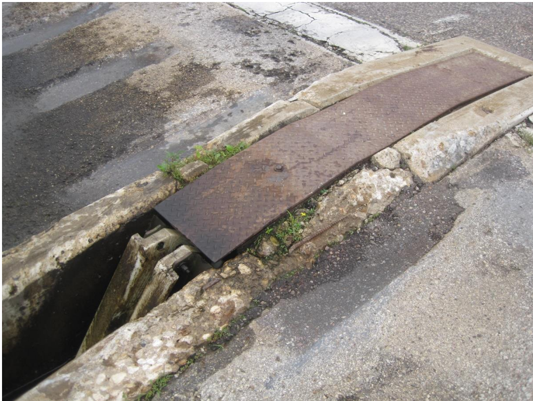
Figure 16: Drive Cable trough concrete spalling, North Landing
