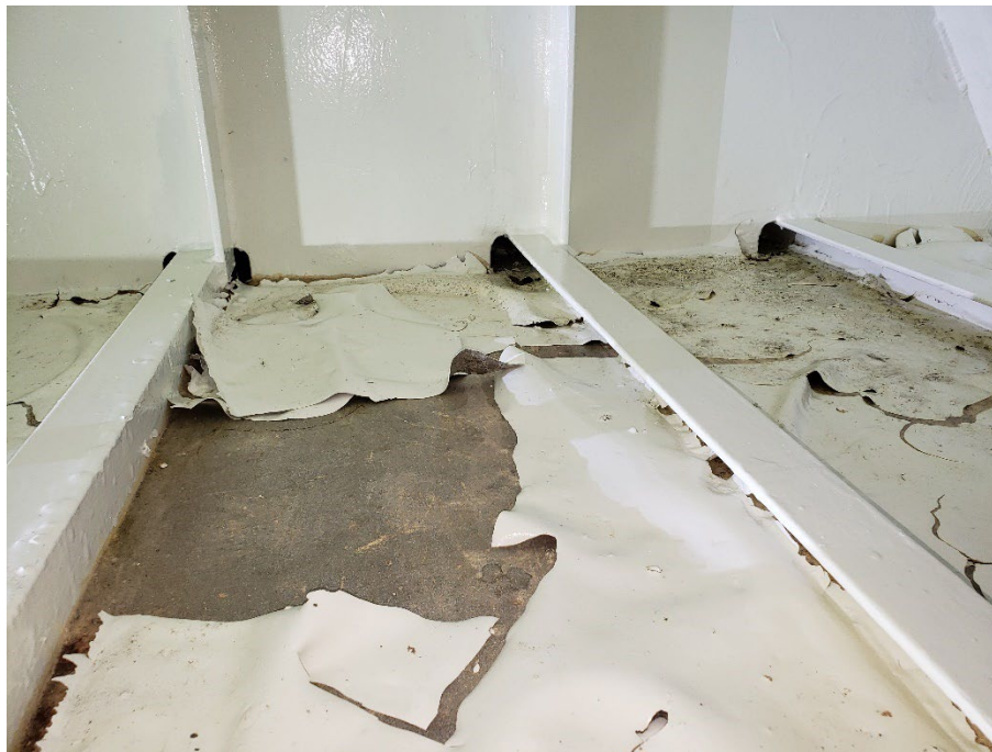
Figure 9: Coating Failure in Cross Deck Structure, North End
