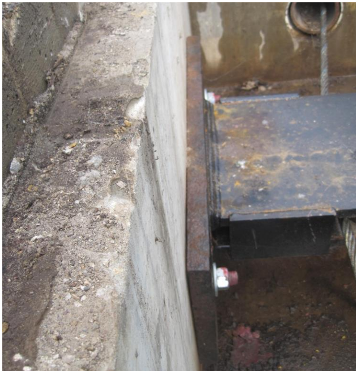
Figure 14: Directional sheave, slight gap beneath south end of baseplate
