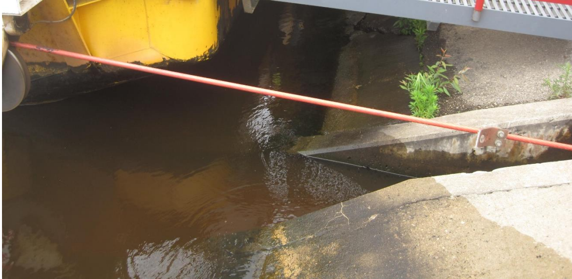
Figure 22: Minor concrete spalling due to mooring clamp at northeast guide cable trough
