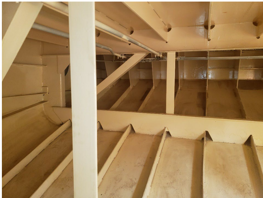
Figure 7: General Hull Structure Condition Image, North End Rake
