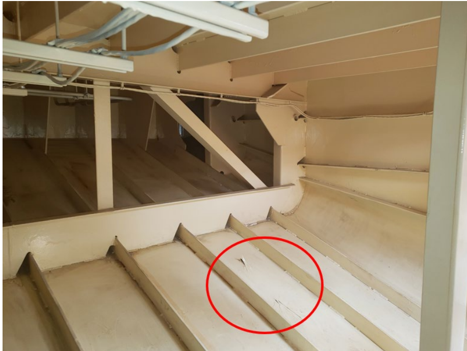
Figure 10: North End Bottom Shell Deformation (re-paint area)
