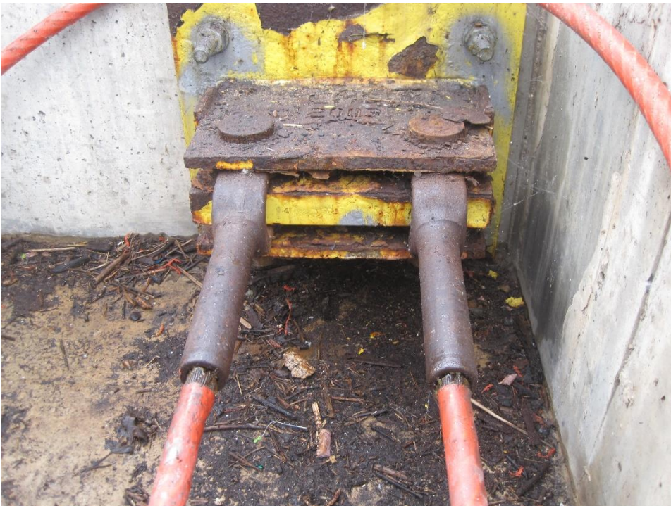
Figure 21: Corrosion of Anchor plate and short anchor cables at south anchor of east guide cable
