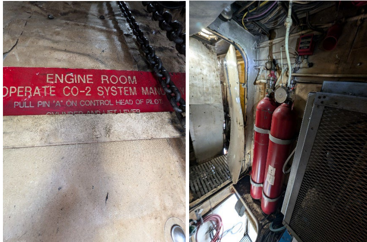
Figure 5: Manual Activation Placard, CO 2 Cylinders Above North Engine
