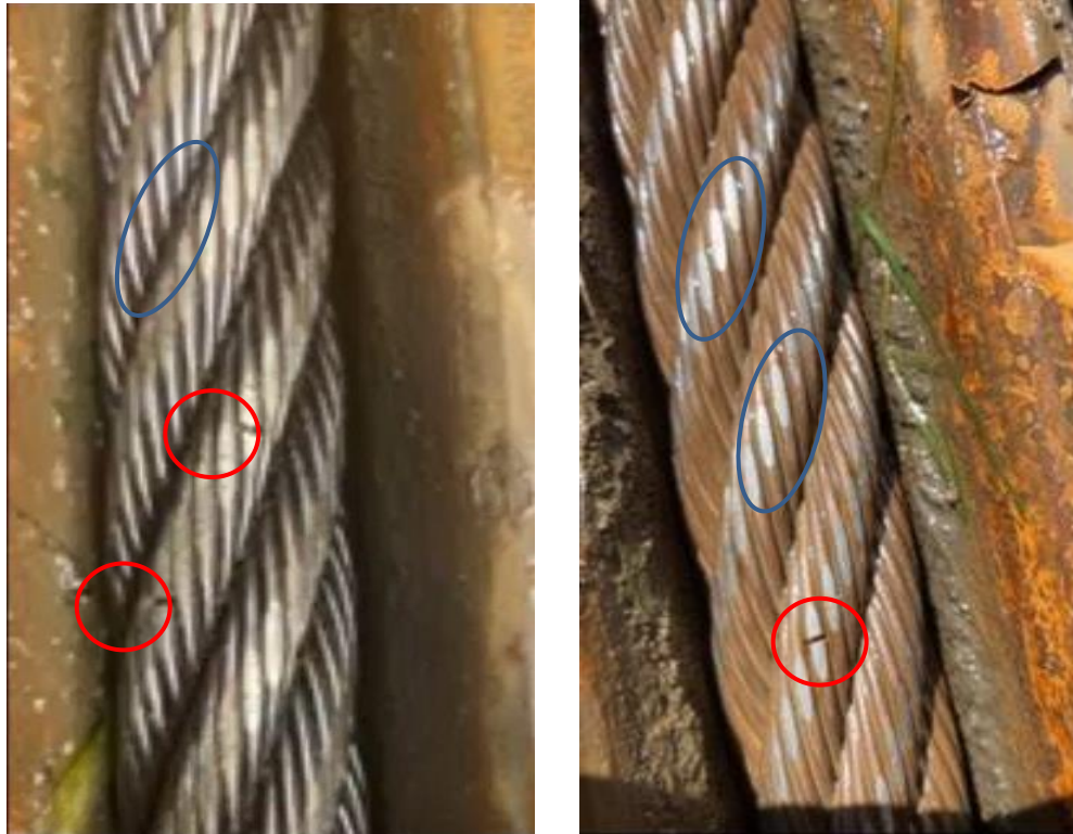
Figure 10: Example of cracks on the crown wired are circled in red and flat spots are circled in blue
