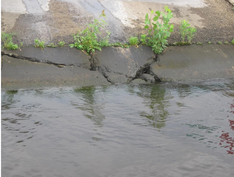
Figure 7: Cracked and deteriorated Concrete, North Landing, Lane 1
