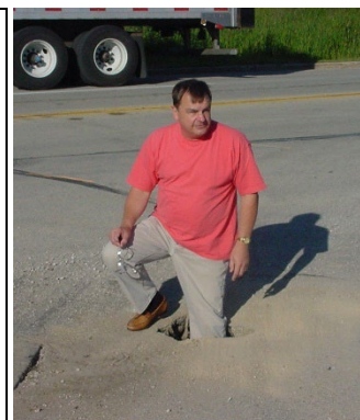
Figure 3: Improper pothole restoration
