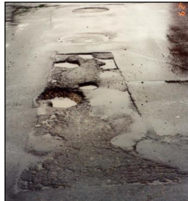
Figure 45: Both patches improperly backfilled/compacted, and not patched to nearest joint or seam
