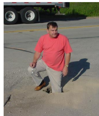
Figure 23: Improper pothole restoration
