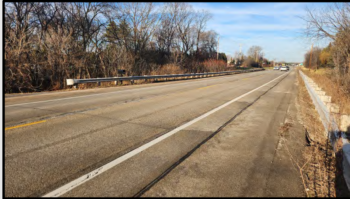
Example of WIS 32/57 pavement deterioration
