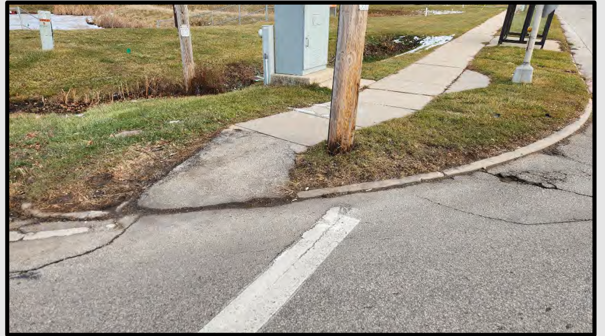
Example of non-compliant curb ramp (SE corner of WIS 32/57 & Cook St)
