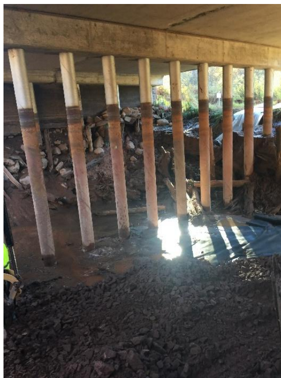
Figure 5 – 2016 Scour damage at B-02-006, Kakagon Slough
