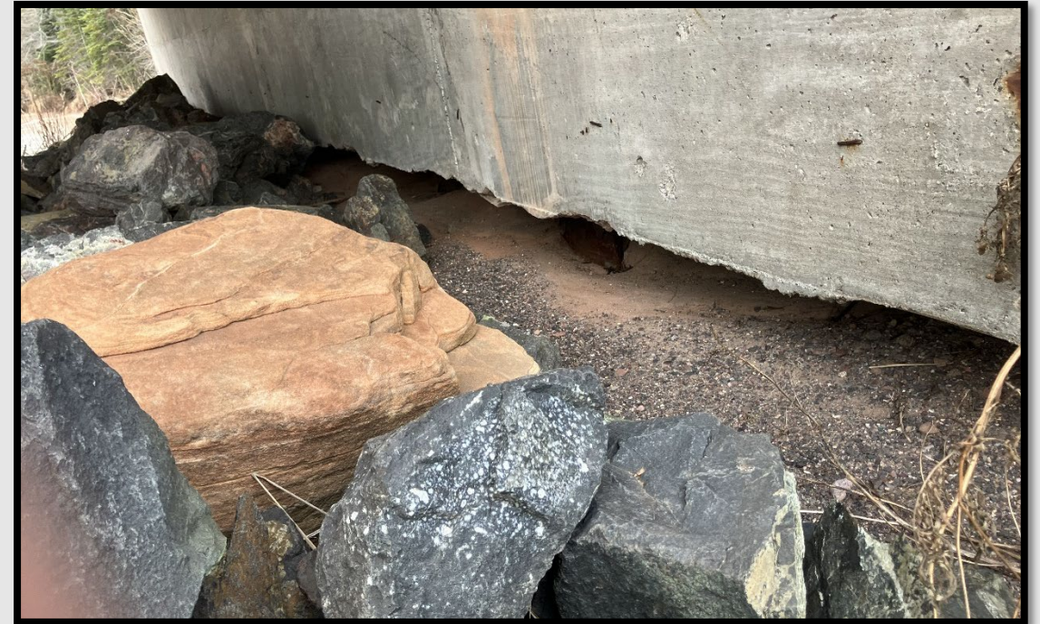
Settlement around Fish Creek Bridge abutment
