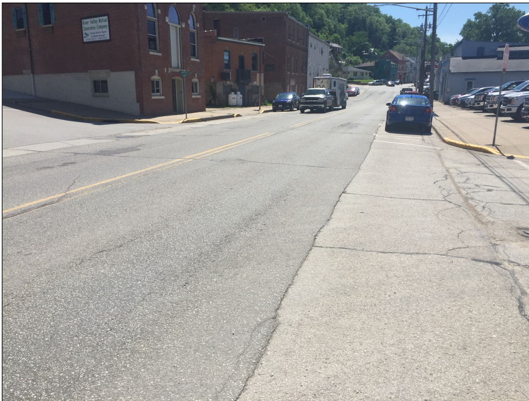
Deteriotating pavement in Fountain City along WIS 35
