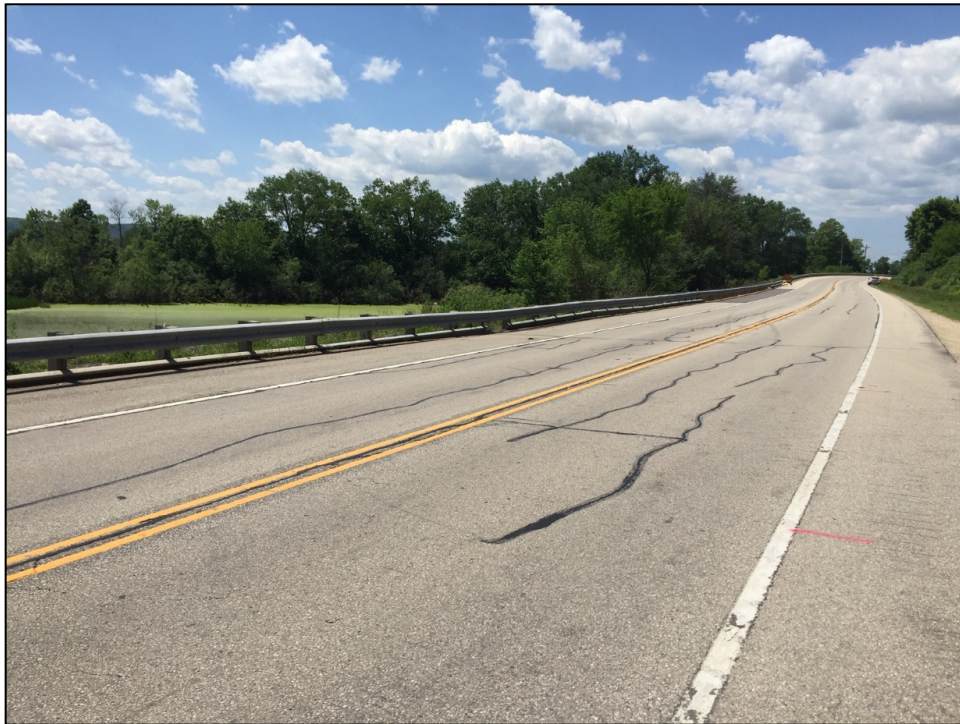
Deteriotating pavement and beam guard in need of replacement along WIS 35
