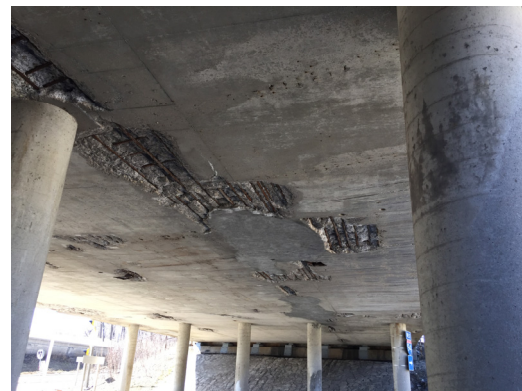
Deteriorating infrastructure (photo shows Stadium Interchange bridge)
