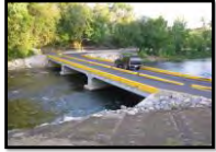
Example of a concrete bridge (not representative of all possible project types).
