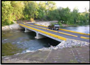
Example of a concrete bridge (not representative of all possible project types).
