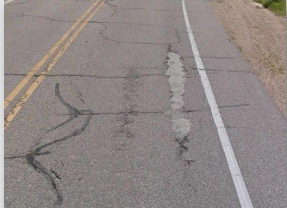
WIS 23 Raveling and Patchwork
