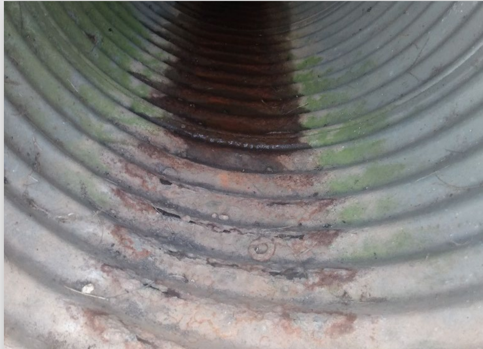
Deteriorated Culvert Pipe
