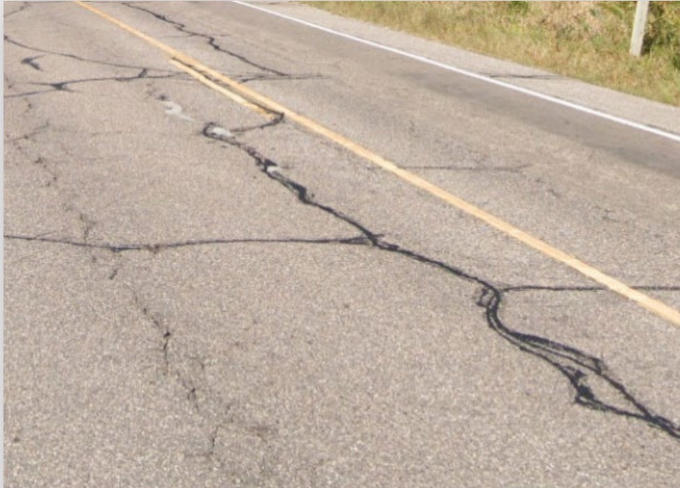
WIS 23 Fatigue Cracking and Rutting
