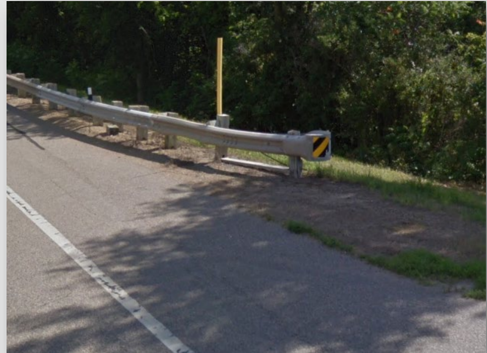
Existing end of guardrail on WIS 23
