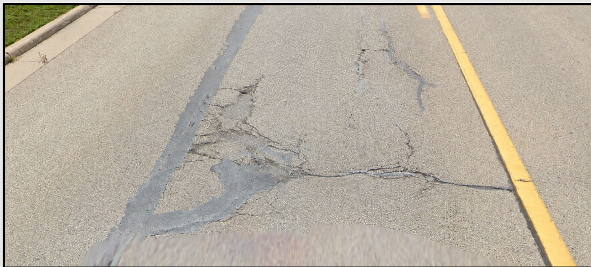
Example of longitudinal and fatigue cracking on WIS 73
