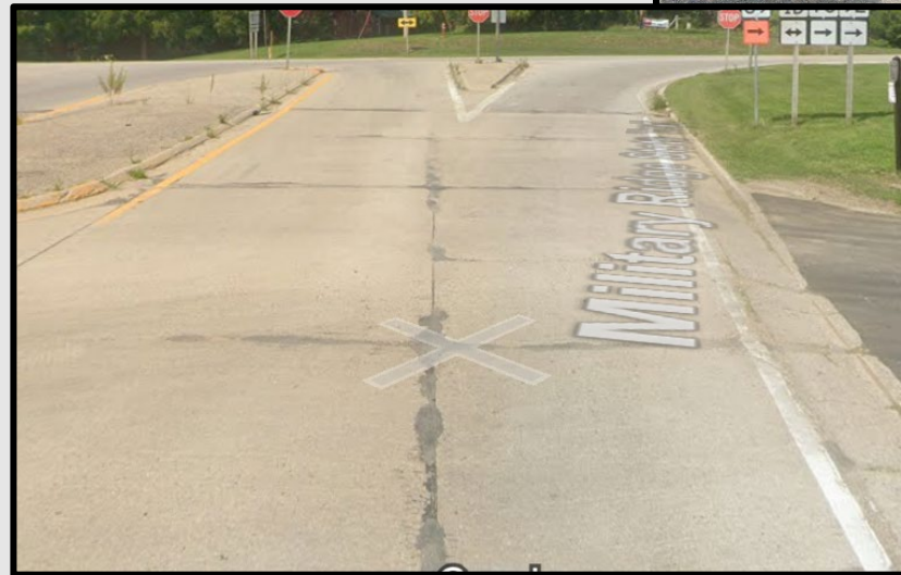
Example of concrete cracking on WIS 78 (south)
