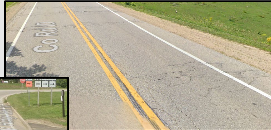
Example of alligator cracking on WIS 78 (east)
