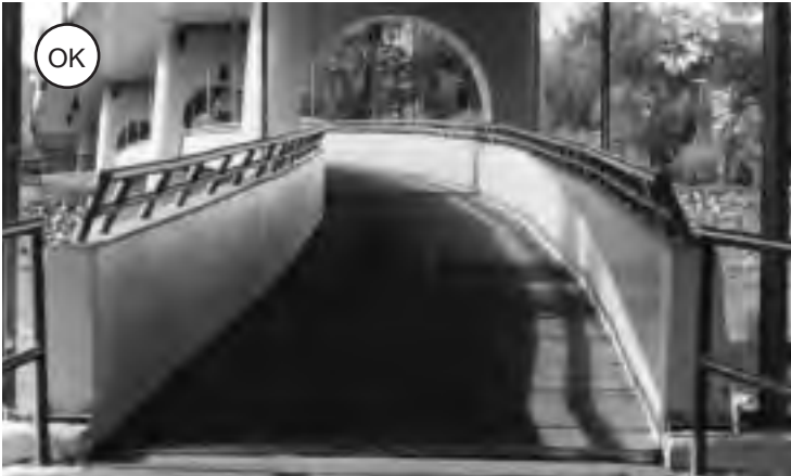
Figure 4-119: This bridge's width was limited by openings in the supports for the transit bridge above. It was further narrowed by angling railings inward.
