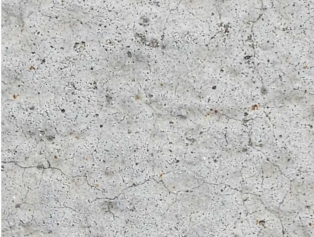
Figure 24 Localized overlay map cracking observed on Bridge B40-336 eight months after placement.
