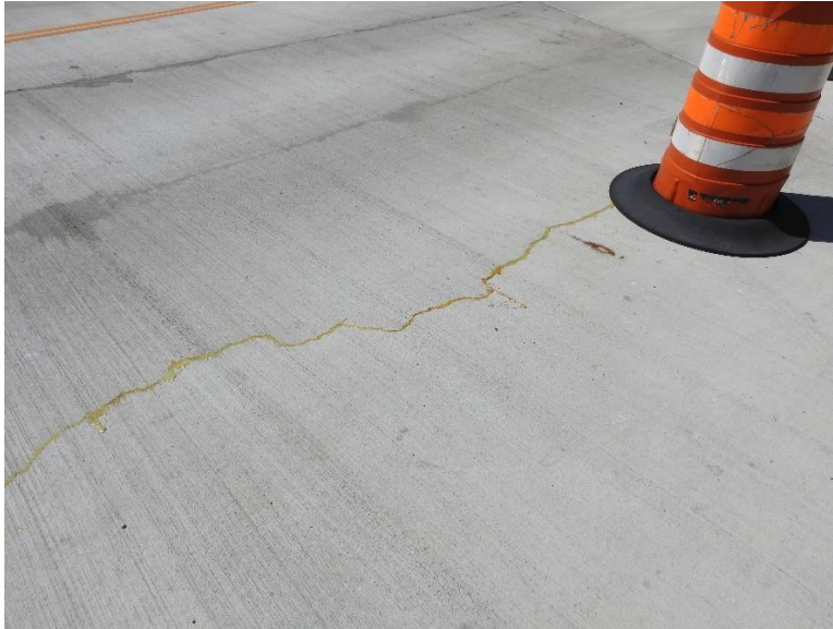
Figure 14. Large crack in B67-099 (epoxy sealed).
