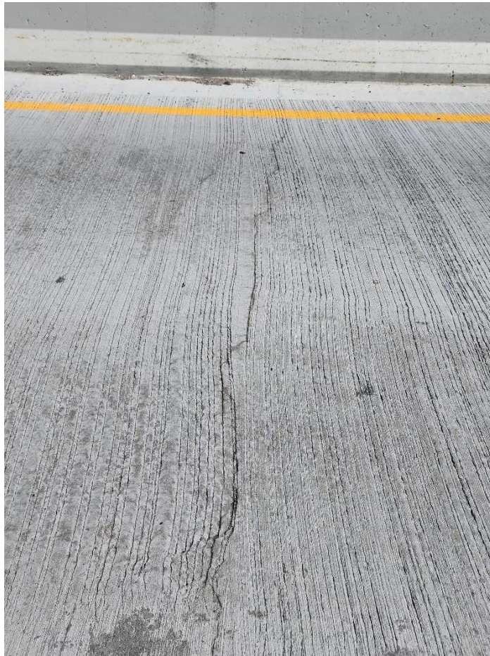
Figure 23 Overlay cracking observed on Bridge B40-336 eight months after placement.
