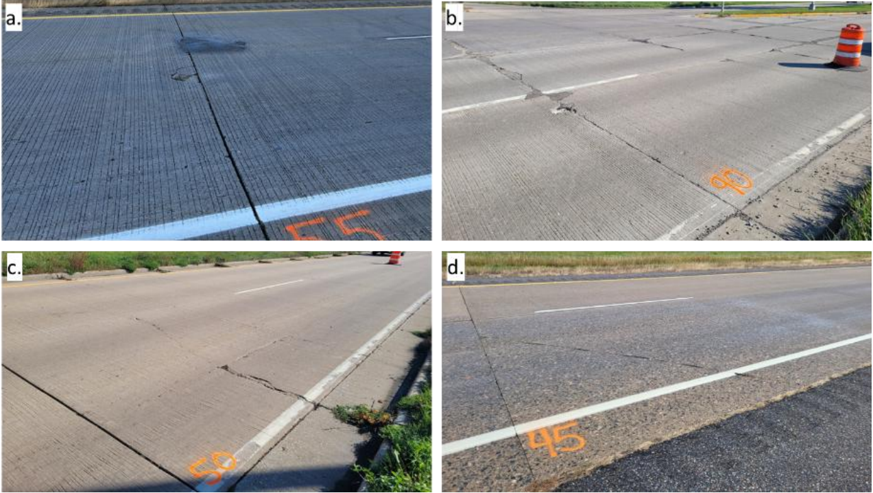
Figure 6. (a) Joint spalling in Eau Claire County on STH 53, (b) joint spalling in Jefferson County on US 12 EB, (c) cracking in Jefferson County on US 12 EB, and (d) cracking in Wood County on US 10 EB.
