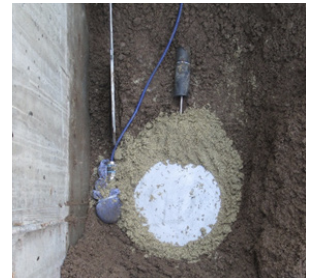
Vertical Earth Pressure Cell and Pore Pressure Sensor Installation at Hobbles Creek Bridge
