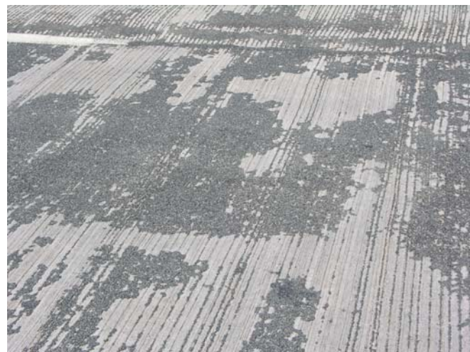
Photo 4: Area of extreme surface loss on STH 35
