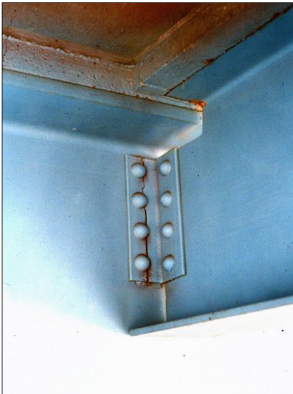
Figure 2.4.4.1-16: Fatigue Crack Through the Rivet Line of a Connection Angle - Condition State 3.
