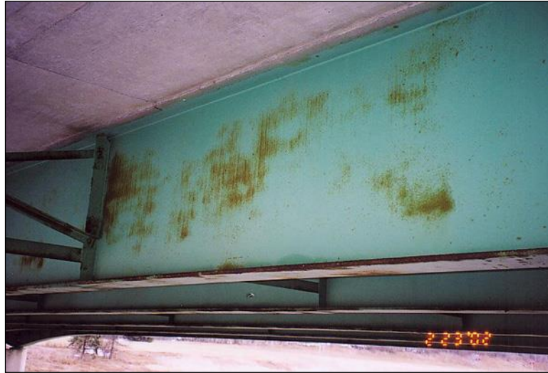
Figure 2.4.4.1-23: Girder – Corrosion Condition State 2.
