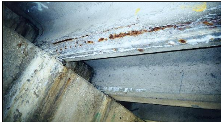
Figure 2.4.3.1-6: Prestressed Channel Beams with Exposed Strands, Longitudinal Cracks, Leaching, and Rust Staining – Cracking Condition State 4.
