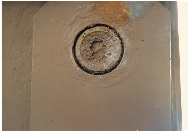
Figure 2.4.4.7-3: Pin Shear Failure.
