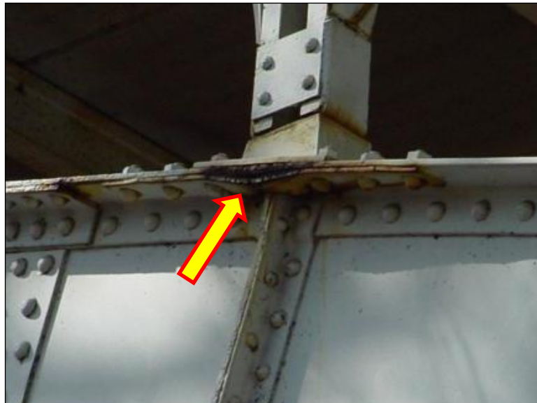
Figure 2.4.4.6-2: Pack Rust at Riveted Steel Arch Flange Plates – Connection Condition State 3.
