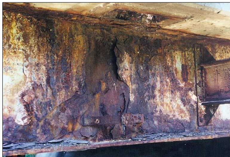
Figure 2.4.4.1-34: Laminate Section Loss of Web – Corrosion Condition State 4.
