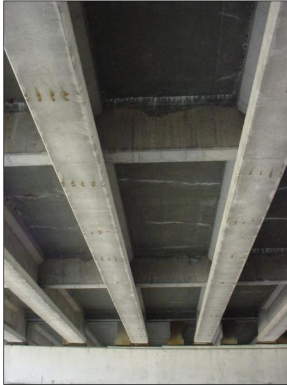
Figure 2.4.3.1-3: Prestressed I-Beams – Condition State 1.
