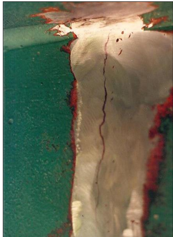
Figure 2.4.4.1-17: Unarrested Fatigue Crack - Condition State 3.
