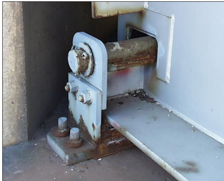
Figure 2.4.8.2-10: Hold-Down (Restraining) Bearing - Corrosion Condition State 2.
