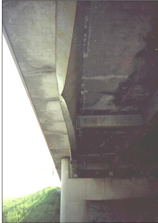
Figure 2.4.4.1-39: Impact Damage to Exterior Girder – Distortion Condition State 4.
