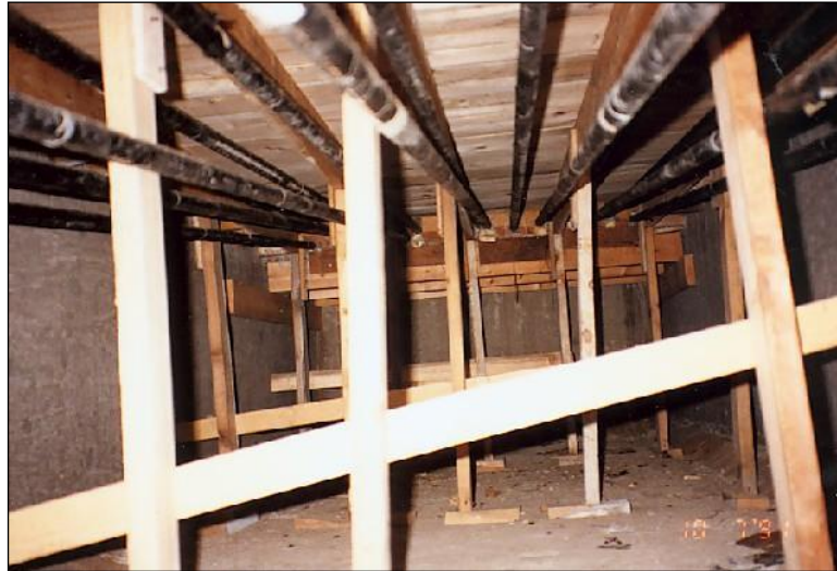
Figure 2.4.4.3-1: Exposed Post Tensioning Rods Inside of a Concrete Box Girder - Condition State 1.
