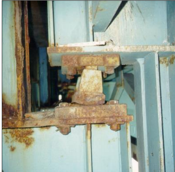
Figure 2.4.8.2-9: Rocker Bearing – Condition State 2.
