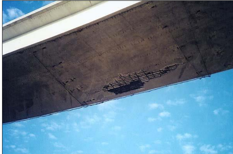
Figure 2.4.2.2-6: Reinforced Concrete Box Girder Bottom Flange Through Thickness Section Loss - Condition State 4.
