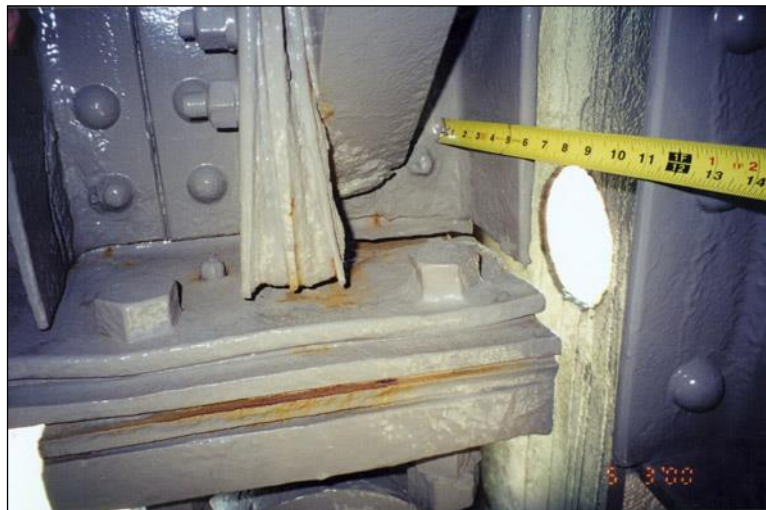
Figure 2.4.4.1-38: Heavy Pack Rust (Painted Over) at a Multiple Plate Bearing Stiffener – Connection Condition State 4.
