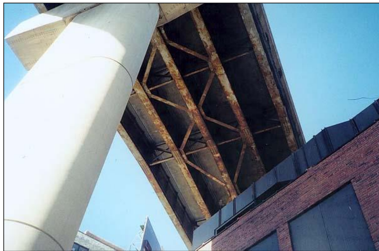
Figure 2.4.4.1-30: Steel Girders – Corrosion Condition State 3.
