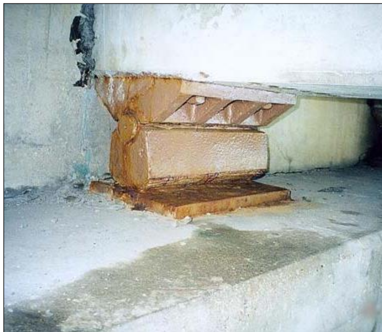
Figure 2.4.8.2-8: Rocker Bearing – Corrosion Condition State 2.
