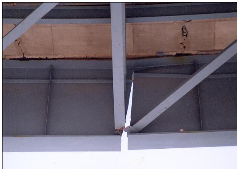
Figure 2.4.4.1-3: Girder Failure Due to Brittle Cracking – Condition State 4.
