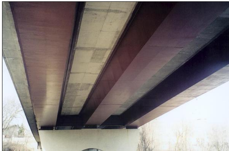
Figure 2.4.4.1-18: Steel Box Girders - Condition State 1.
