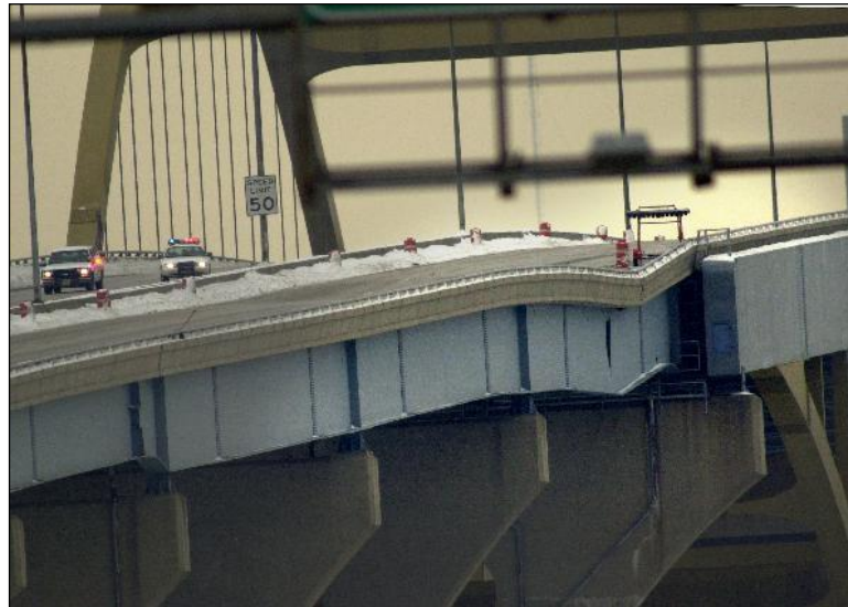
Figure 2.4.4.1-4: Girder Failure Due to Brittle Cracking – Condition State 4.
