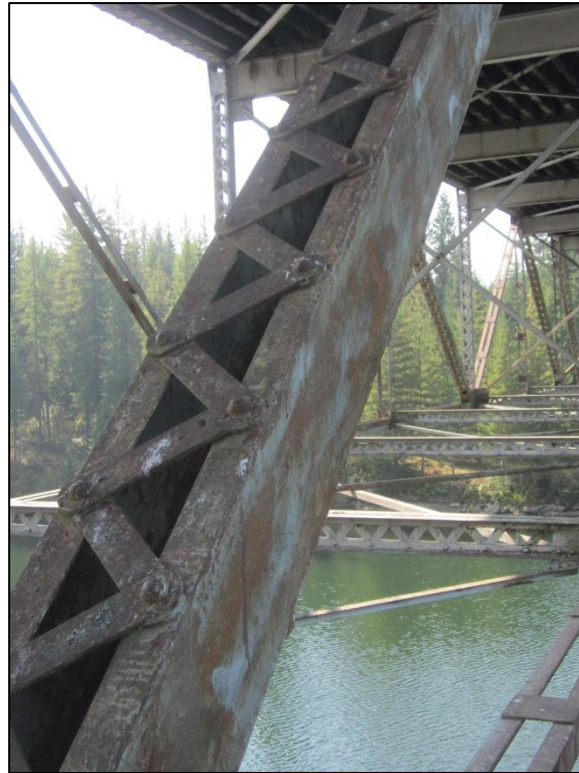
Figure 2.4.4.4-3: Diagonal Truss Member Exhibiting Rust with No Loss of Section – Corrosion Condition State 2.
