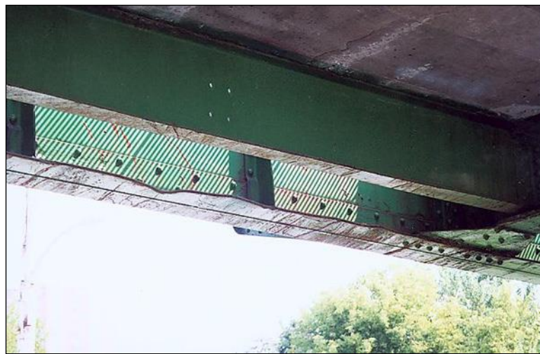
Figure 2.4.4.1-28: Impact Damage to Bottom Flange of a Two-Girder Bridge – Distortion Condition State 2.
