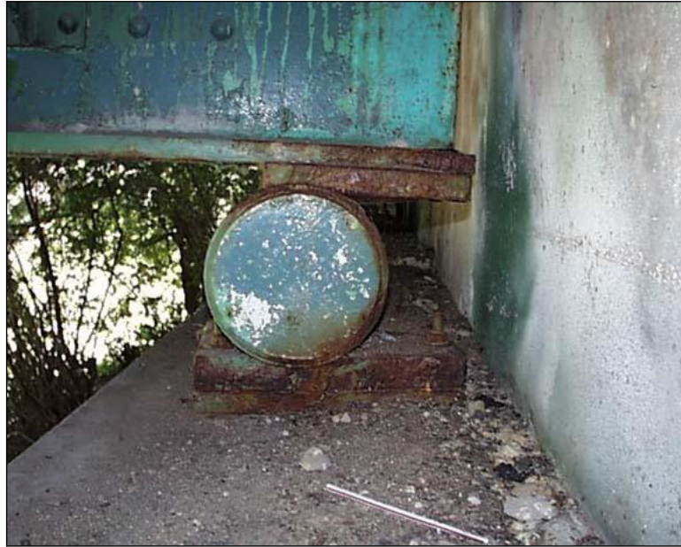
Figure 2.4.8.2-11: Critically Misaligned Roller Bearing – Alignment Condition State 3.
