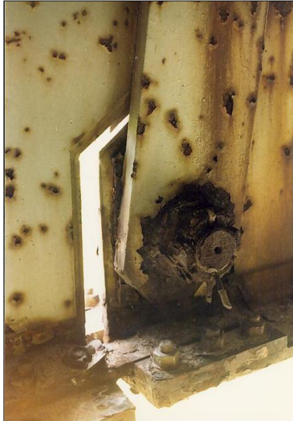
Figure 2.4.4.7-6: Pin and Hanger – Corrosion Condition State 4.
