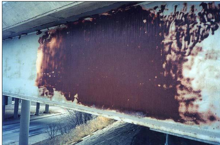
Figure 2.4.4.1-24: Steel Girder – Corrosion Condition State 2.
