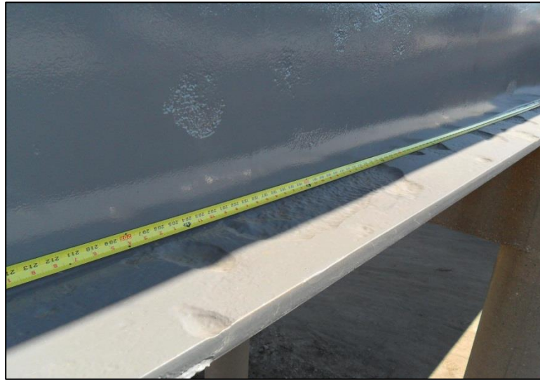
Figure 2.4.4.1-33: Severe Pitting Along Bottom Flange Painted Over – Corrosion Condition State 4.
