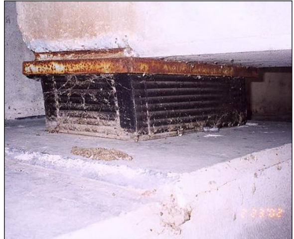
Figure 2.4.6.1-3: Elastomeric Bearing Experiencing Shear Deformation – Condition State 1.
