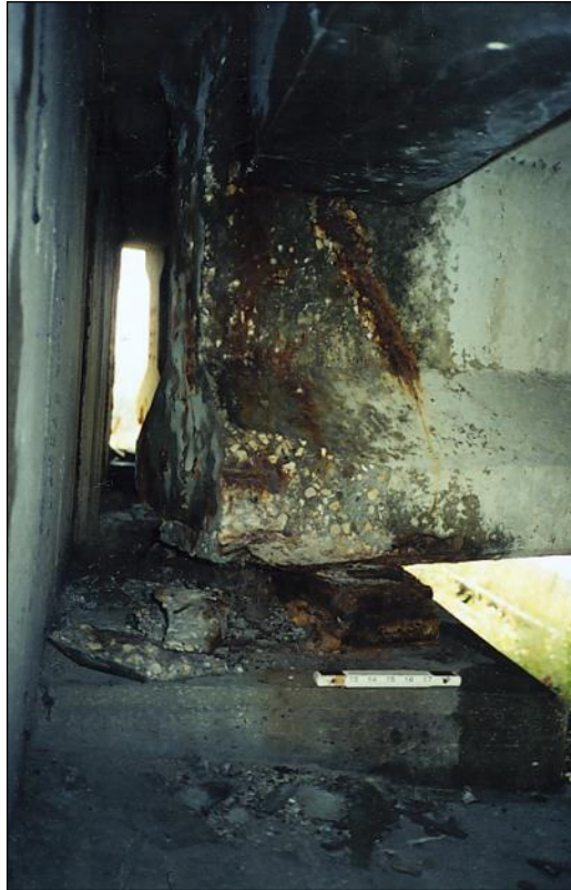
Figure 2.4.3.1-5: End of Prestressed I-Beam with Spalls and Exposed Strands and Rebar – Delamination/Spall/Patched Area Condition State 3.
