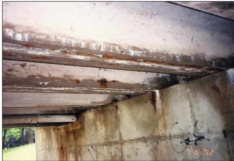
Figure 2.4.3.1-4: Prestressed Channel Beams – Cracking Condition State 3.
