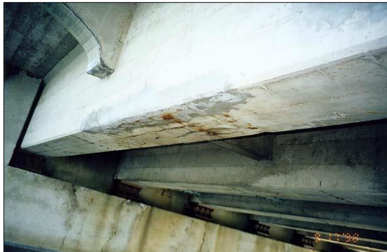
Figure 2.4.2.2-3: Reinforced Concrete Tee Beam – Condition State 2.
