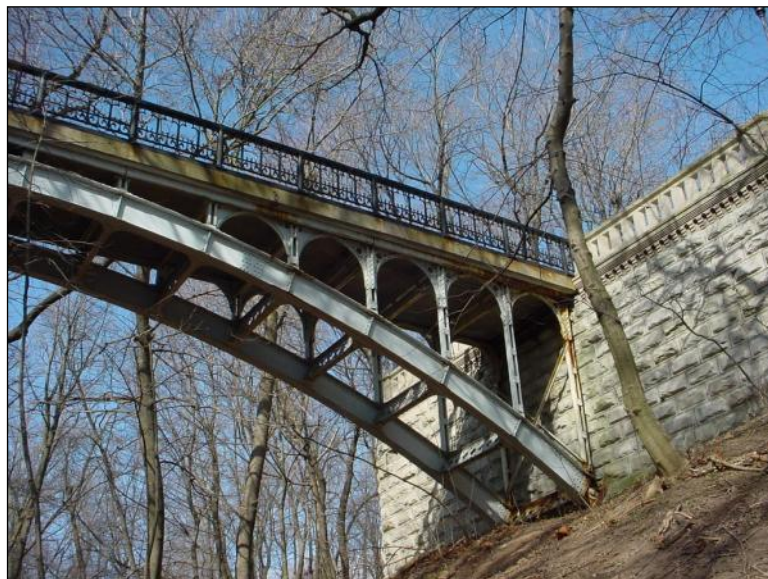
Figure 2.4.4.6-1: Steel Arch and Spandrel Bent Columns.
