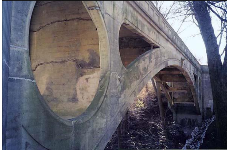
Figure 2.4.2.3-2: Open Spandrel Reinforced Concrete Arch – Cracking Condition State 2.
