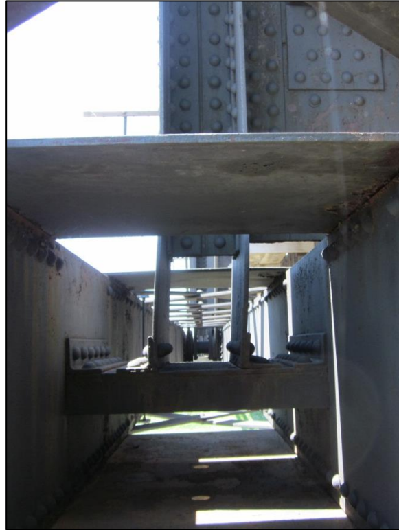
Figure 2.4.4.5-1: Vertical to Bottom Chord Gusset Plate Deformed Out-of-Plane – Distortion Condition State 2.
