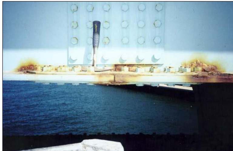
Figure 2.4.4.1-26: Pack Rust at Bolted Girder Bottom Flange Field Splice – Connection Condition State 2.
