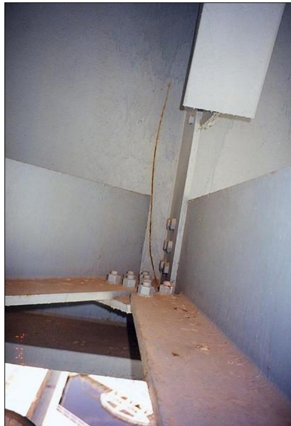
Figure 2.4.4.1-6: Same Crack as shown in Figure 4.75, Inside Face of Girder at Lower Lateral Shelf Plate - Condition State 4.
