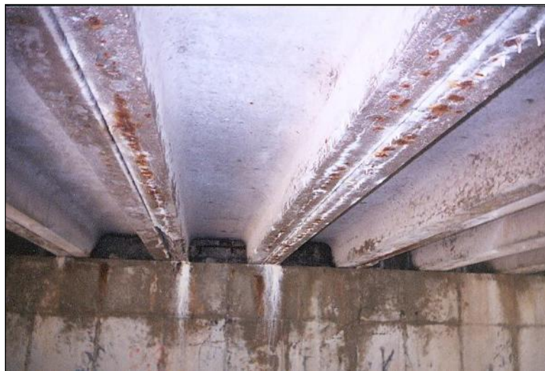
Figure 2.4.3-4: Deteriorated Prestressed Channel Beams.
