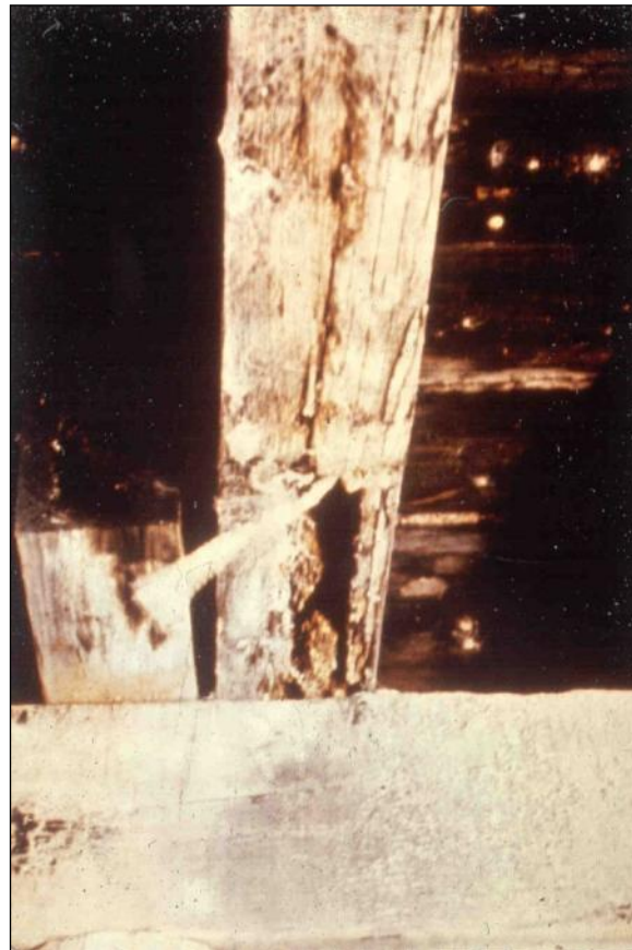
Figure 2.4.5.1-4: Timber Beam – Decay/Section Loss Condition State 4.
