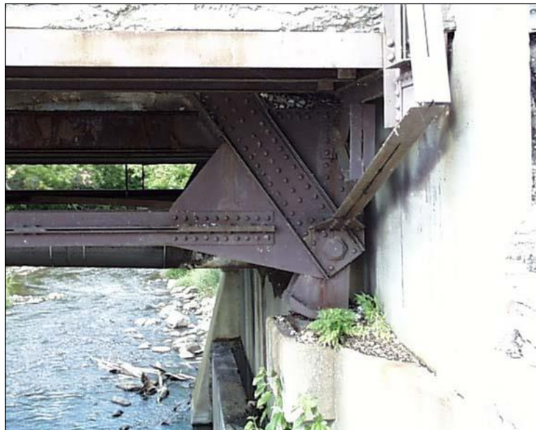
Figure 2.4.8.2-12: Rocker Bearing – Movement Condition State 3.
