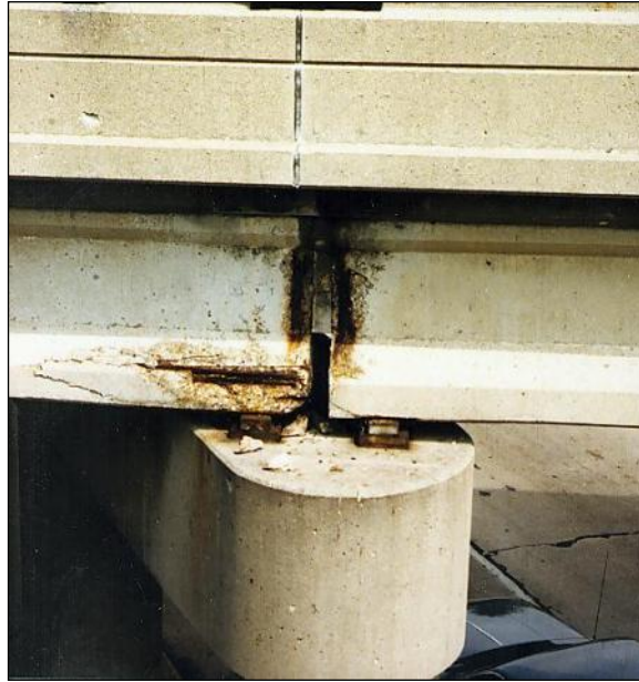
Figure 2.4.3.1-7: Delaminated/Spalled Prestressed Beam End with Exposed Strands – Exposed Prestressing Condition State 4.
