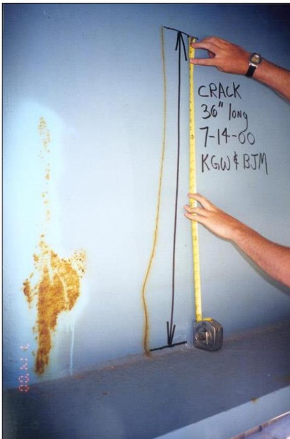
Figure 2.4.4.1-5: Brittle Crack 3 Feet Long in a Girder Web 10 Feet Deep, Opposite of Lower Lateral Shelf Plate - Condition State 4.
