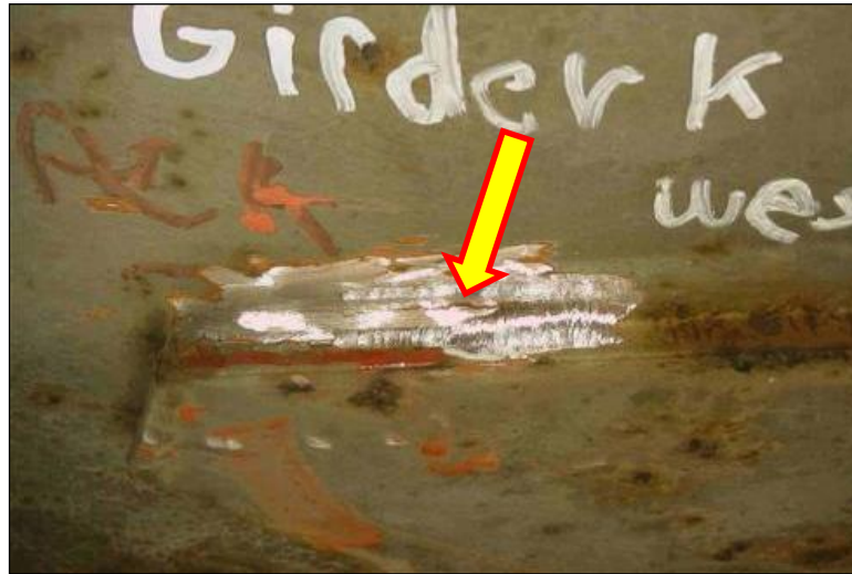
Figure 2.4.4.1-7: Fatigue Crack at a Welded Cover Plate End (Rust Line within the Ground Area).
