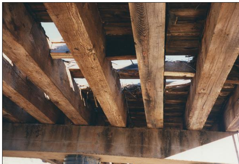
Figure 2.4.5.1-2: Timber Beams – Decay/Section Loss Condition State 1.
