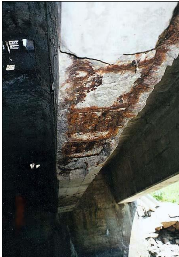
Figure 2.4.2.2-5: Reinforced Concrete Tee Beam – Condition State 4.
