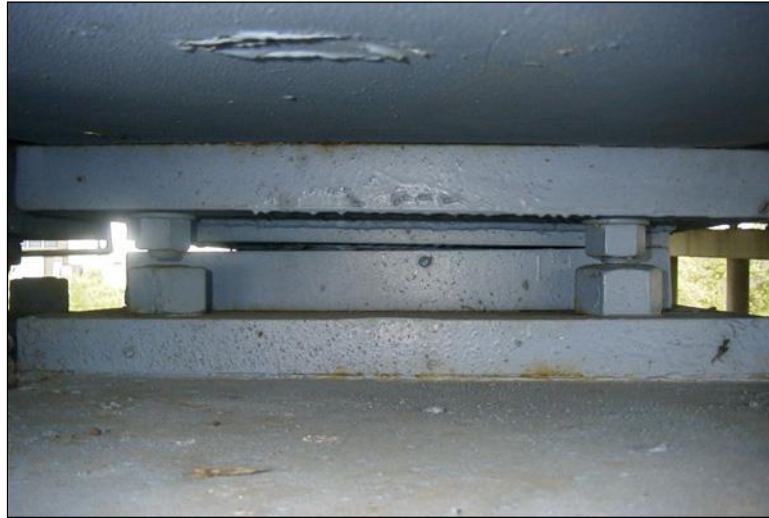
Figure 2.4.8.4-2: Tipped Pot Bearing – Movement Condition State 2.
