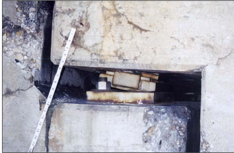
Figure 2.4.8.2-15: Severely Tipped Sliding Bearing – Movement Condition State 3.
