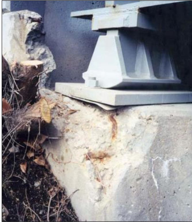
Figure 2.4.8.2-7: Rocker – Loss of Bearing Area Condition State 2
