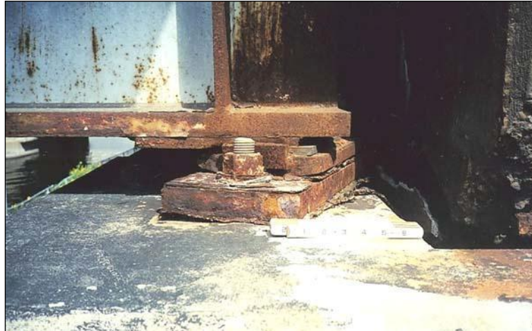
Figure 2.4.8.2-13: Masonry Plate Walking Out Due to Failed Anchor Bolt – Connection Condition State 3.
