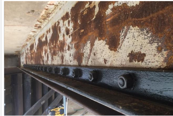
Maintenance and Rehab Needs
