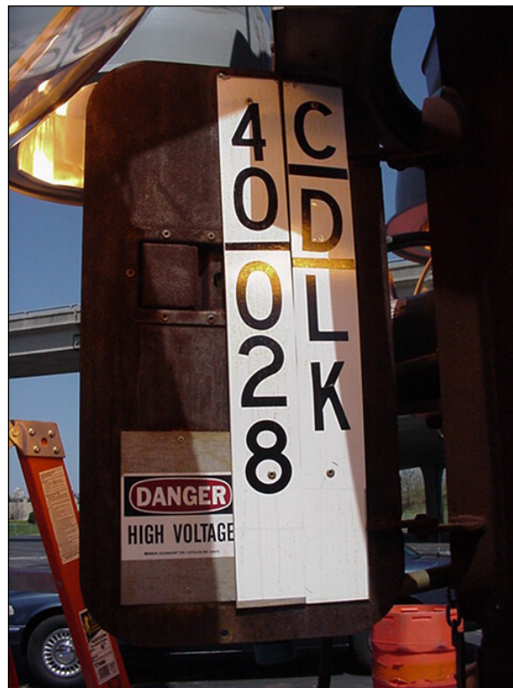
Figure 1.5.2.3-1: Structure Plaque and Circuit Plaque Mounted on a High mast Hatch Door. (Note that the location number “028” would read “0028” according to current convention.)
