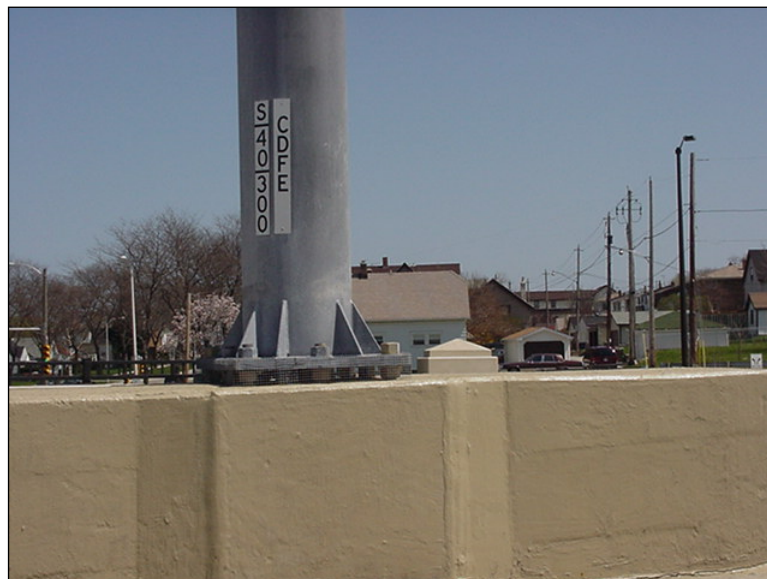
Figure 1.5.2.2-1: Structure Plaque and Circuit Plaque Mounted on a Sign Bridge. (Note that the location number “300” would read “0300” according to current convention.)
