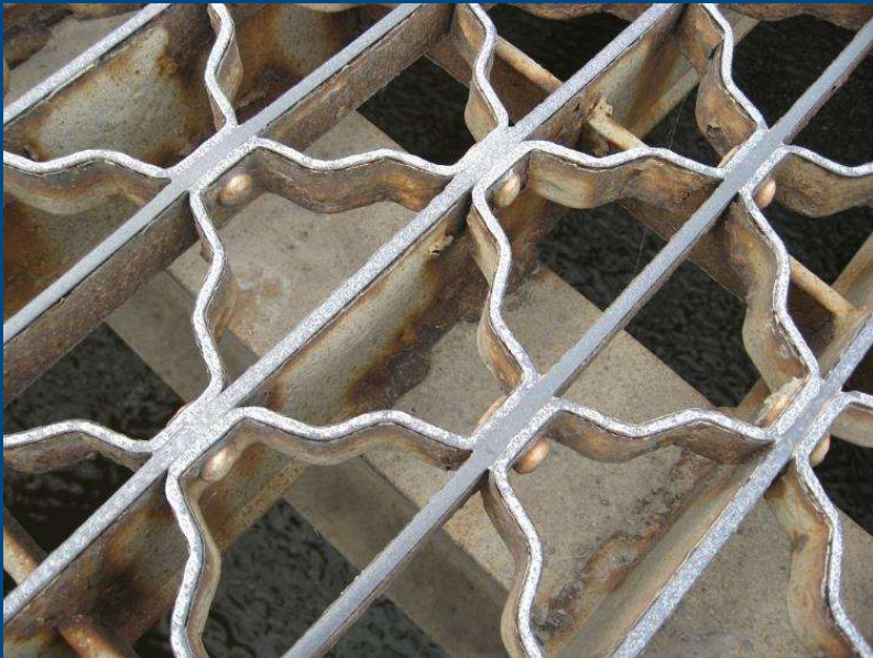
Bascule Deck Grating
