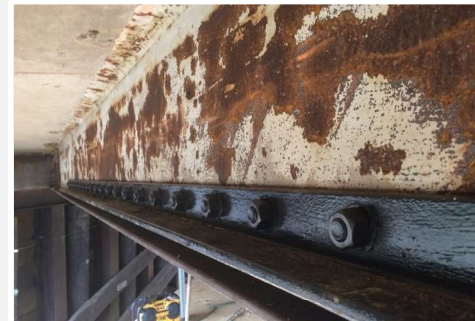
Maintenance and Rehab Needs
