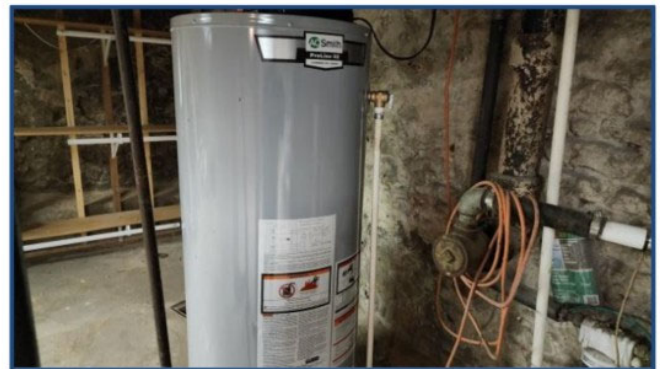
Basement Water Heater
