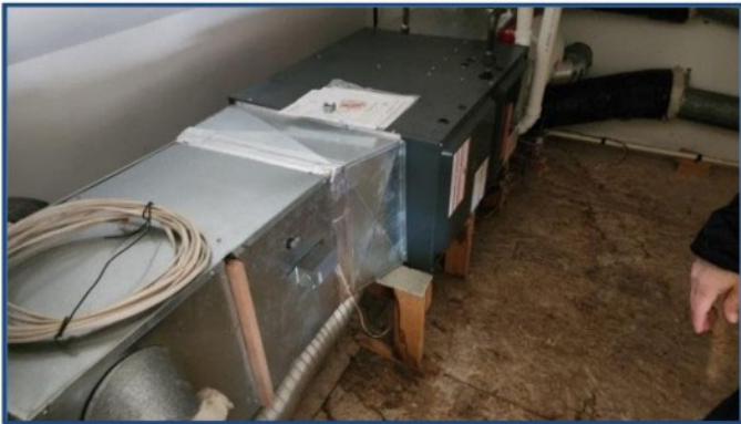
Attic Furnace Servicing Second Floor
