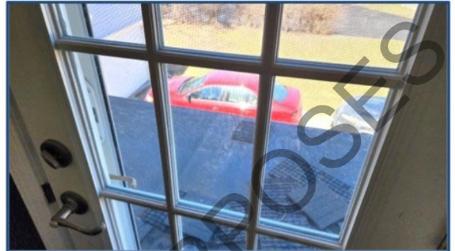
Second Floor Bedroom 2 - Balcony Without Railings
