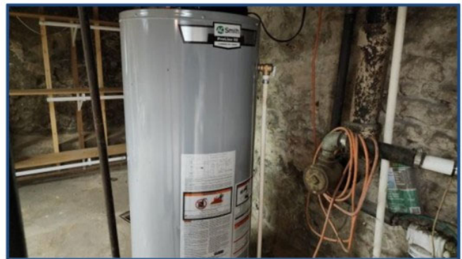
Basement Water Heater
