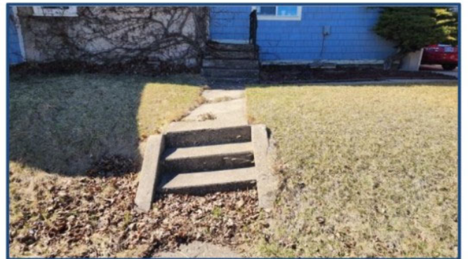
Damaged Concrete at East Elevation
