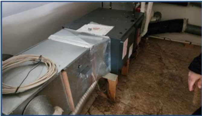
Attic Furnace Servicing Second Floor
