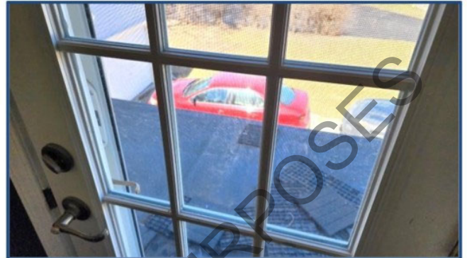
Second Floor Bedroom 2 - Balcony Without Railings
