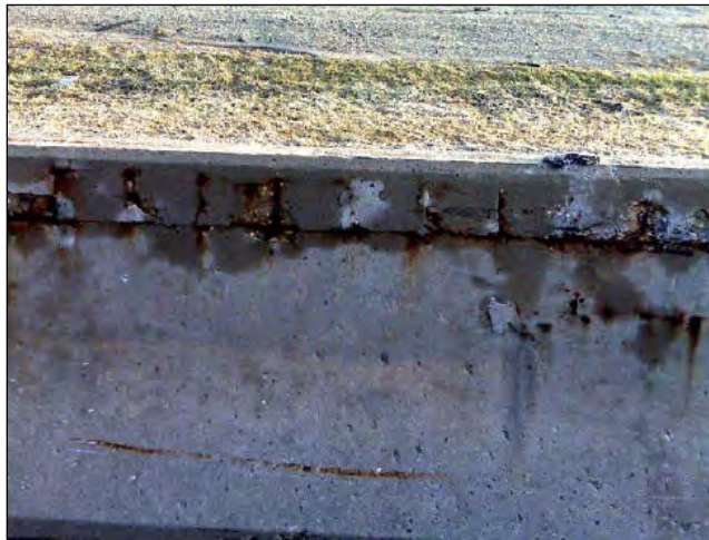
FIGURE 145-10 Exposed Steel Reinforcement
