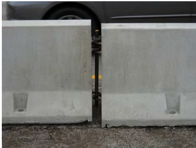
FIGURE 145-22 Improper Connection of 12.5' Temporary Barrier
