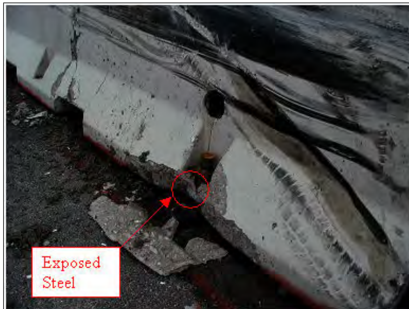
FIGURE 145-8 Anchor Hole Damage
