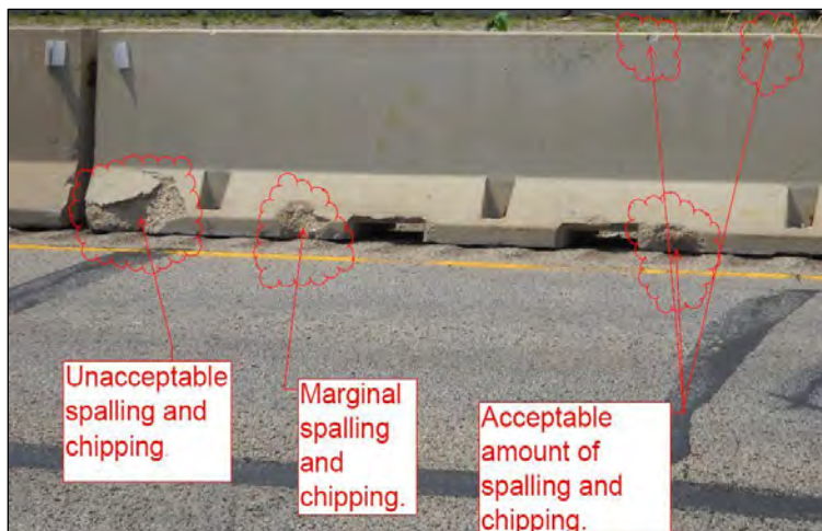
FIGURE 145-12 Unacceptable Chipping and Spalling
