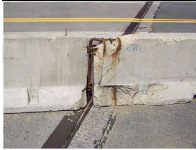
FIGURE 145-7 Exposed Steel and Section Loss Near End Section
