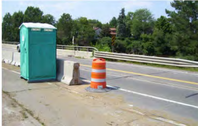
FIGURE 145-19 Improper Termination of Barrier and Object within Deflection Distance
