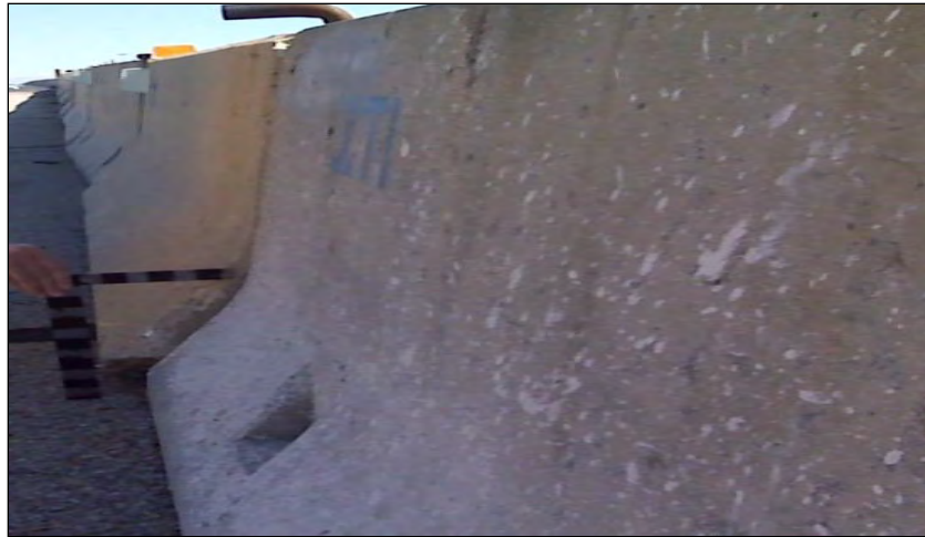
FIGURE 145-16 Potential Snag Point Caused by Different Barrier Styles Not Matching Up
