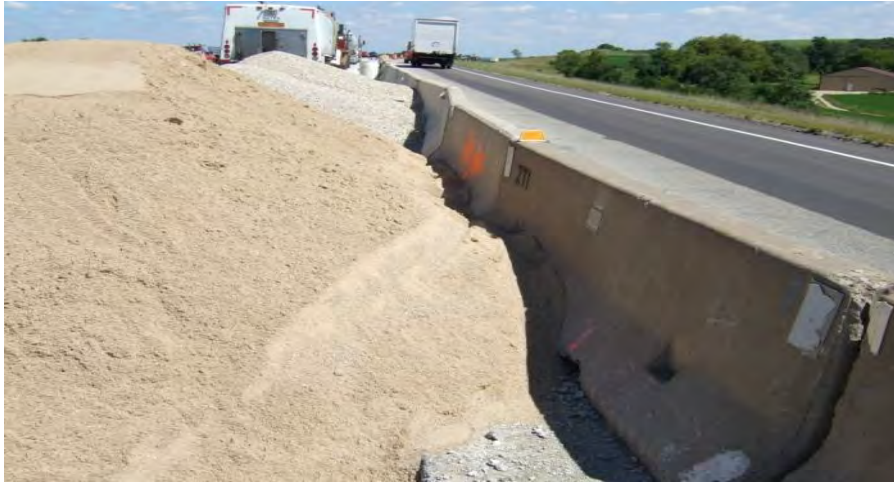
FIGURE 145-21 Insufficient Clearance Behind Temporary Barrier
