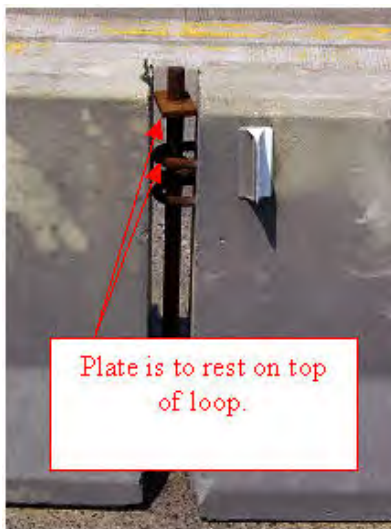
FIGURE 145-3 Improperly Connected Barrier
