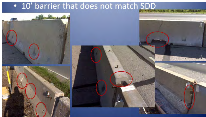
FIGURE 145-23 Barrier Not Matching Standard Details
