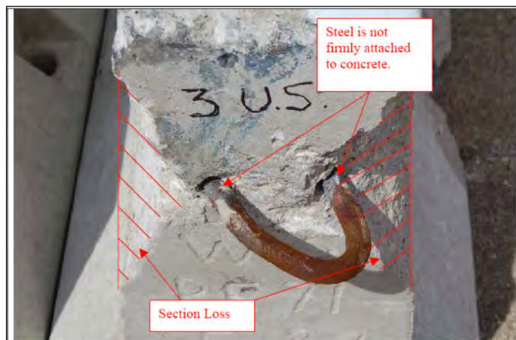
FIGURE 145-6 Loop Not Firmly Connected to Barrier
