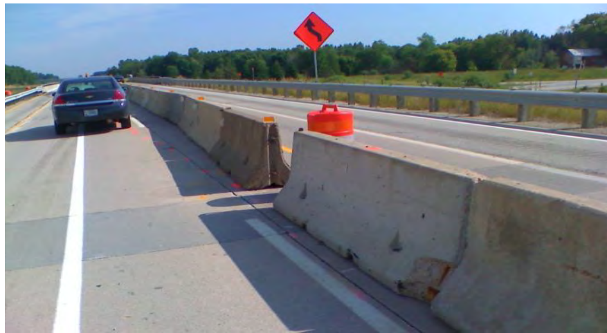
FIGURE 145-20 Gap in Barrier
