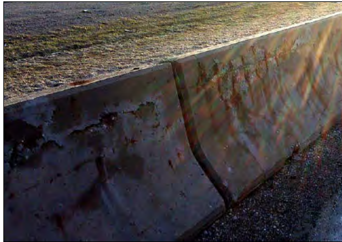
FIGURE 145-11 Exposed Steel Reinforcement
