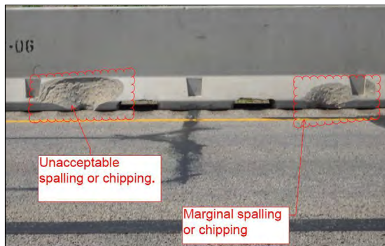
FIGURE 145-15 Chipping and Spalling
