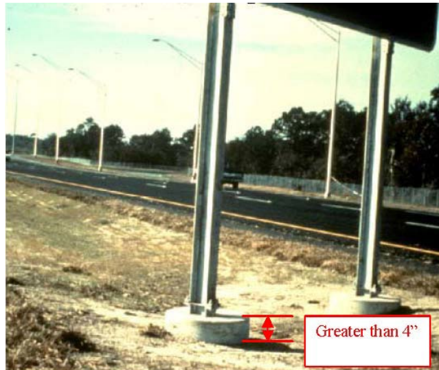
Figure 25.4 Improperly Installed Concrete Footing 3
