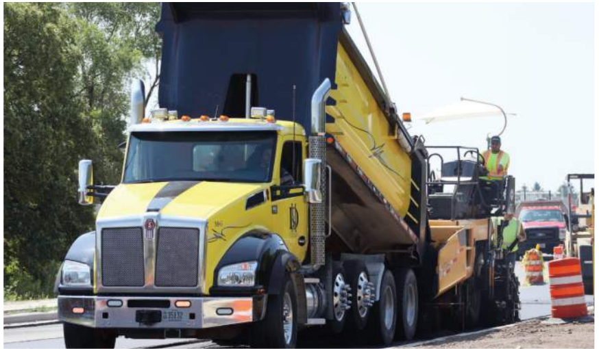
Milwaukee County / I-43 & County Line Road DMS Transportation, LLC
