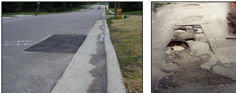
Figure 5: Both patches improperly backfilled/compacted, and not patched to nearest joint or seam
