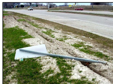
Figure 1: Improper Sign Removal
