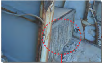
Heavy Concrete Deterioration with Exposed Rebar
