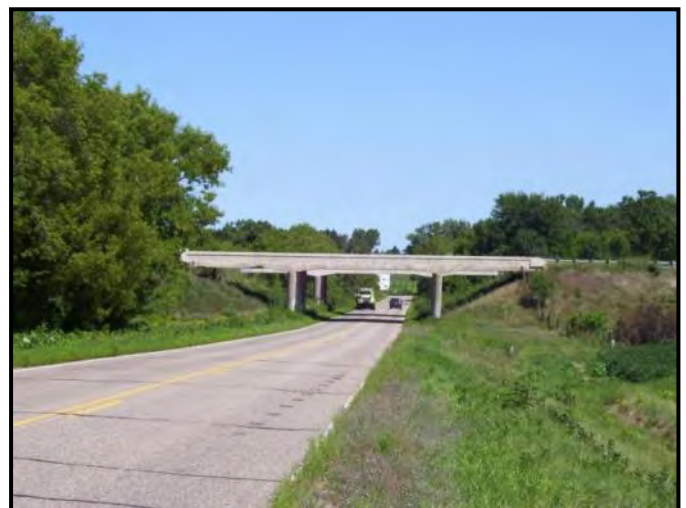
Figure 16 – Width Restriction on Local Road at Piers
