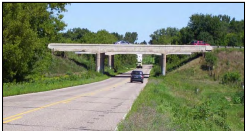
Figure 5 - Deteriorating I-94 bridge over 100 th Street
