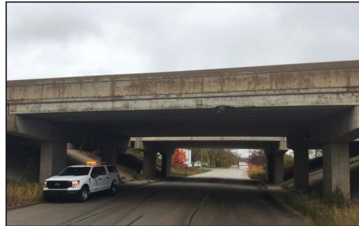
Bridge condition: Deck deterioration occurs along the corridor.
