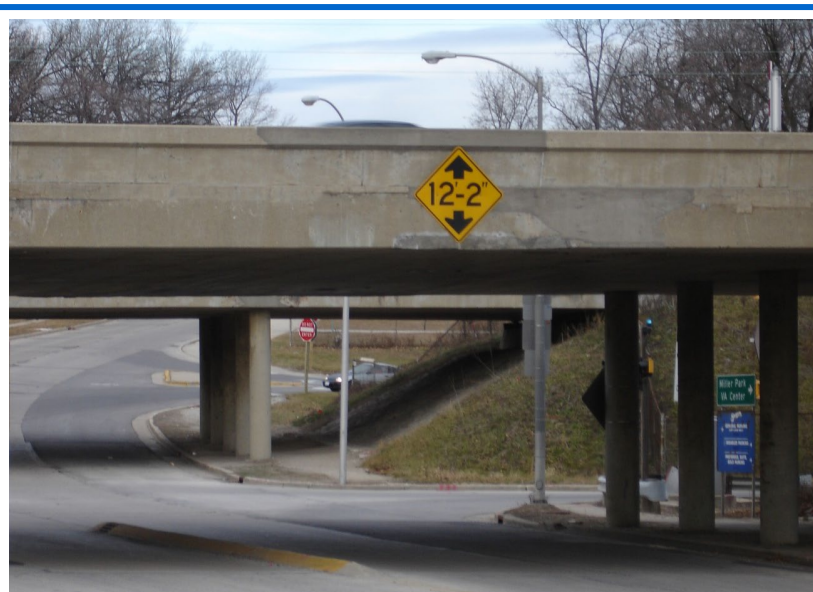
I-94 westbound bridge over General Mitchell Boulevard. Due to the low clearance of this bridge, several trucks have crashed into the underside of the bridge and become stuck. The incidents have contributed to the deterioration of the bridge.
