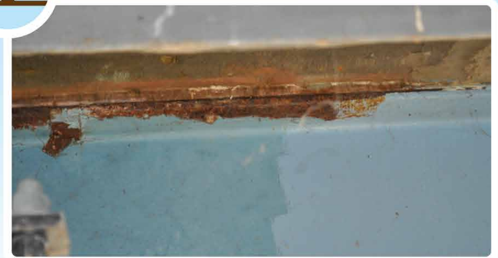
Pack rust has formed between steel elements causing bulging and distortion, leading to added stress and cracking in the concrete deck.
