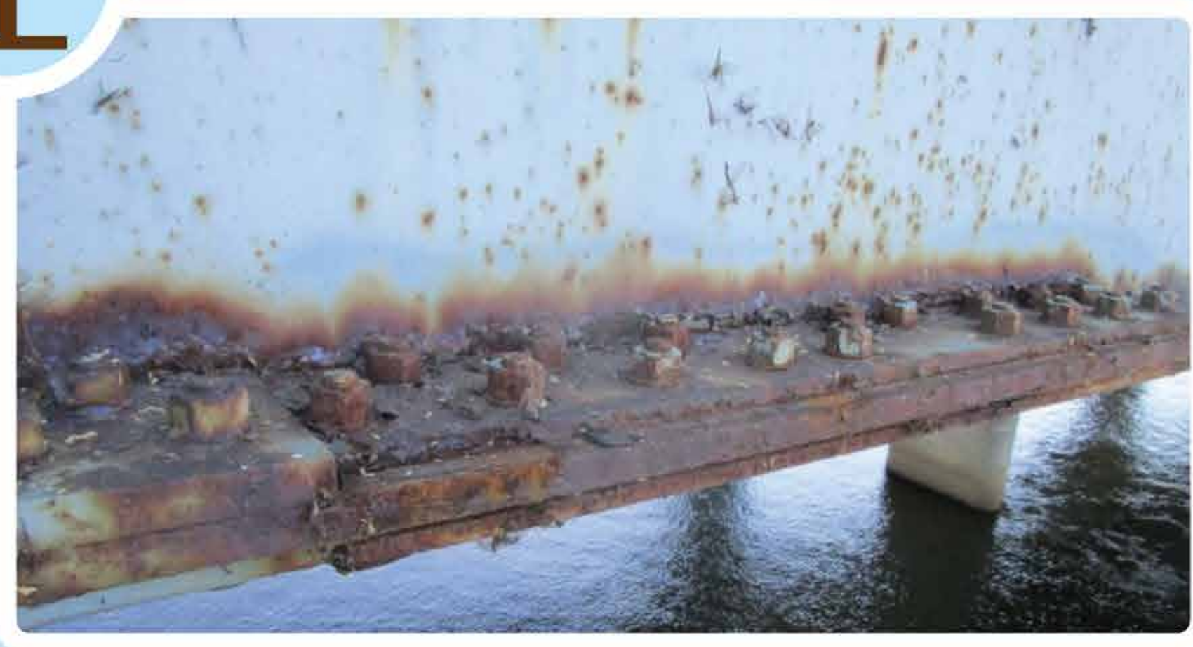
Loss of protective coating over steel elements and connections.
