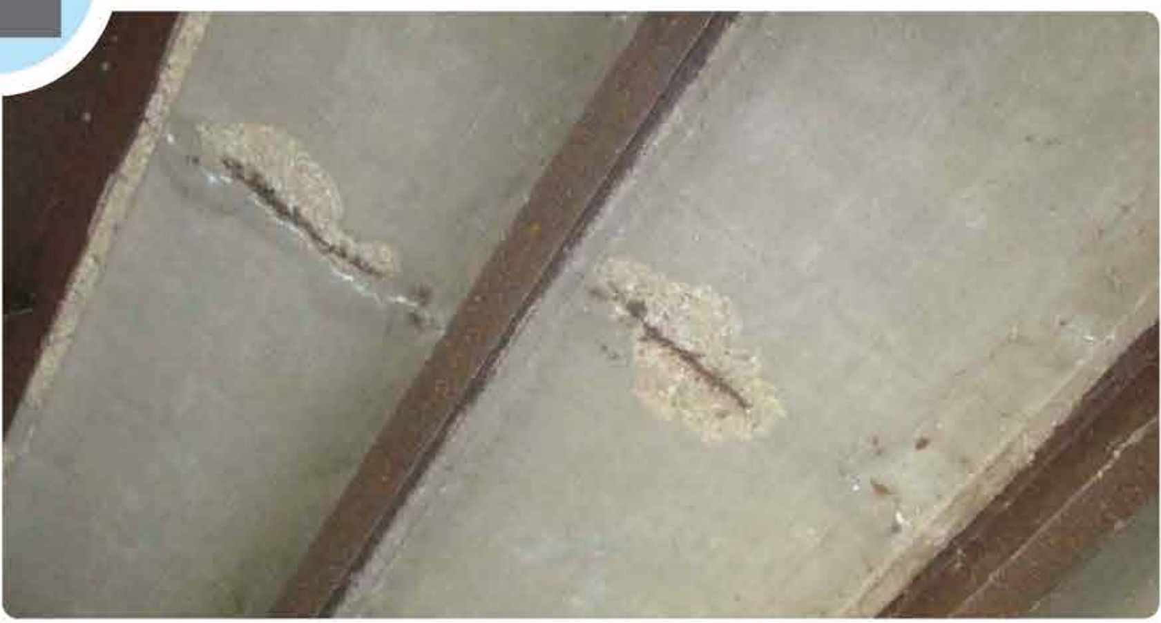
Concrete on the bottom of the bridge deck is cracking and chipping off, exposing the reinforcing steel.
