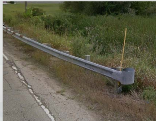
Existing end of guardrail on WIS 113
