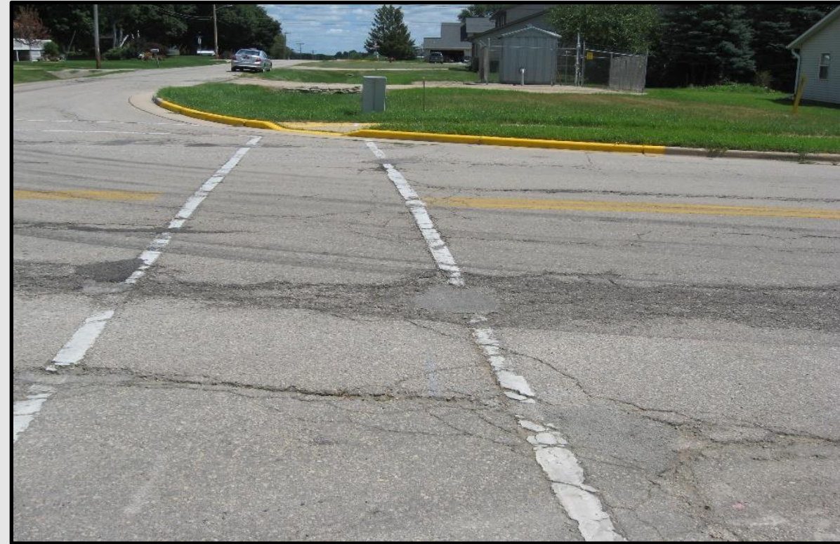
Example of rutting and alligator cracking on WIS 73
