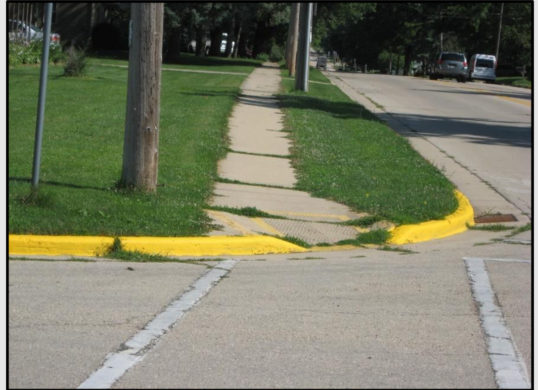
Example of non-compliant curb ramp on WIS 73
