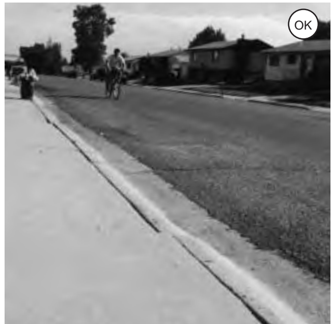
Figure 2-12 (top): A rough edge created by not feathering the overlay into the curb.
