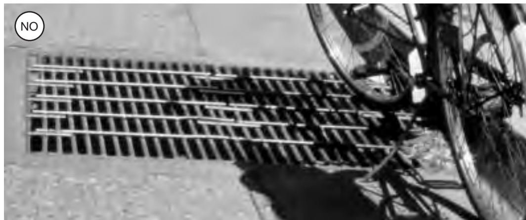
Figure 2-21: Temporary measures, like welded straps, may be more costly in the long run.
