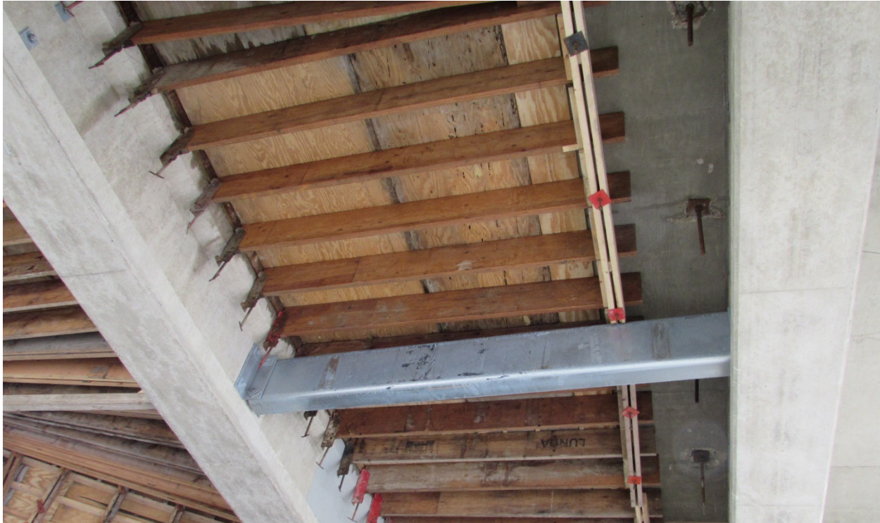
Figure 7.9 - Formwork system as seen in staged construction of bridge B-64-123. Wood beams are supported by top flange of left girder and rods are drilled through Stage 1 hardened deck on right side.
