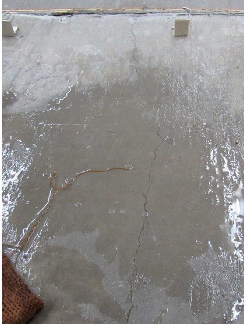
Figure 7.29 - Flexural crack resulting from deflections applied during curing of Stage 2 segment.
