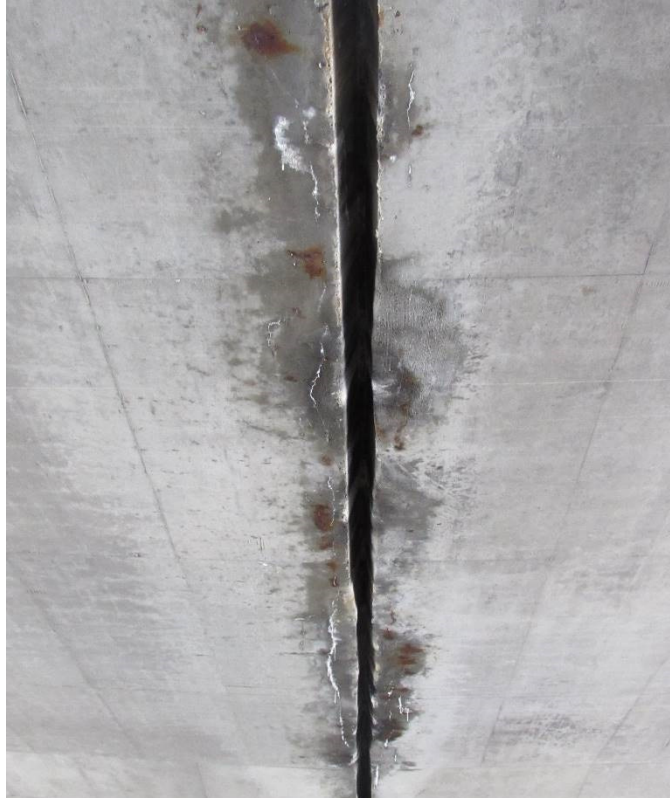
Figure 4.13 - Efflorescence and corrosion due to retained moisture at waterstop joint between adjacent bridges. (B-30-025/026)
