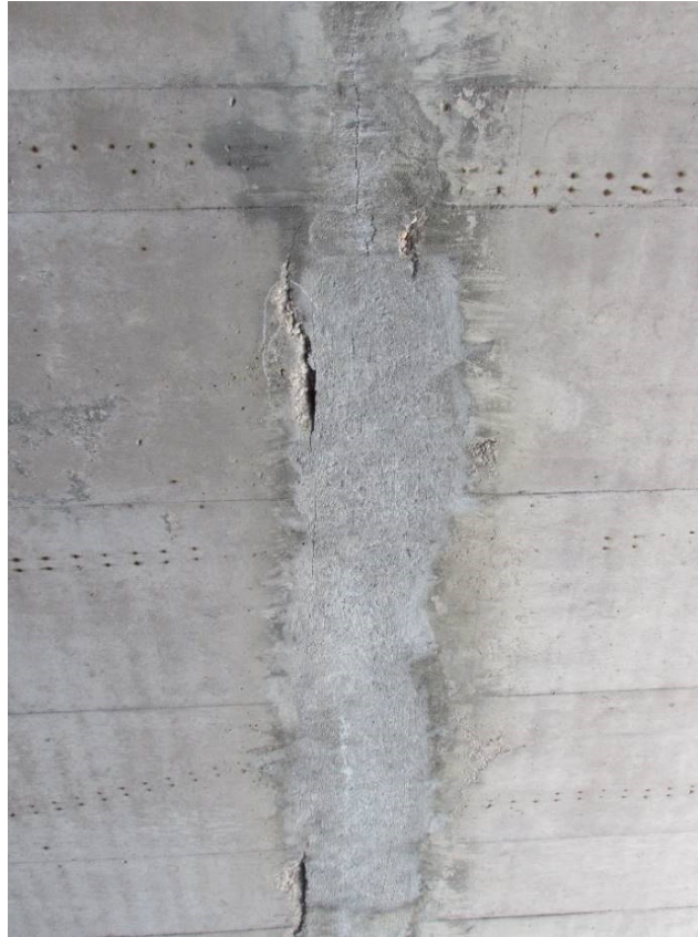
Figure 4.9- Patching of previously spalled concrete at longitudinal construction joint in haunched slab bridge. (B-30-026)
