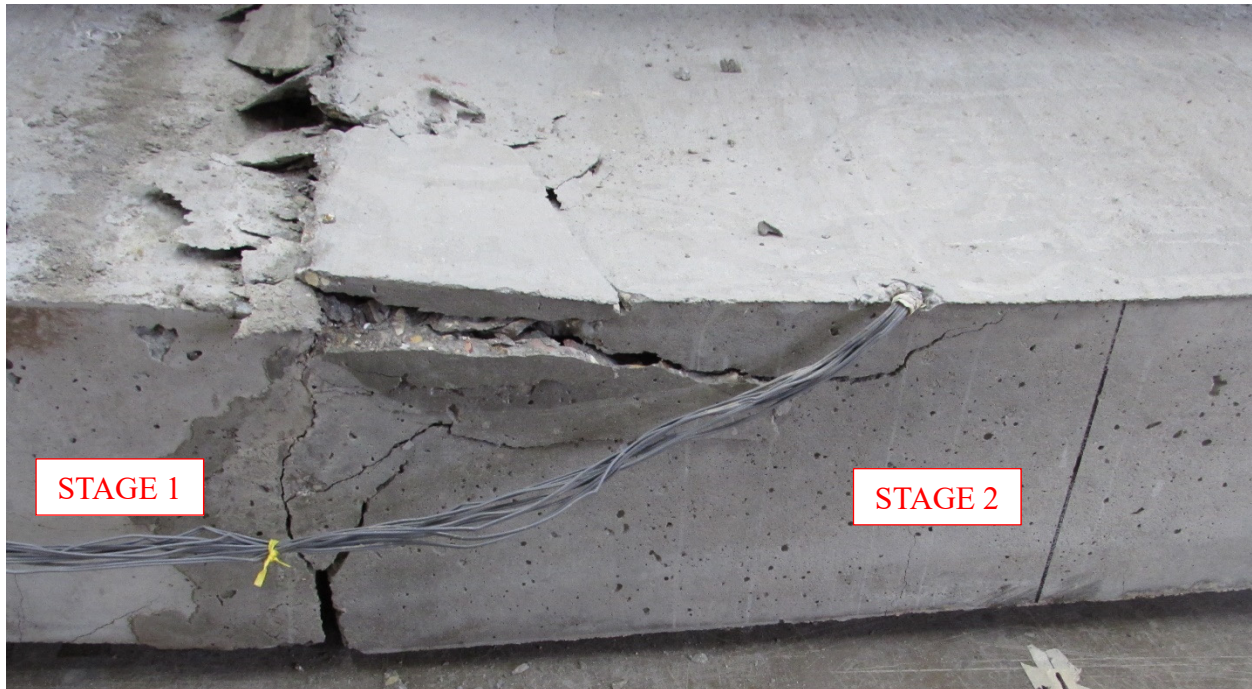
Figure 7.31 - Specimen 2 compression block failure at construction joint.
