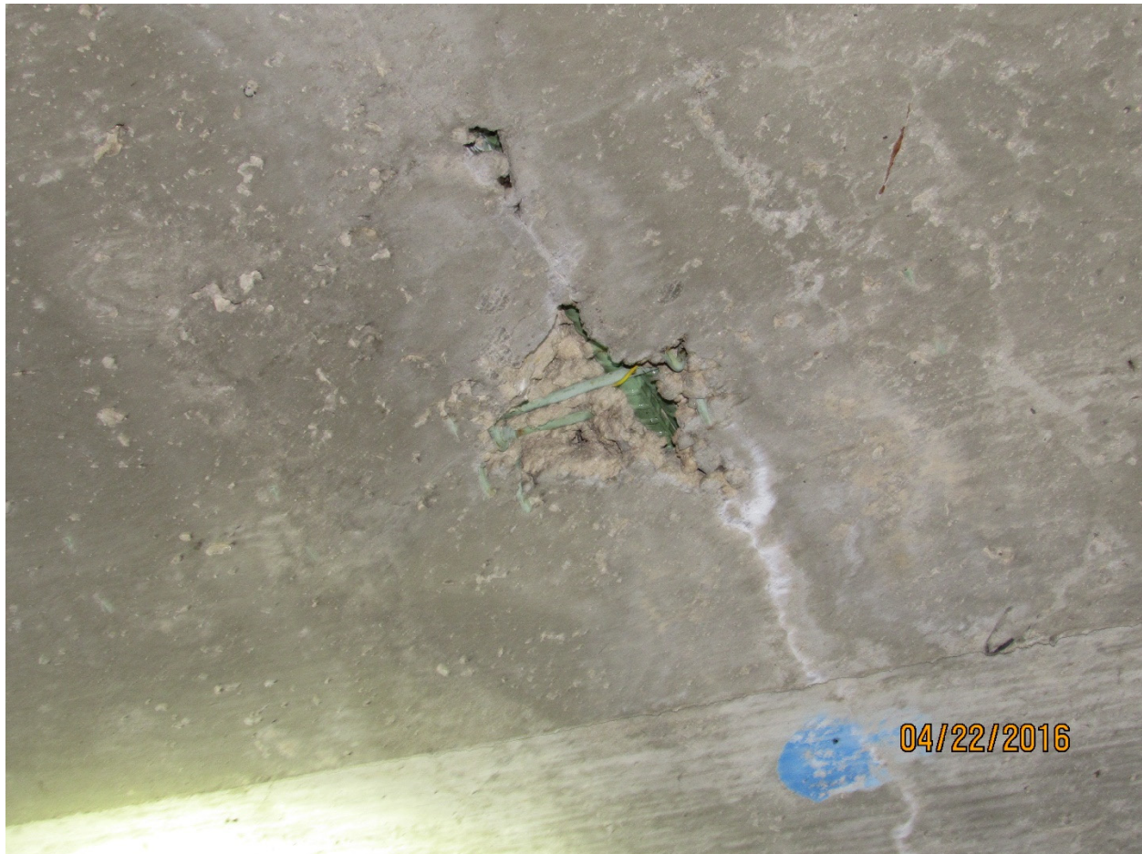
Figure 4.2- Inadequate concrete consolidation exposing reinforcement in the longitudinal joint region. (B-40-216 – Dowel bar splicer, detail B per Figure 4.1)
