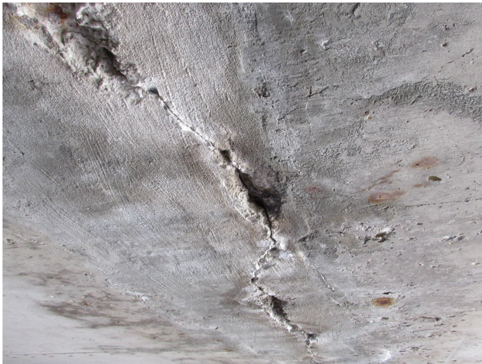
Figure 4.14 - Large longitudinal crack opening approximately 1/4" during the passage of large trucks. (B-30-015)
