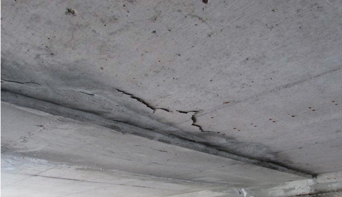
Figure 4.12 - Delaminated area adjacent to longitudinal construction joint in widened portion of deck. (B-30-014)
