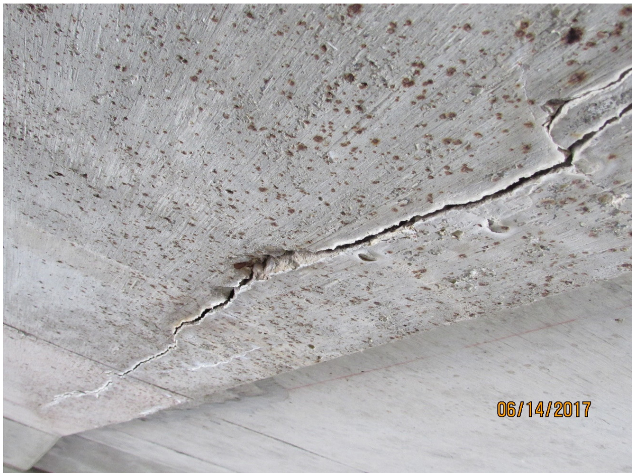
Figure 4.11- Large longitudinal crack adjacent to construction joint. (B-51-017)
