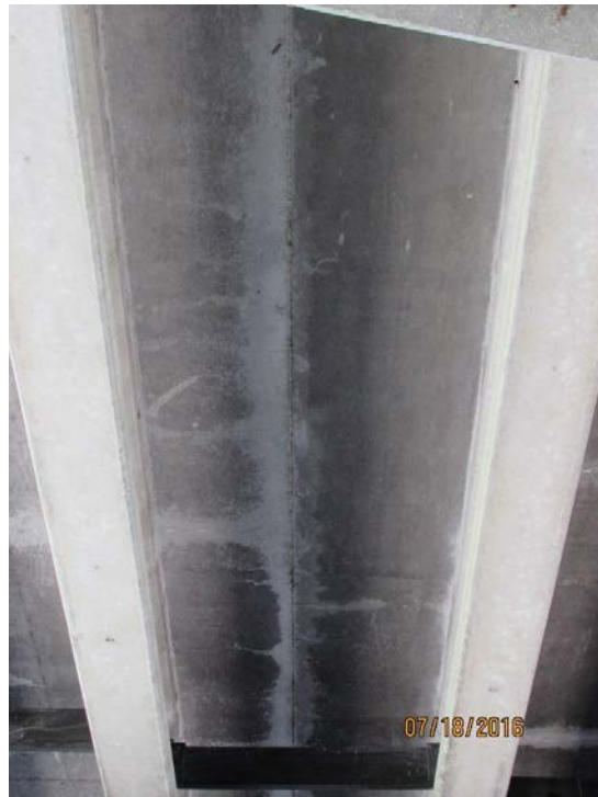
Figure 4.4 - Typical leakage through a longitudinal construction joint (B-53-083)
