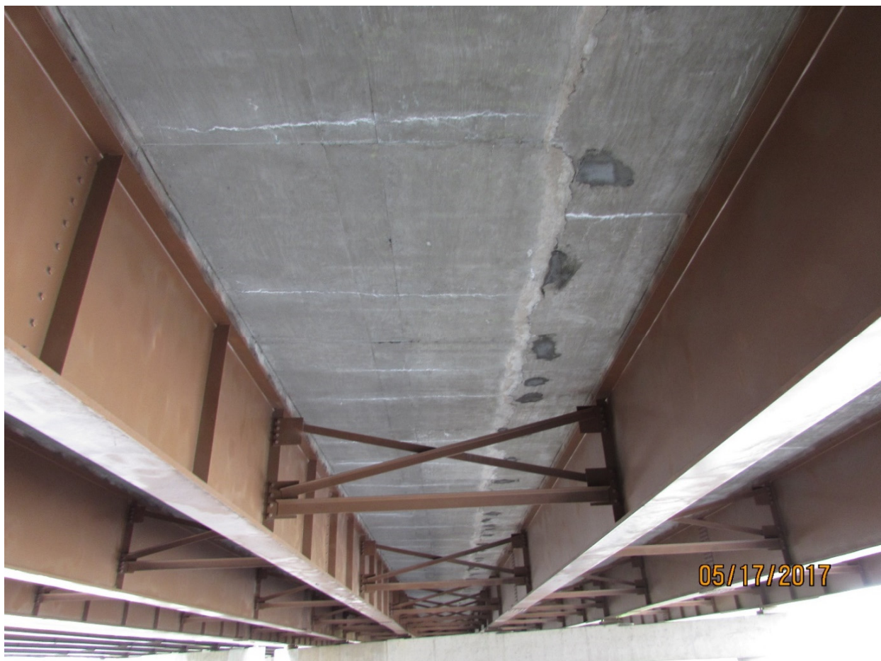
Figure 4.3- Typical regularly spaced transverse cracks with efflorescence (B-70-176)
