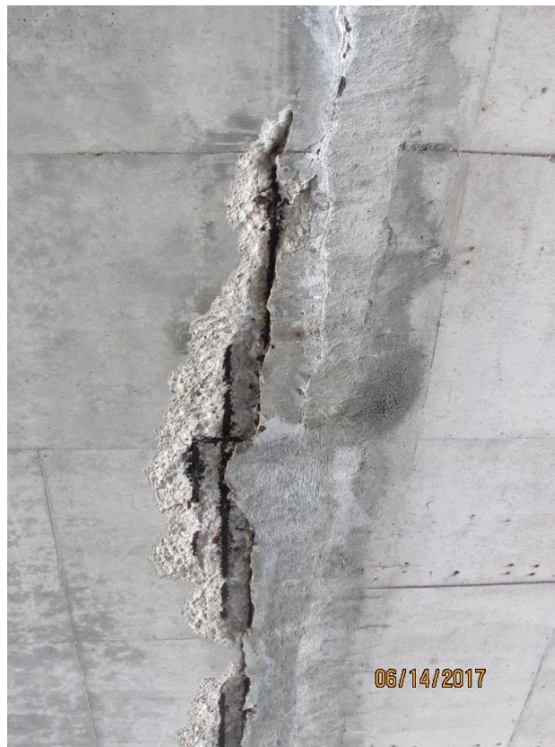
Figure 4.10- Spalled concrete at longitudinal construction joint exposing corroded reinforcement. (B-30-014)
