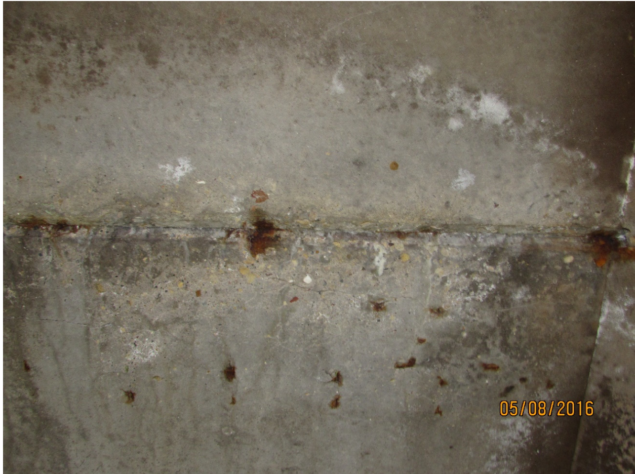
Figure 4.6 - Typical spots of corrosion on the underside of the longitudinal construction joint (B-56-022)
