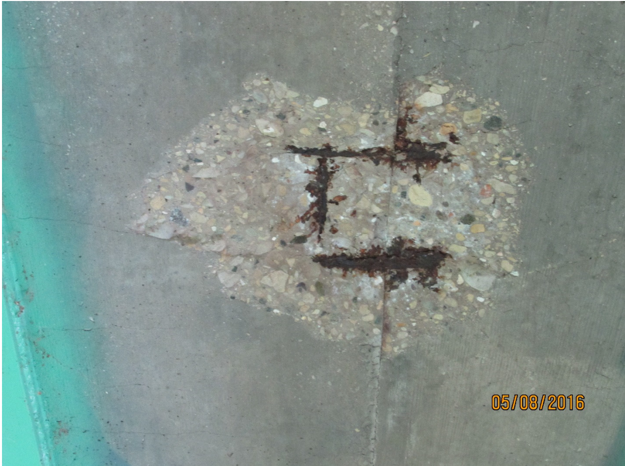
Figure 4.7- Spalled concrete and corroded reinforcement. Transverse cracking at approx. same spacing as transverse reinforcement (B-13-593)
