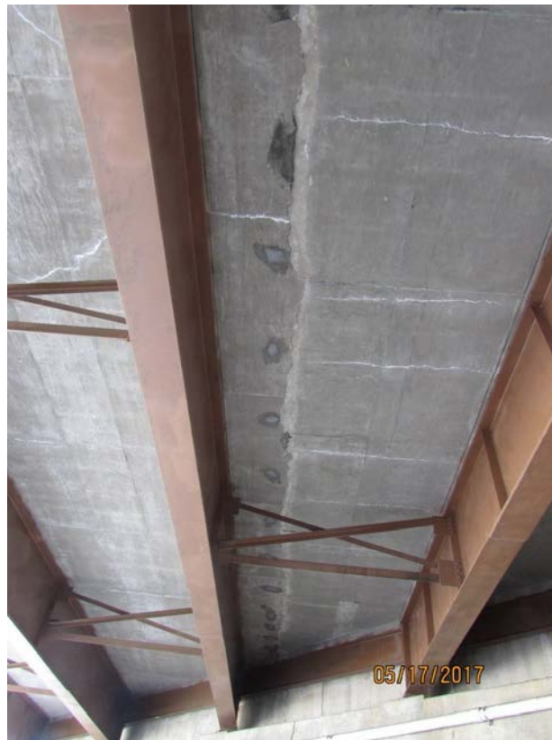
Figure 4.8- Transverse cracks extending to abutment in Stage 2 deck (right side). Transverse cracks in Stage 1 deck (left side) only near midspan region. (B-70-176)
