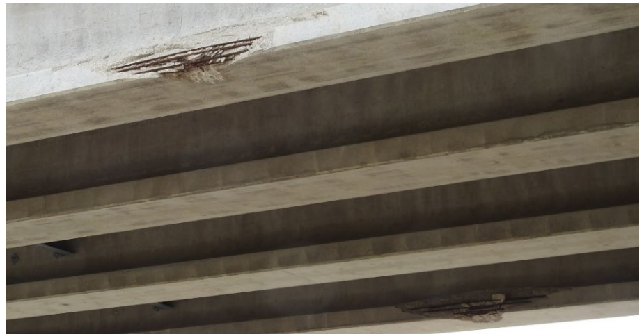
Initial-impact (top left) and rebound-impact (bottom right) damage
