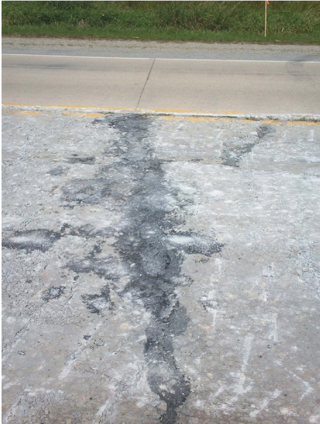
Figure 15. Joint in poor condition after rubblization
