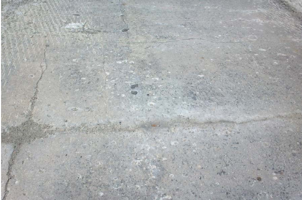
Figure 13. Crack in good condition
