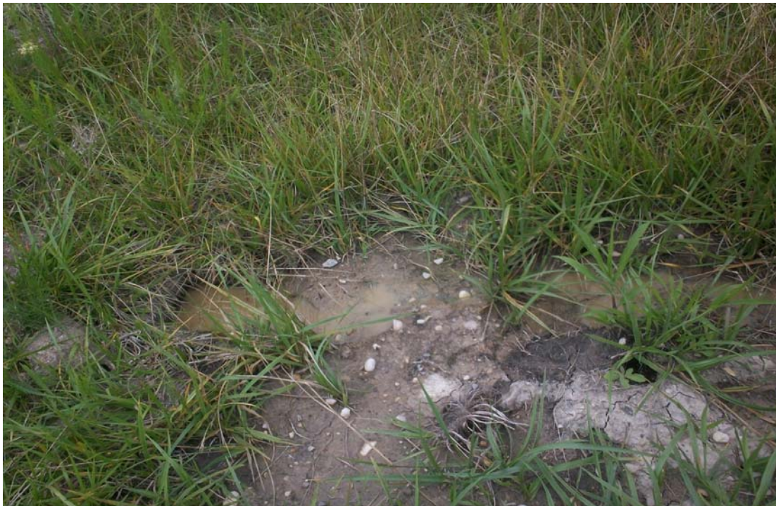
Figure 35. Condition of existing edge drain on I-43
