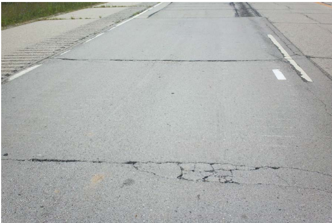
Figure 11. Reflection crack in HMA overlay on I-43 in poor condition
