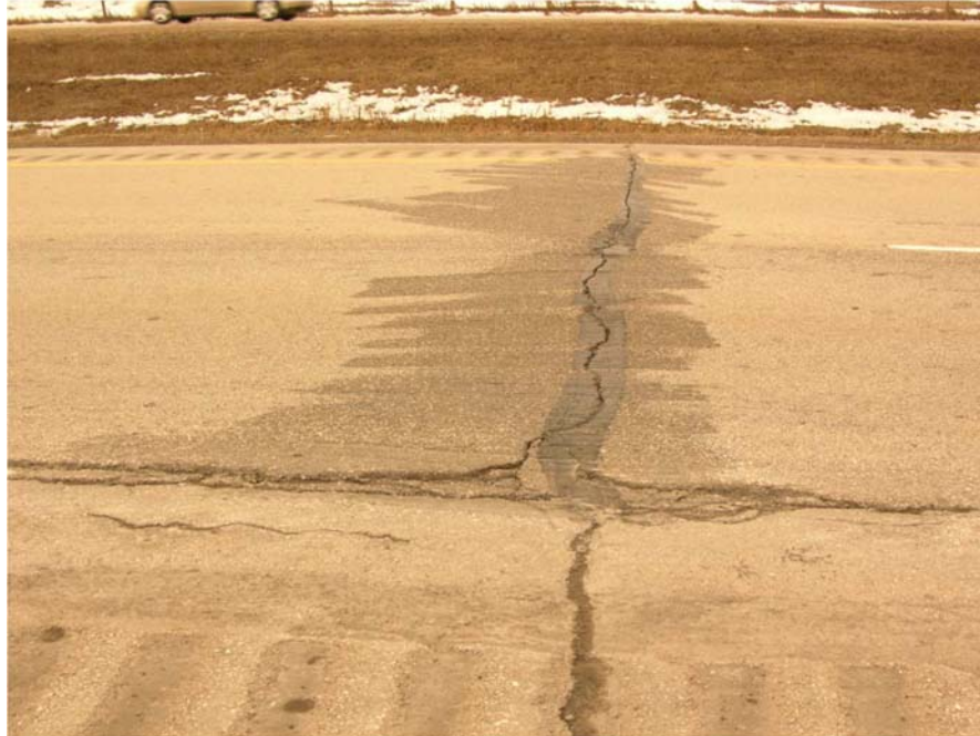
Figure 2. Tented crack on USH 41, Brown County, Wisconsin (Battaglia and Paye, 2011)
