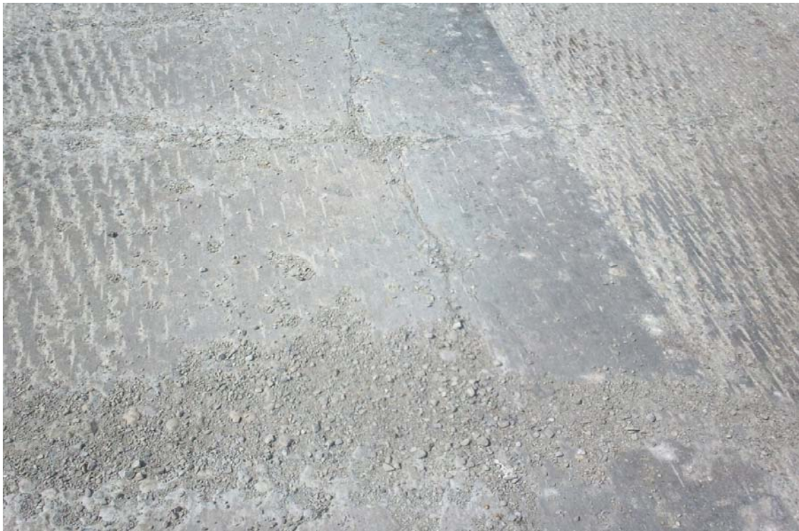
Figure 14. Crack in poor condition
