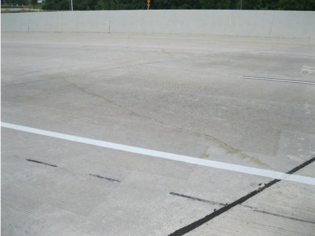
Figure 5-11 B-05-0605 Approach Cracking at Bridge Exit
