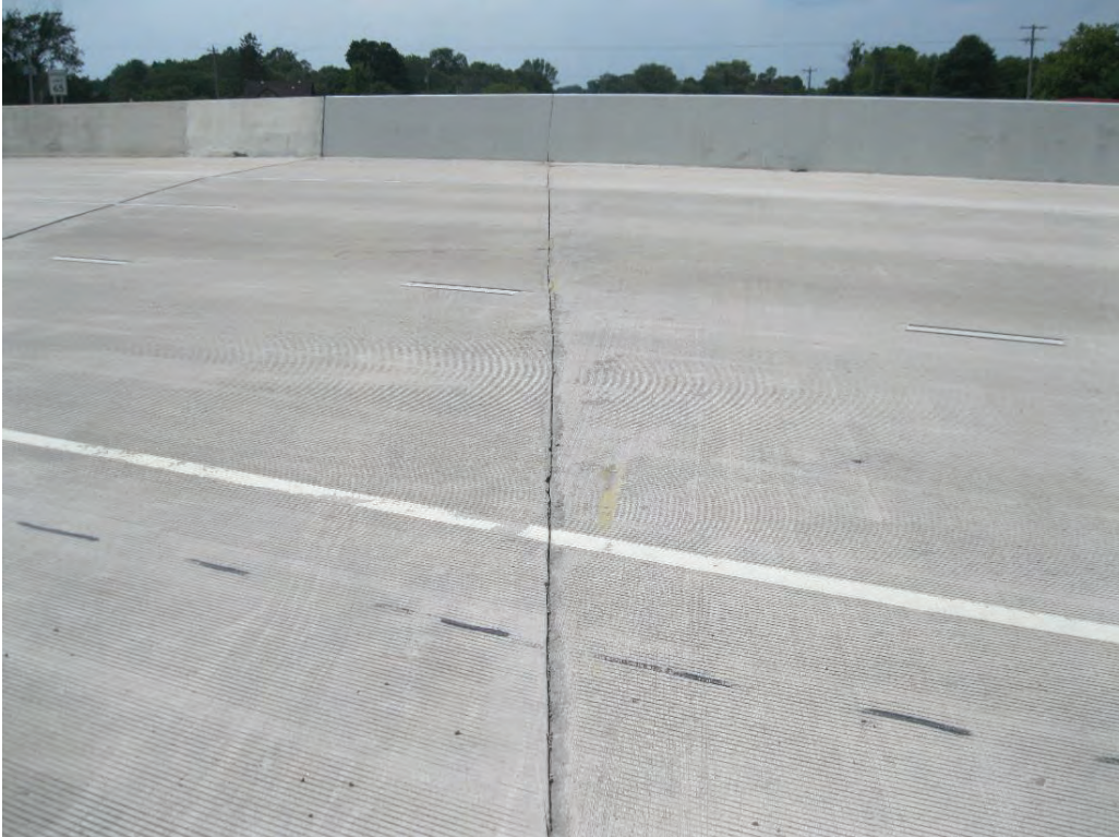
Figure 5-33 B-05-0607 Bridge Deck Scuffing
