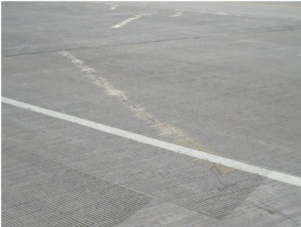
Figure 5-3 B-05-0604 Approach Apron Cracking
