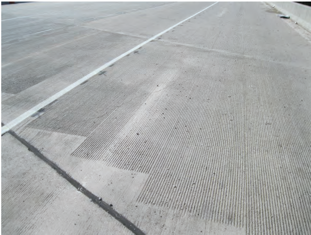
Figure 5-37 B-05-0650 Approach Apron Cracking
