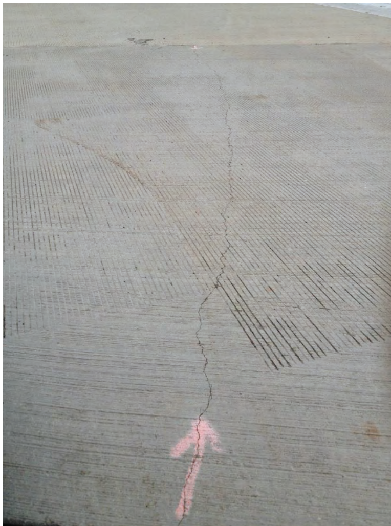
Figure 5-77 Wisconsin Approach Cracking
