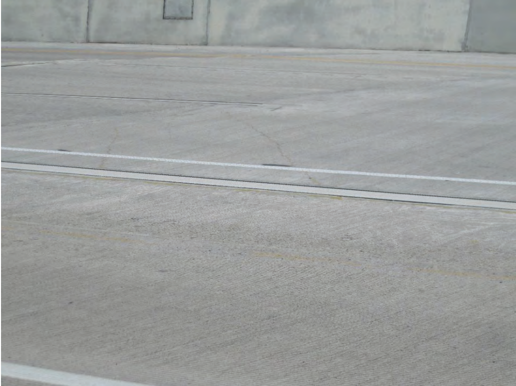
Figure 5-45 B-05-0651 Bridge Deck Cracking
