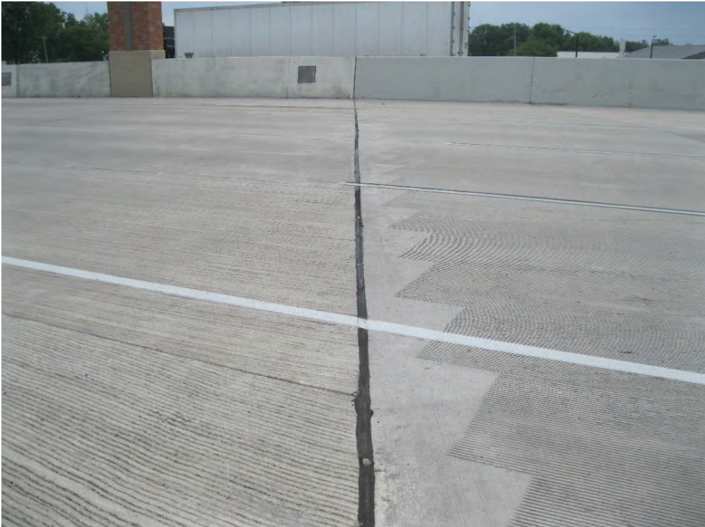
Figure 5-25 B-05-0606 Pavement to Approach Expansion Joint
