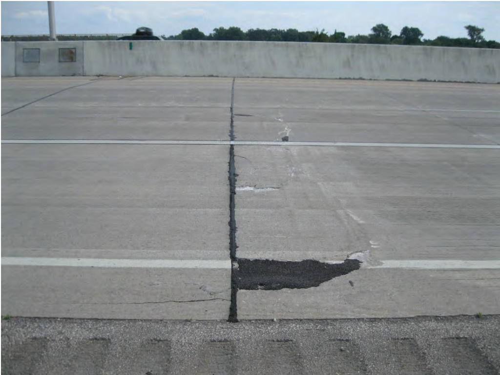
Figure 5-52 B-70-0264 Approach Cracking
