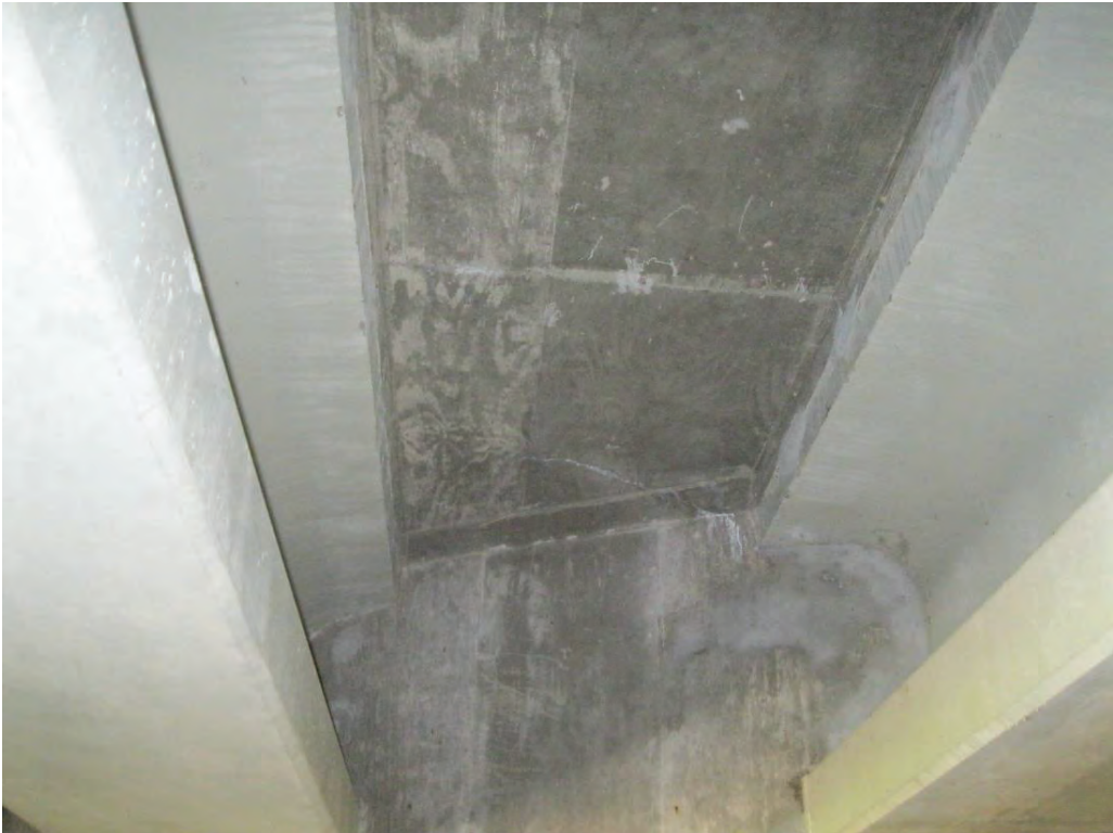
Figure 5-14 B-05-0605 Deck Underside Cracking
