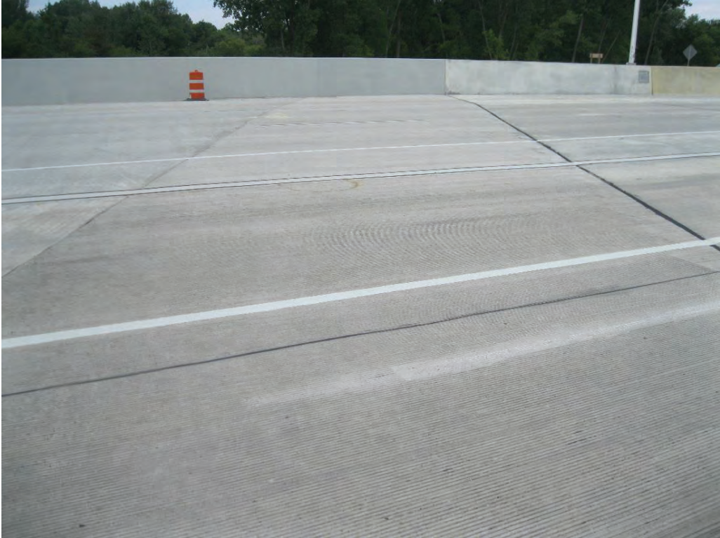
Figure 5-43 B-05-0651 Approach apron cracking
