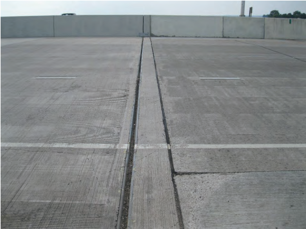
Figure 5-61 B-70-0265 Expansion Joint Debris Build-up
