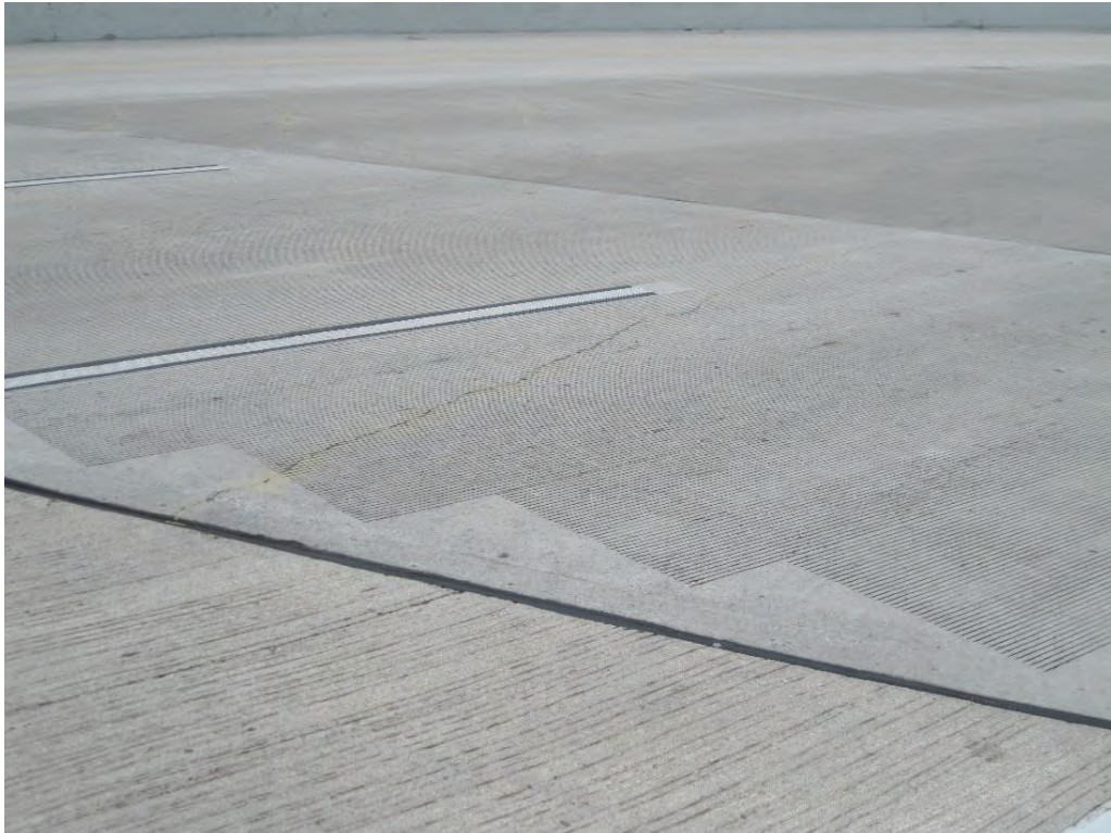
Figure 5-23 B-05-0606 Approach Apron Cracking
