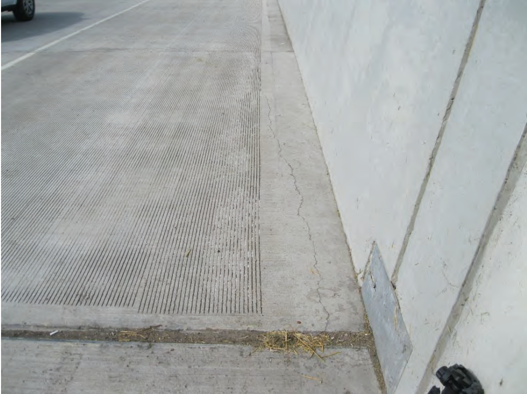
Figure 5-60 B-70-0265 Approach Cracking
