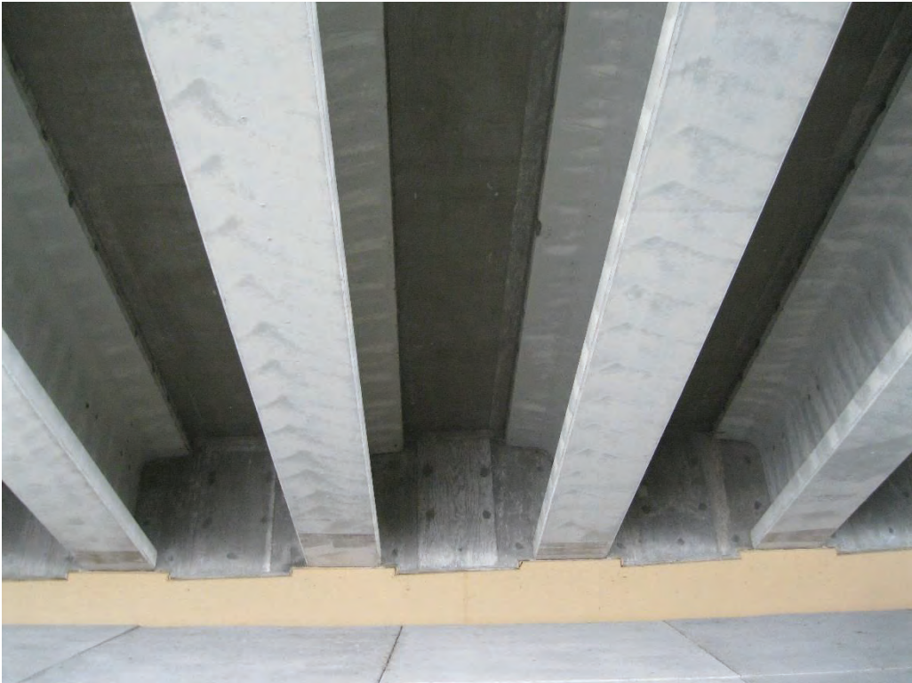
Figure 5-68 B-70-0266 Underside of Deck Condition
