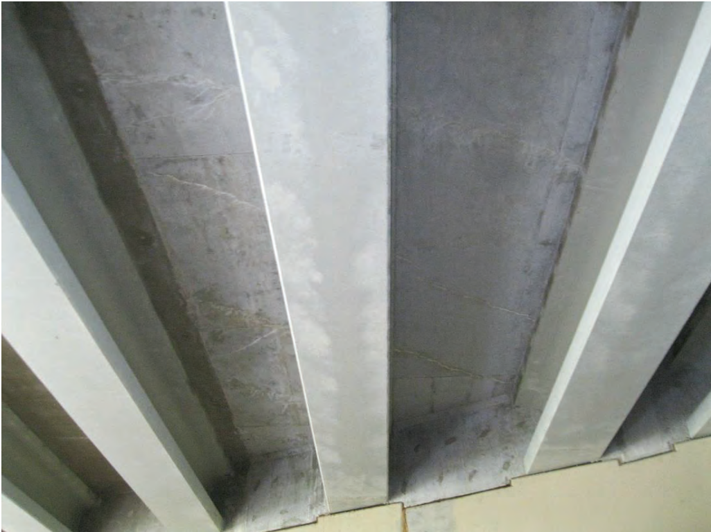
Figure 5-46 B-05-0651 Cracking on Underside of Bridge Deck
