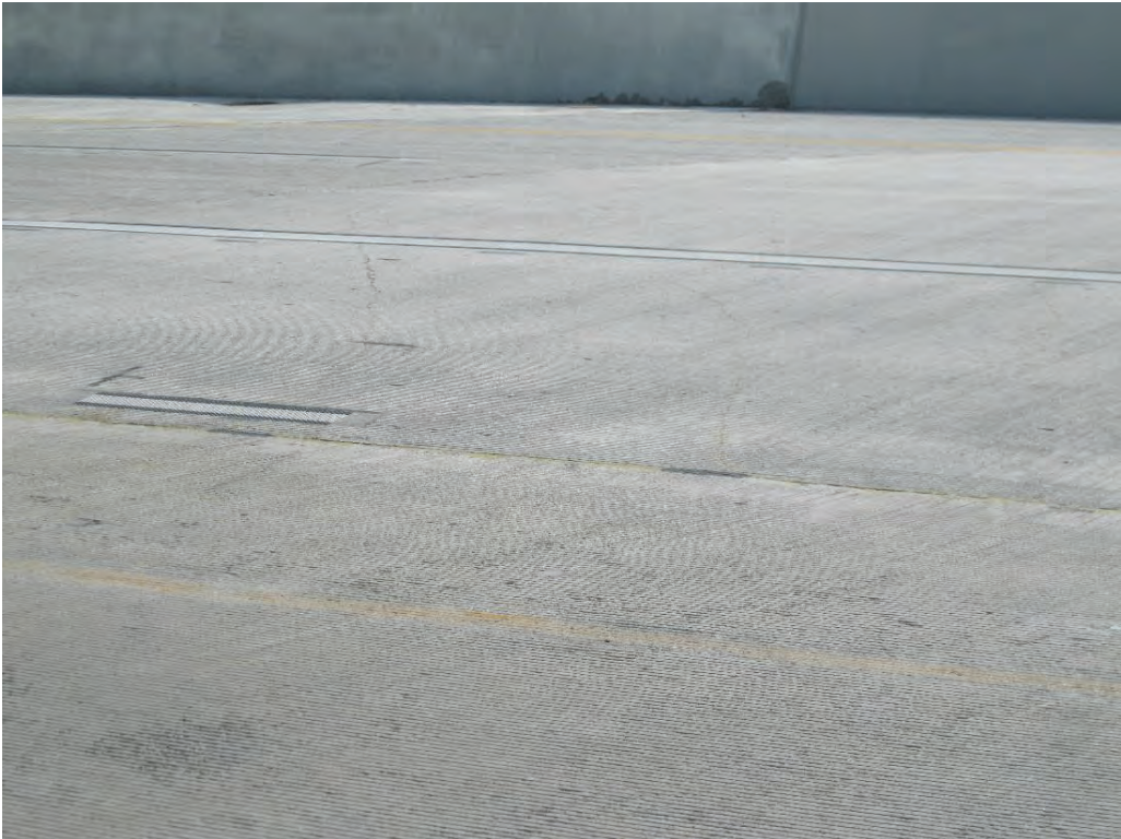
Figure 5-39 B-05-0650 Bridge Deck Cracks
