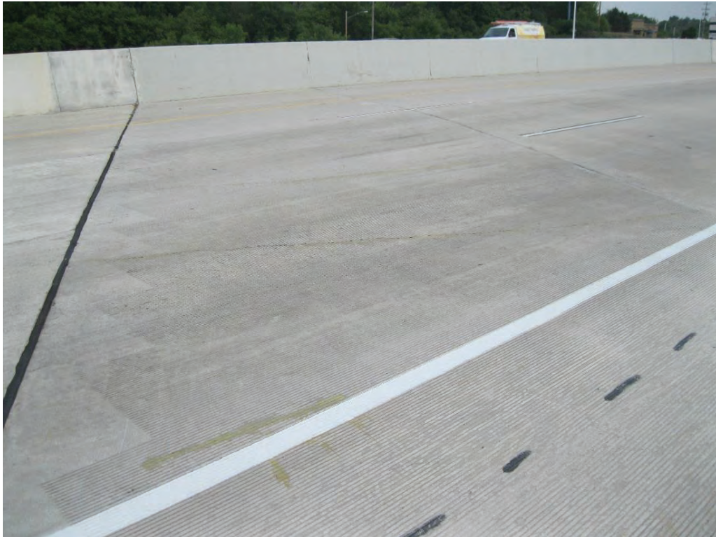
Figure 5-10 B-05-0605 Approach Cracking at Bridge Entrance
