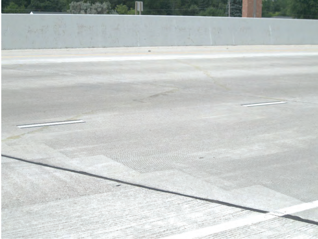
Figure 5-30 B-05-0607 Approach Apron Cracking
