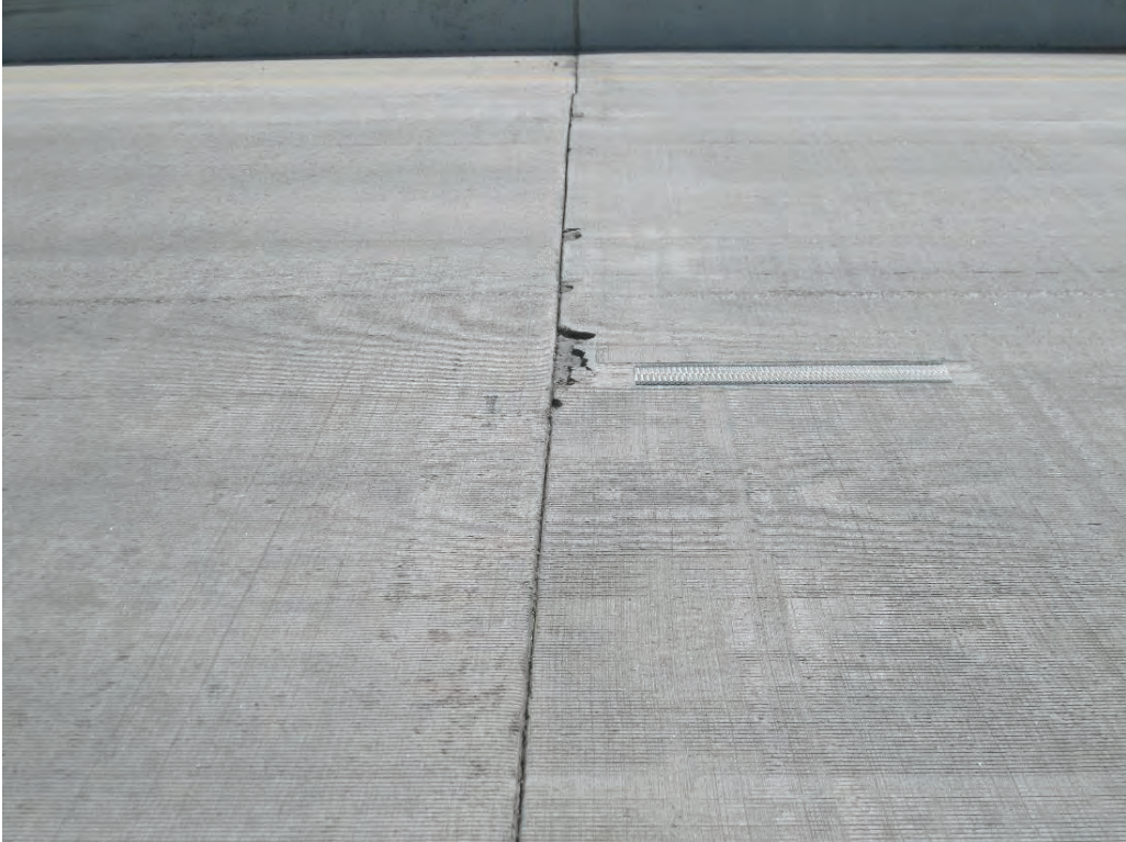
Figure 5-65 B-70-0266 Bridge Deck Joint Spalling
