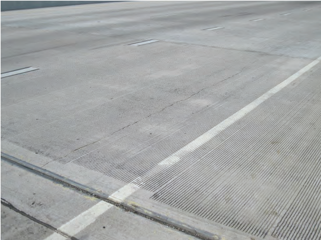
Figure 5-59 B-70-0265 Approach Cracking
