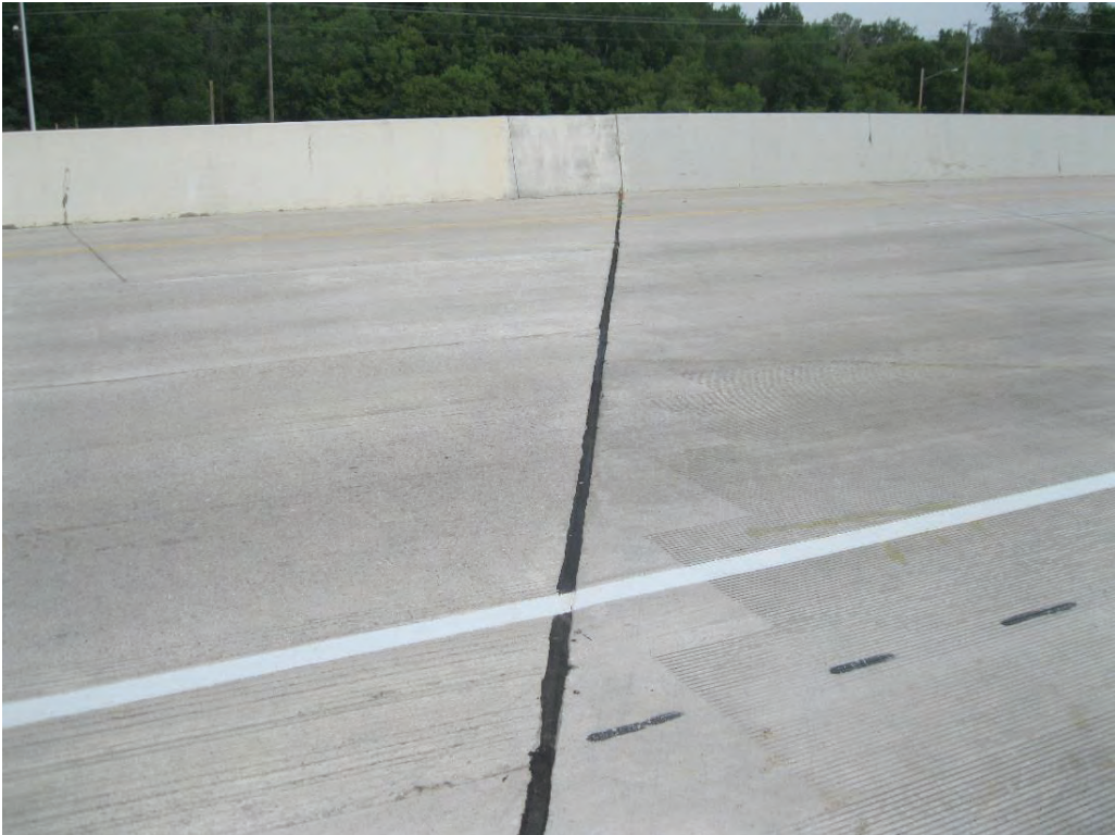
Figure 5-12 B-05-0605 Pavement to Approach Expansion Joint
