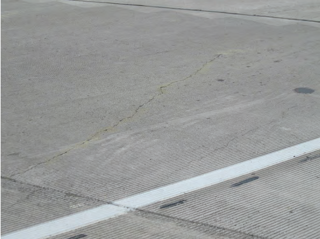
Figure 5-24 B-05-0606 Approach Apron Cracking
