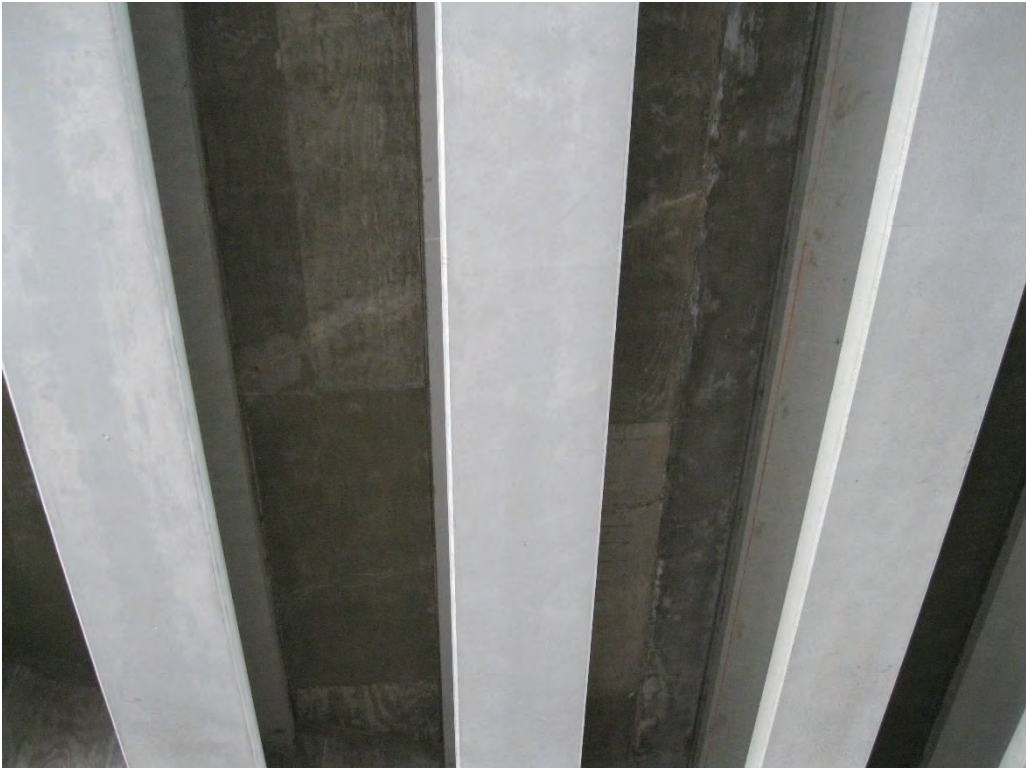
Figure 5-32 B-05-0607 Underside of Deck Cracking
