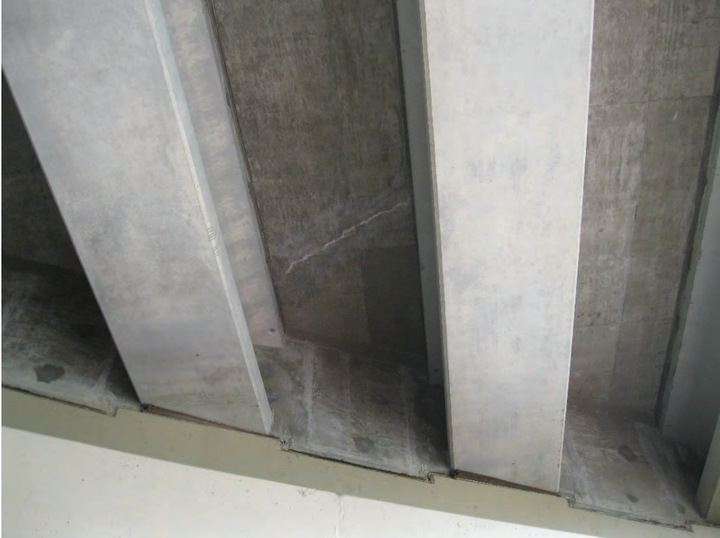
Figure 5-31 B-05-0607 Underside of Deck Cracking
