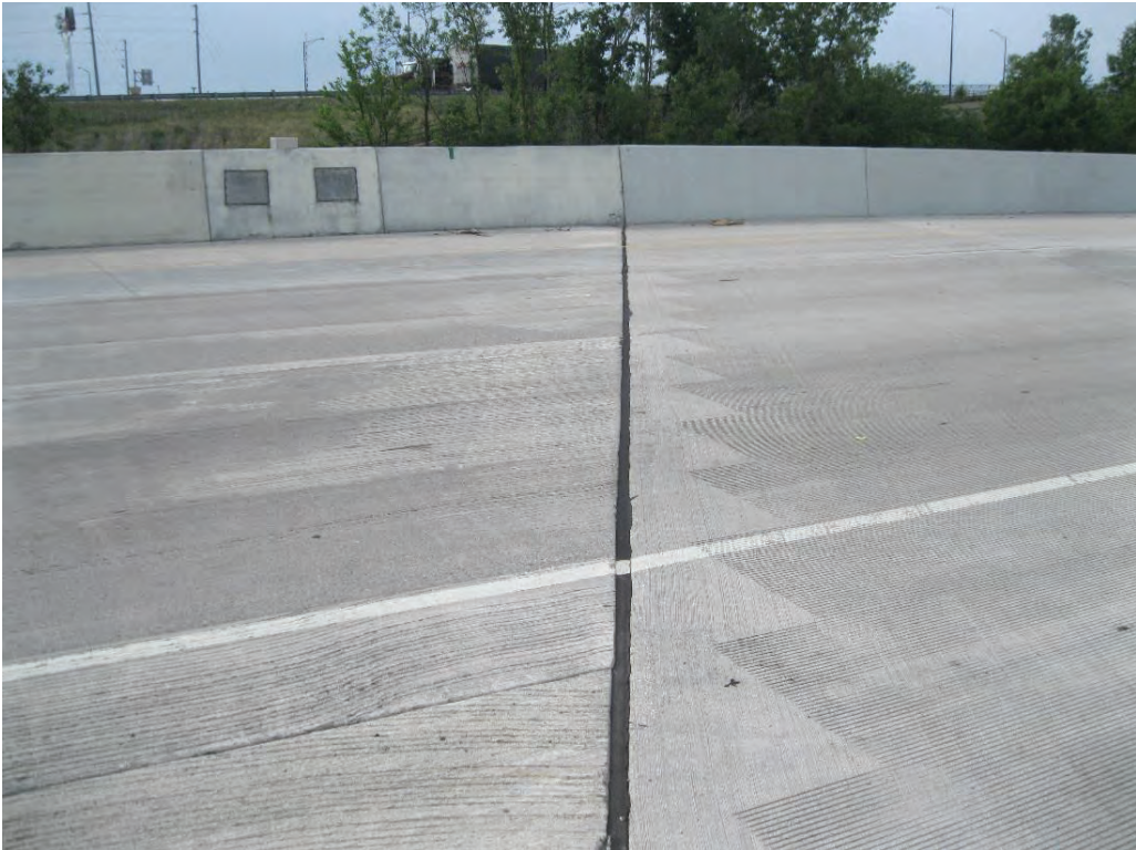
Figure 5-5 B-05-0604 Pavement to Approach Expansion Joint
