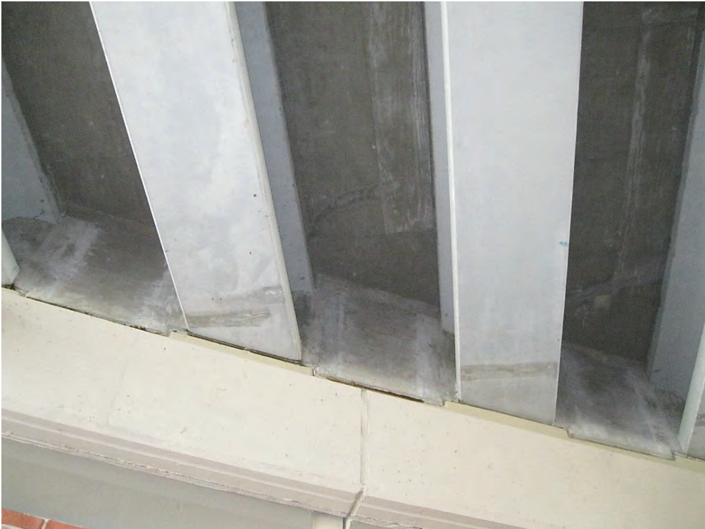
Figure 5-27 B-05-0606 Deck Underside Cracking
