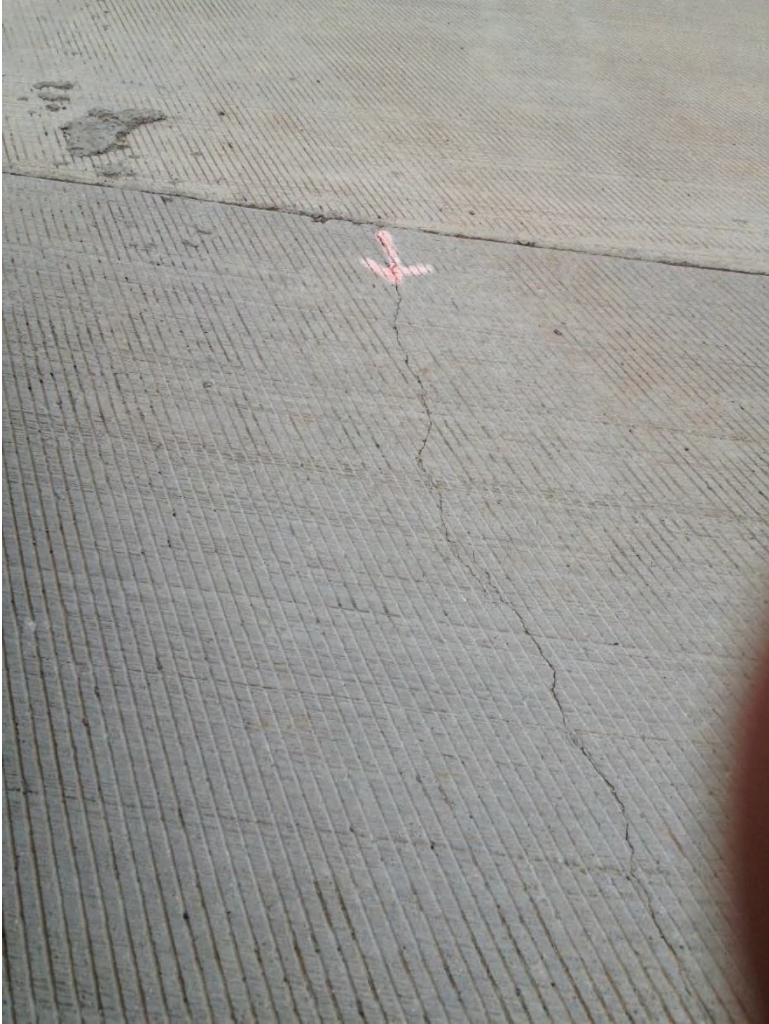
Figure 5-78 Wisconsin Approach Cracking
