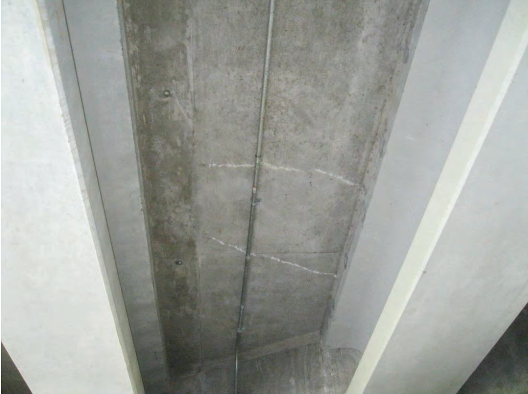
Figure 5-40 B-05-0650 Bridge Deck Cracks Seen from Below
