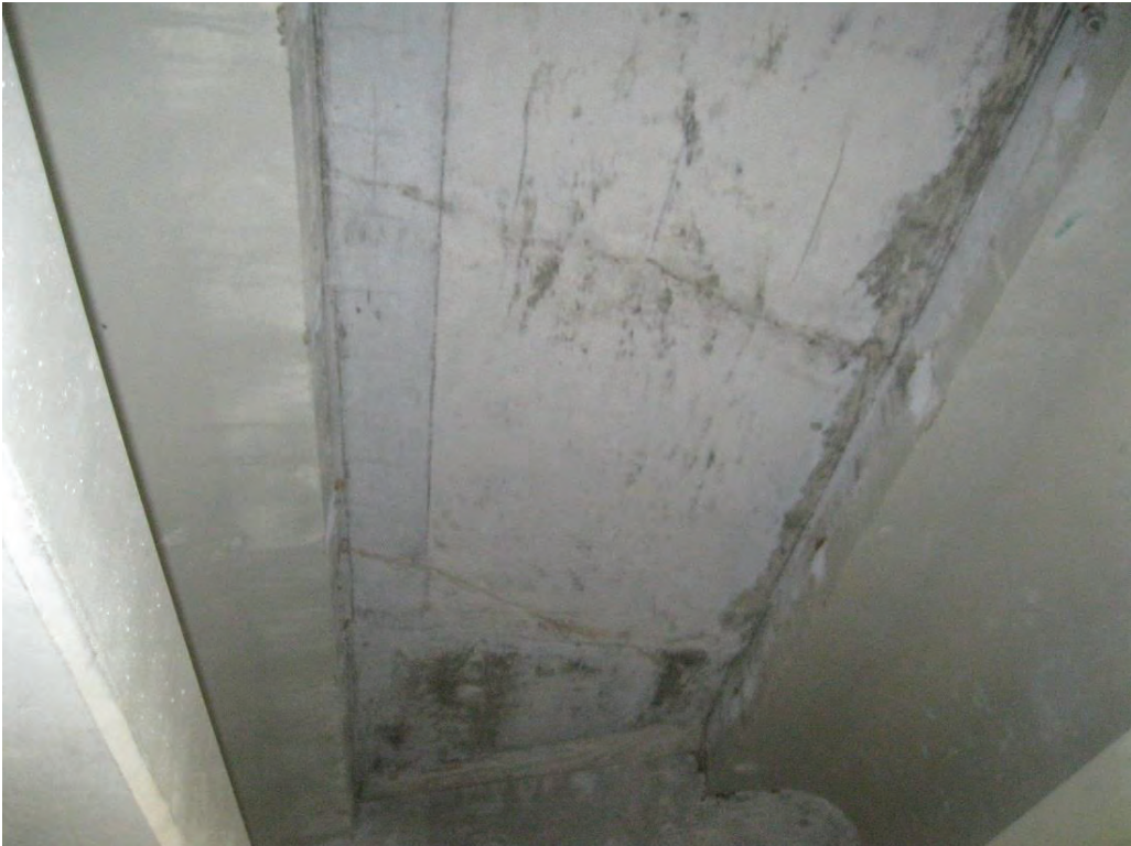
Figure 5-7 B-05-0604 Deck Underside Cracking
