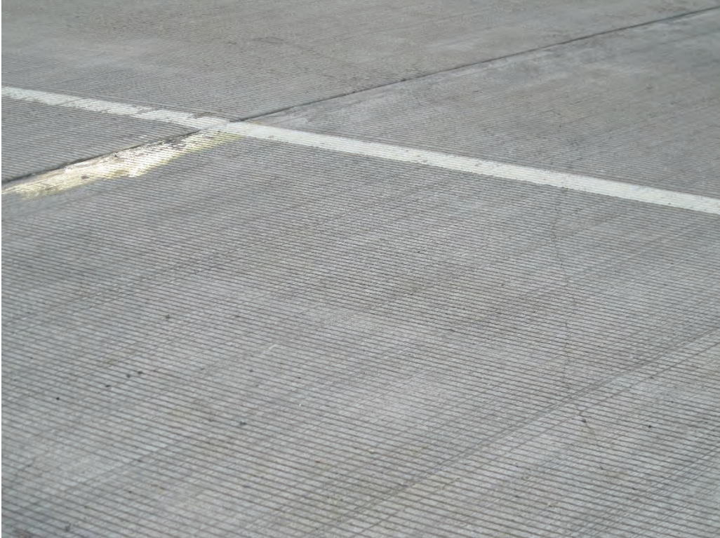
Figure 5-4 B-05-0604 Approach Apron Cracking
