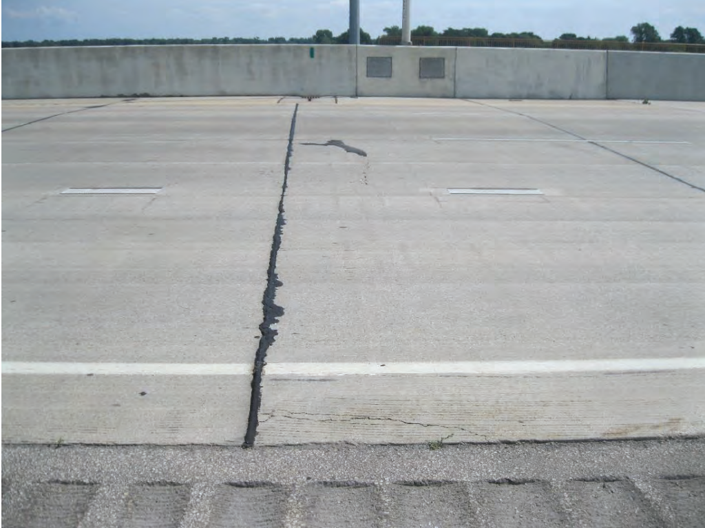
Figure 5-51 B-70-0264 Approach Patch and Cracking
