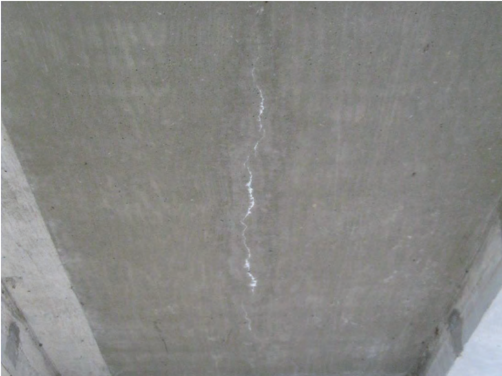
Figure 5-76 B-70-0268 Deck Cracking
