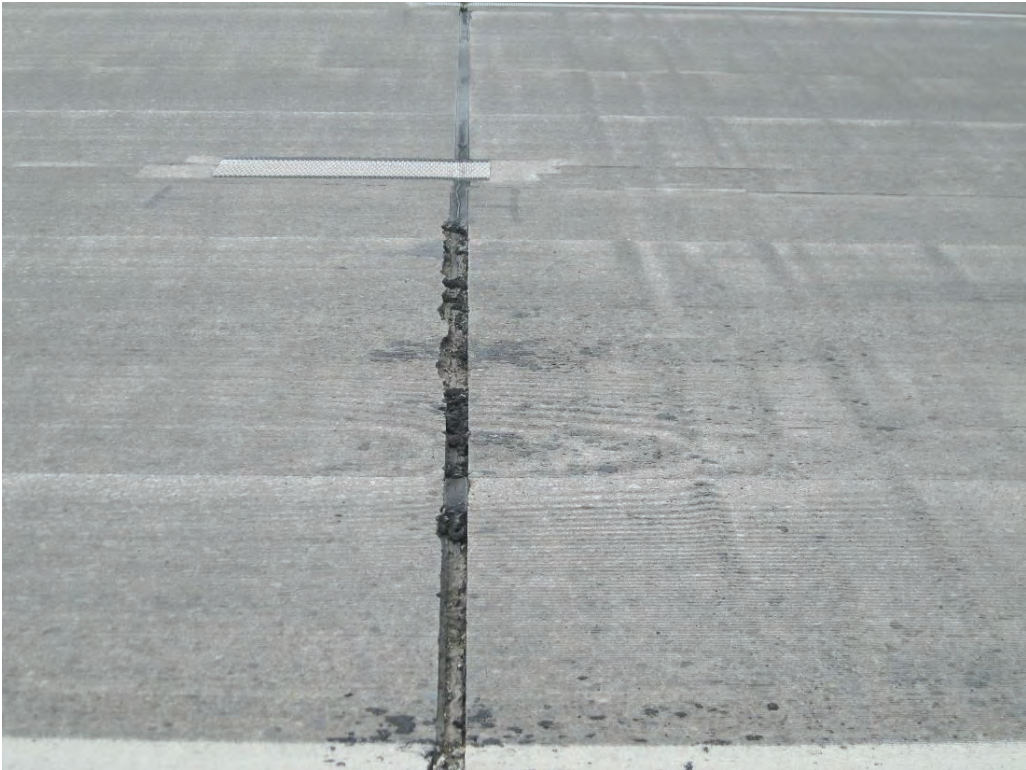
Figure 5-71 B-70-0267 Missing Joint Sealant
