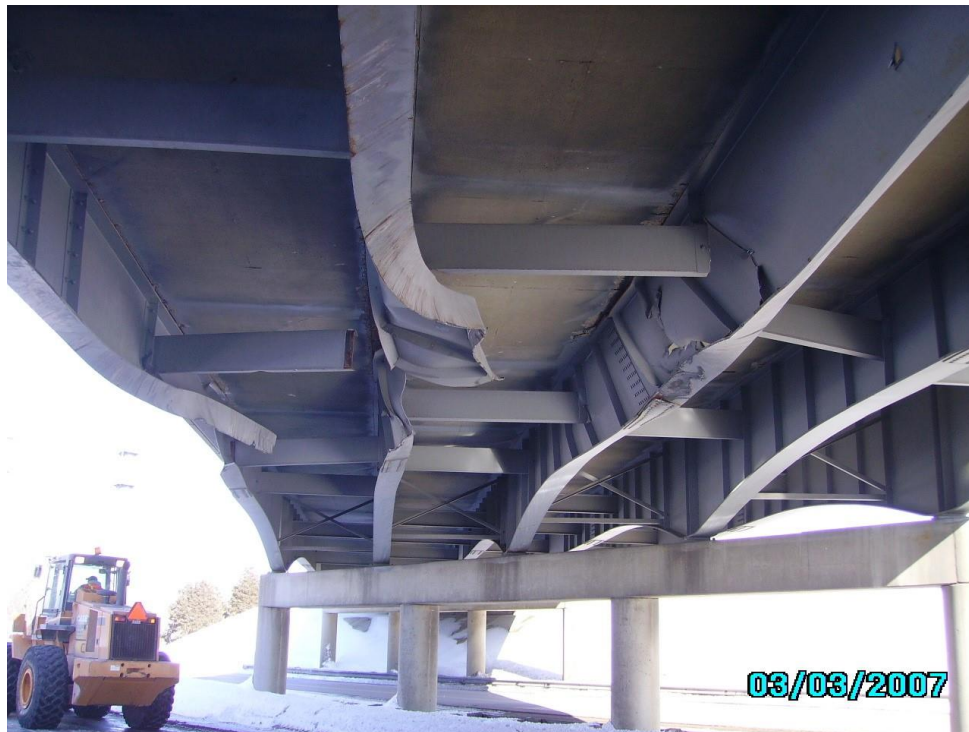
Figure 1.3.16.1-1: Critical Finding Photo
