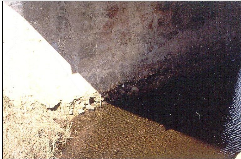
Figure 1.3.7.1-1: Local Scour at the Base of an Abutment.
