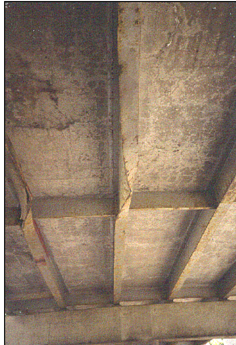
Figure 1.3.12.1-1: Impact Damage to a Steel Girder Bridge.
